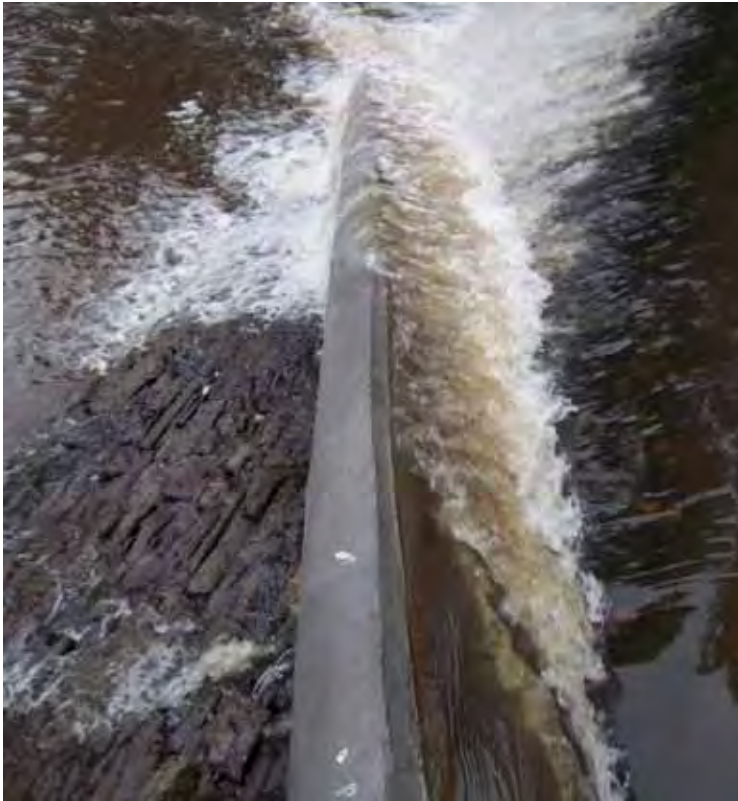
A baulk fish pass at Hunton on the River Arrow. This is one of several on the Arrow and a very cost effective way of restoring fish access on rivers with many weirs.
