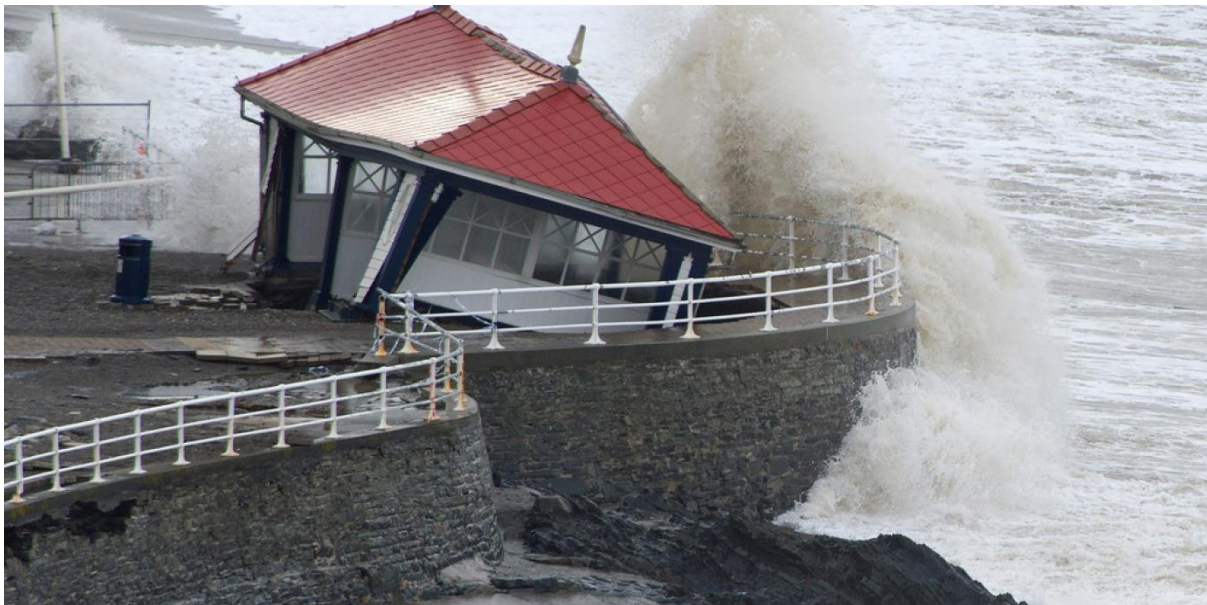
Figure 8: Coastal storm damage to Aberystwyth sea front, January 2014
