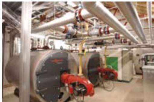
Gas fired boilers at the Stockethill development Reproduced with permission of Aberdeen City Council
