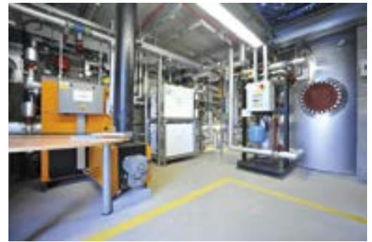
Energy centre at Greenwatt Way Reproduced with permission of SSE
