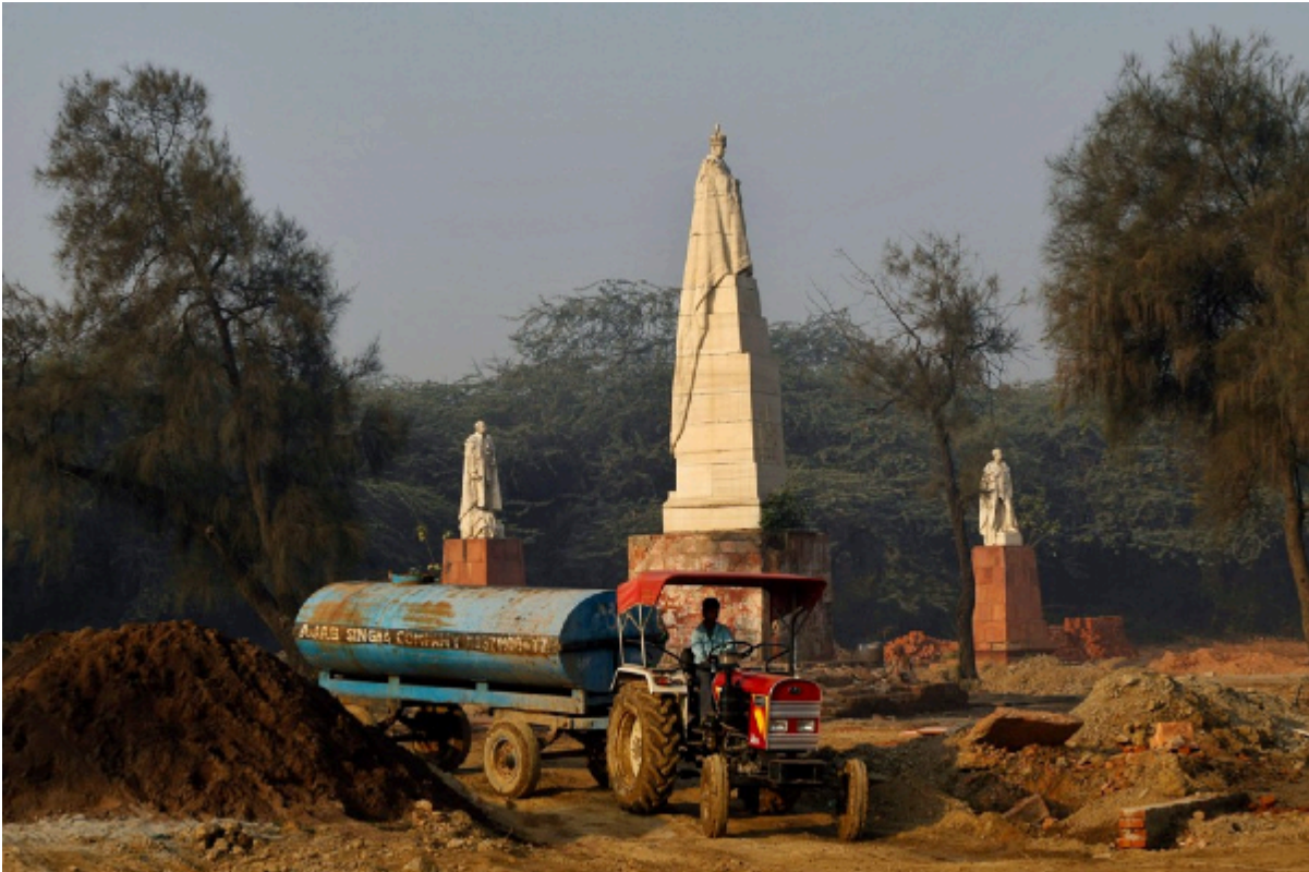
Statues of George V and two Viceroys during maintenance work at Coronation Park, Delhi.(Associated Press, Alamy).
