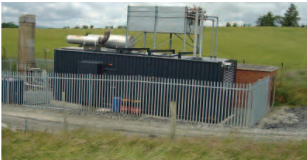
Figure 6: Generator utilising landfill gas
