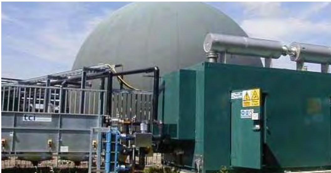
Figure 7: Combined heat and power generator utilising biogas at a sewage treatment works
