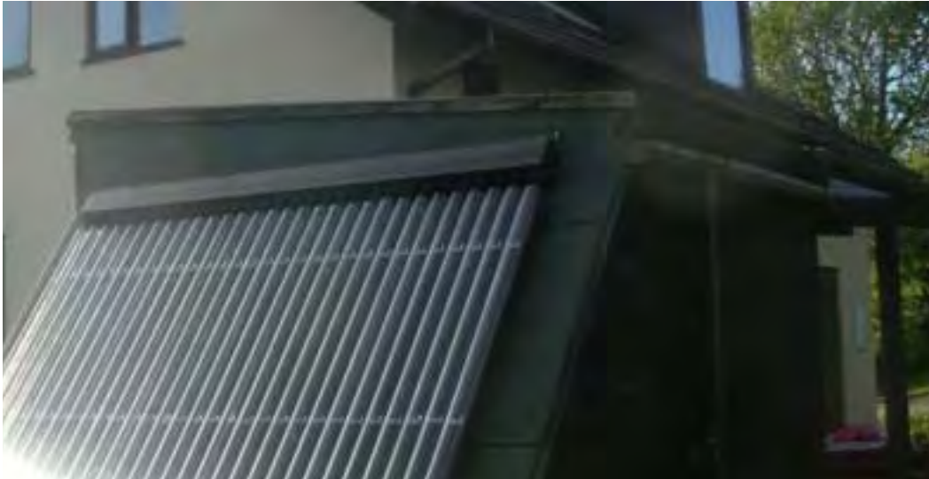
Figure 11: Evacuated tube collectors that have had to be sited other than on the roof in order to face south
