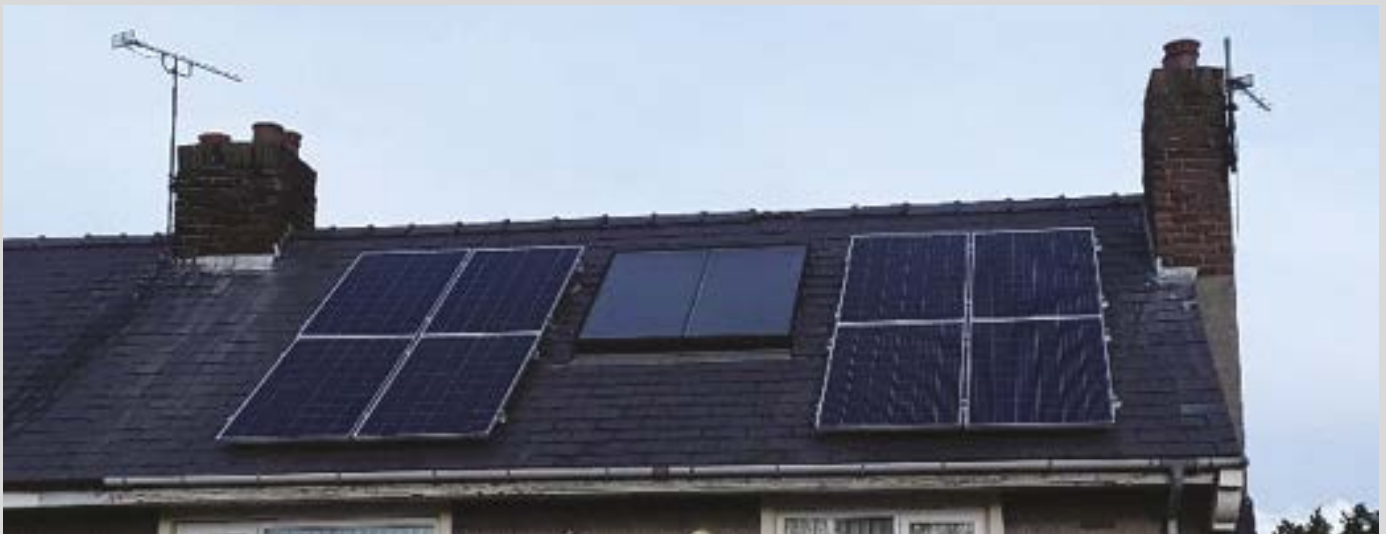
Solar panels installed through the Welsh Government's Arbed scheme
