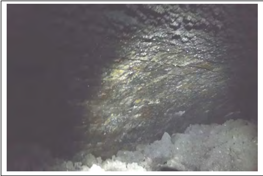
Photograph no 218: D/S haunch at 3122m Wet, otherwise good
