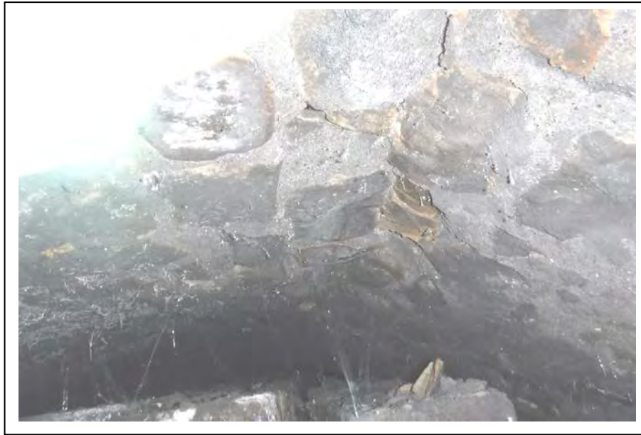
Photograph no C43: Arch flattened over Cwg ② Hinge pronounced in this area
