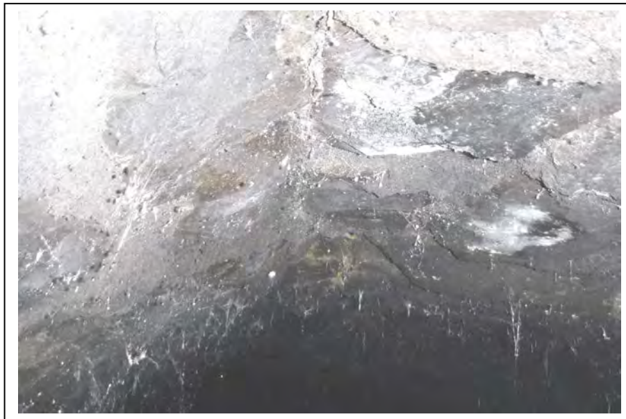
Photograph no C45: Hinge remains pronounce above LE of Cwg ③
