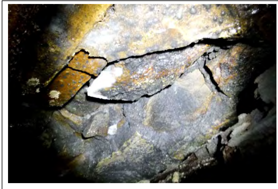
Photograph no 89: Crown at 857m (Ribs 43-44) Spalling 130 deep x 750 wide
