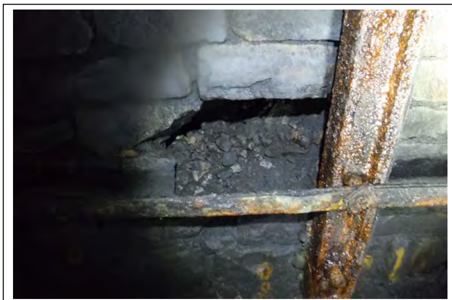
Photograph no 46: D/S sidewall at 190m (Ribs 122-123) Loss of section 375 high x 550 wide x 550 deep
