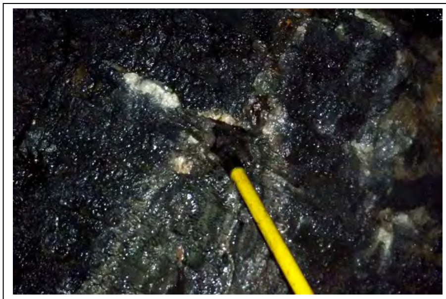
Photograph no 194: D/S haunch at 3069m Old timber packs to drainage line
