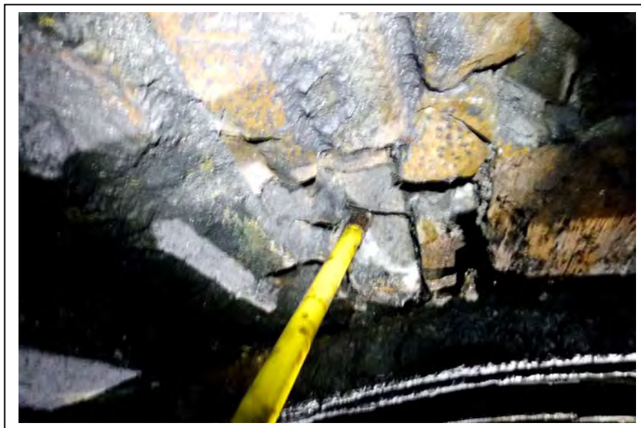
Photograph no 88: Crown at 857m (Ribs 43-44) Spalling 130 deep x 750 wide
