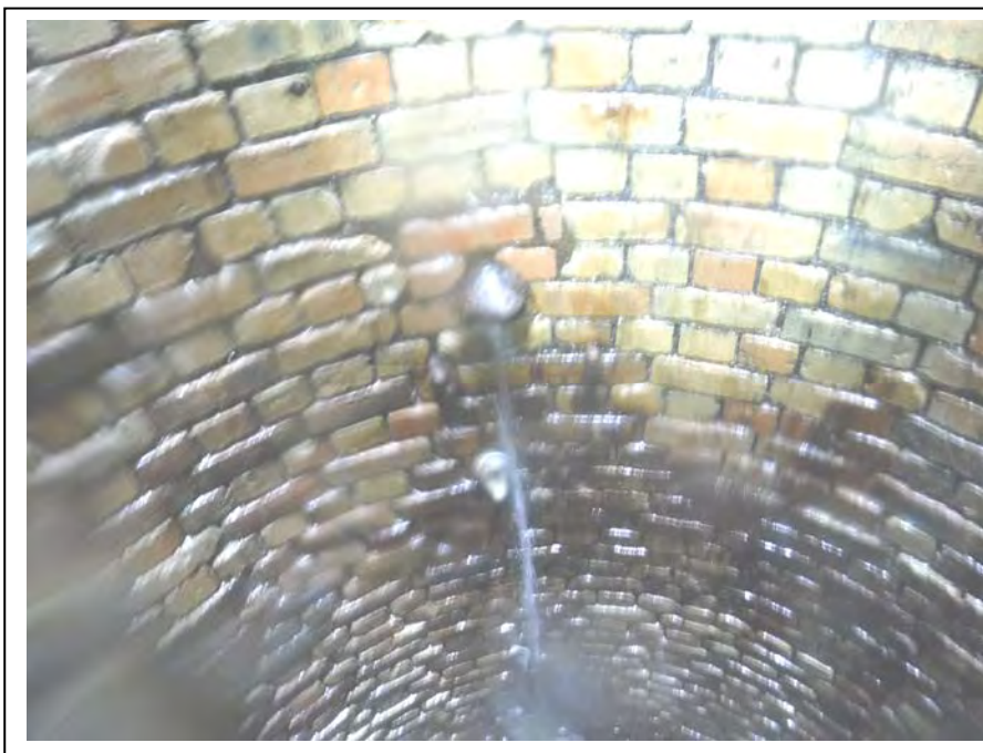
Photograph no 178: Water running from inlet at 8.5 – 10m Down-pipes missing below Brickwork very wet throughout below inlet level
