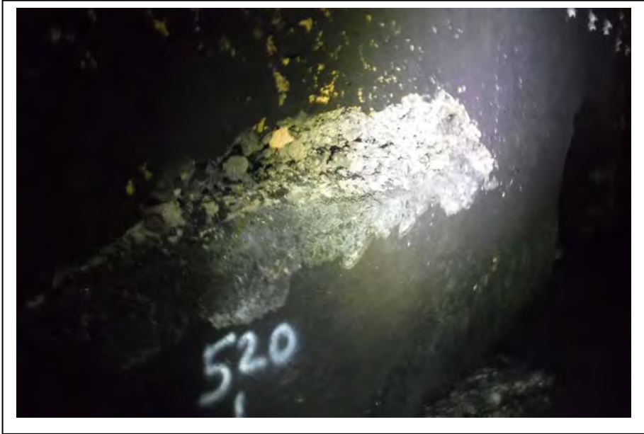
Photograph no 62: D/S sidewall at 520m Large section of loose concrete removed to sidewall Remainder hollow above for 5m 2
