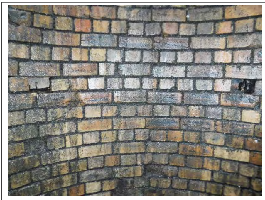
Photograph no 172: New slab level - 2m Brickwork to shaft is wet and dirty throughout Top section with open joints to 10
