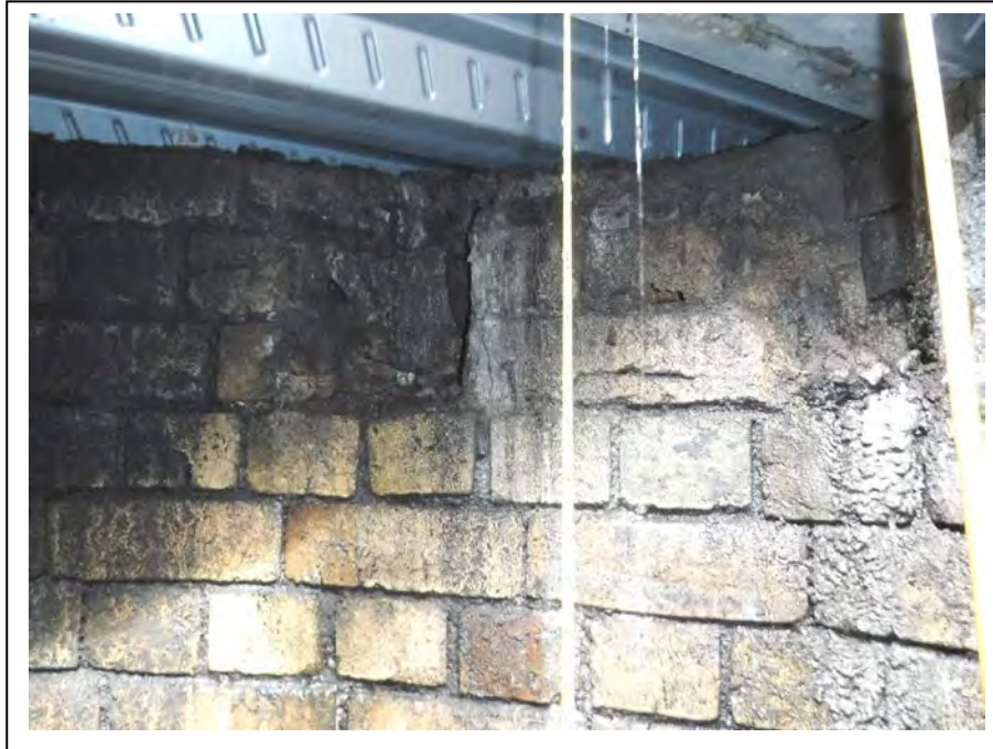
Photograph no 169: New slab level - 0.5m Widespread missing bricks to top 3no courses (below permanent metal formwork)
