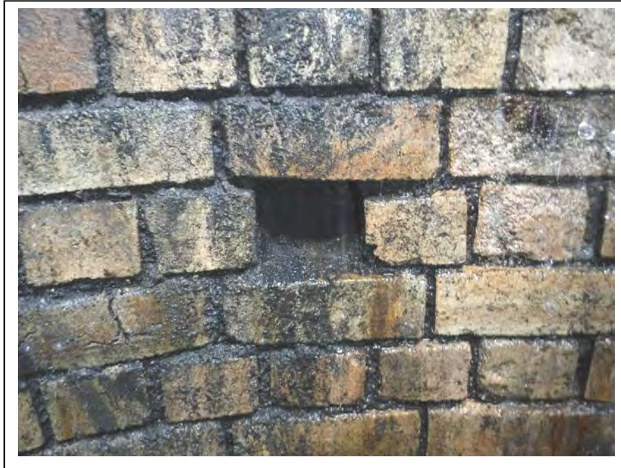
Photograph no 171: New slab level - 0.75m Bricks cut out for platform support during original construction (no timber remains) Typical throughout
