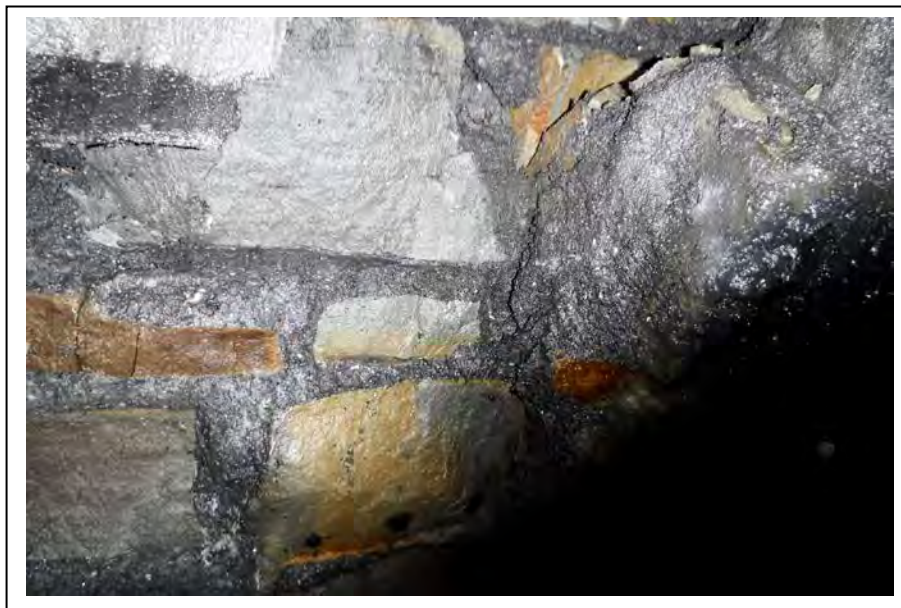
Photograph no 100: D/S haunch at 980m – 982m (Ribs 42-44) Loss of section 3m 2 to 230 max
