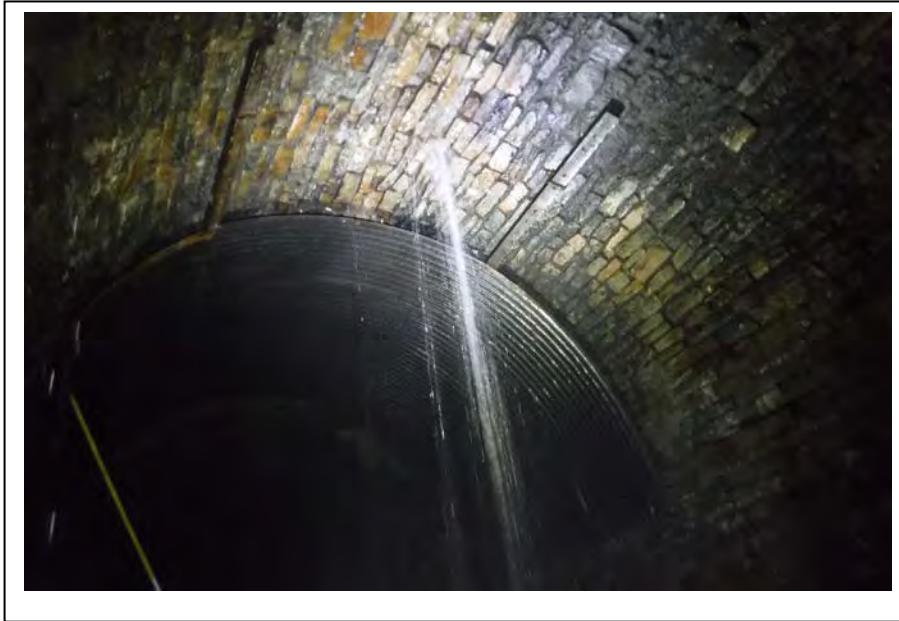
Photograph no 11: Crown at 56m Water running (full bore) Corrugated metal sheeting to rear
