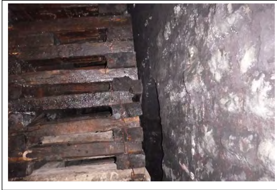
Photograph no C3: Cwg ① LE US sidewall
