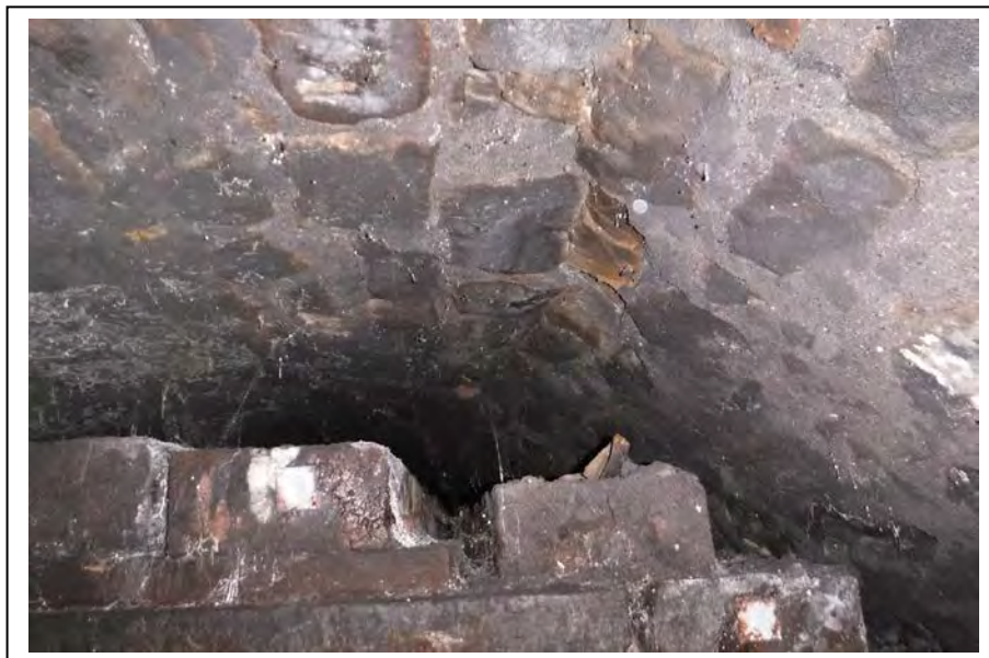
Photograph no C38: Arch flattened over Cwg ② Hinge pronounced in this area
