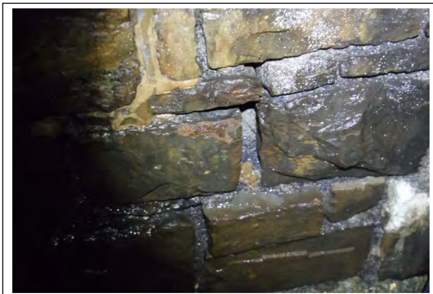
Photograph no 4: D/S sidewall at 5m Isolated joint loss 70mm to 200mm
