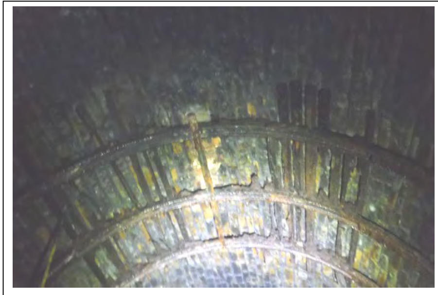
Photograph no 49: D/S haunch at 196m Water dripping
