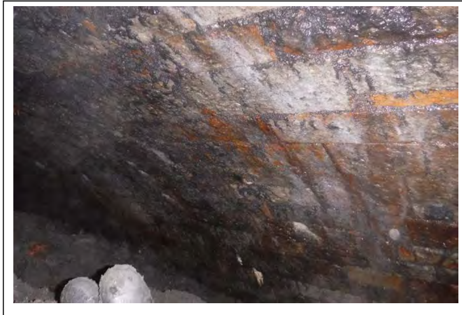
Photograph no 219: D/S haunch at 3122m Wet, otherwise good
