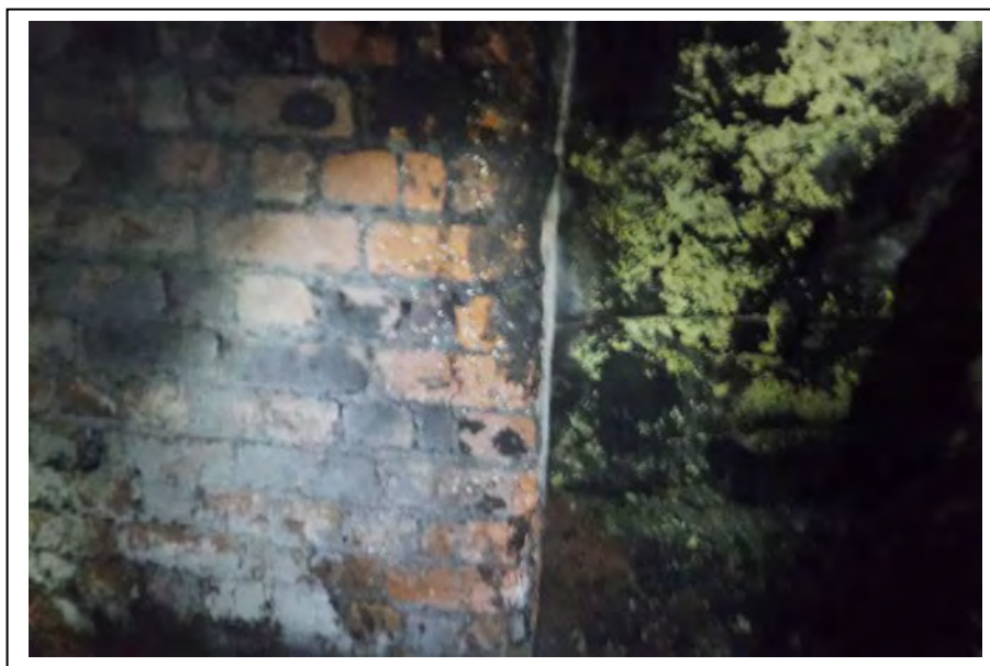
Photograph no 134: D/S sidewall at 1720m Spalling 30 to relieving arch pier quoin 1m long (Typical for several spans)
