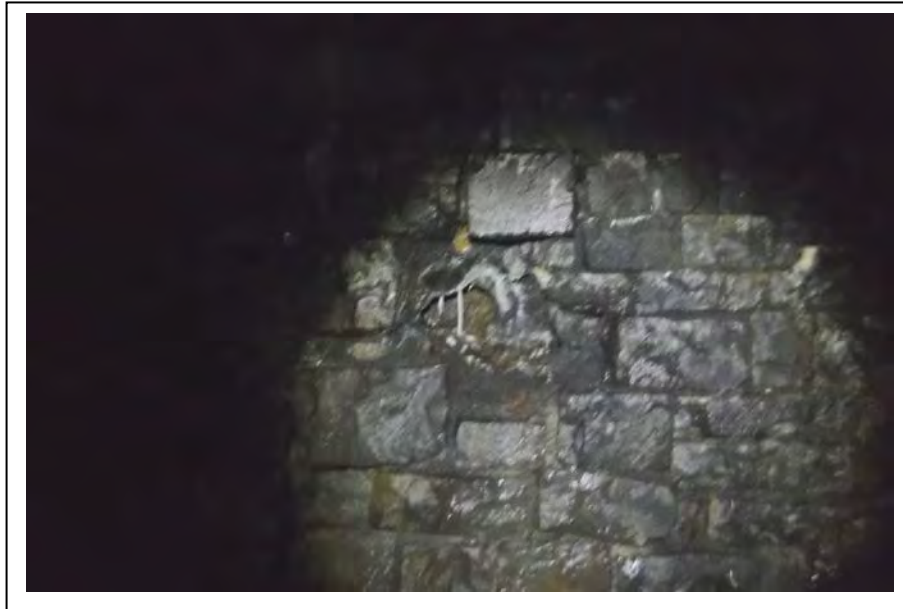
Photograph no 7: DS sidewall at 25m Loss of section 450 high x 550 wide x 750 deep
