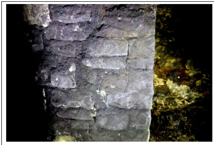
Photograph no 118: U/S refuge at 1050m CE quoin fractured on both faces 1.8m long open 5mm to sidewall
