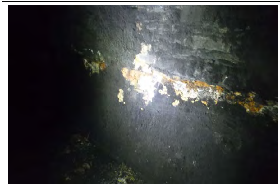
Photograph no 144: D/S sidewall at 2440m Soft concrete repair to surface slightly hollow to above 5m 2
