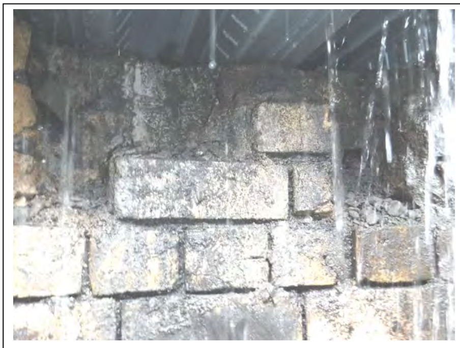
Photograph no 168: Shaft Widespread missing bricks to top 3no courses (below permanent metal formwork)
