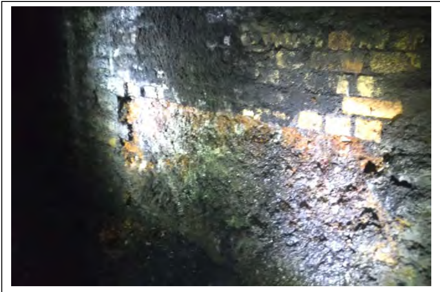
Photograph no 148: D/S sidewall at 2585m Failing brickwork repair 2000 wide x 850 high x 140 deep with 1m 2 hollow above
