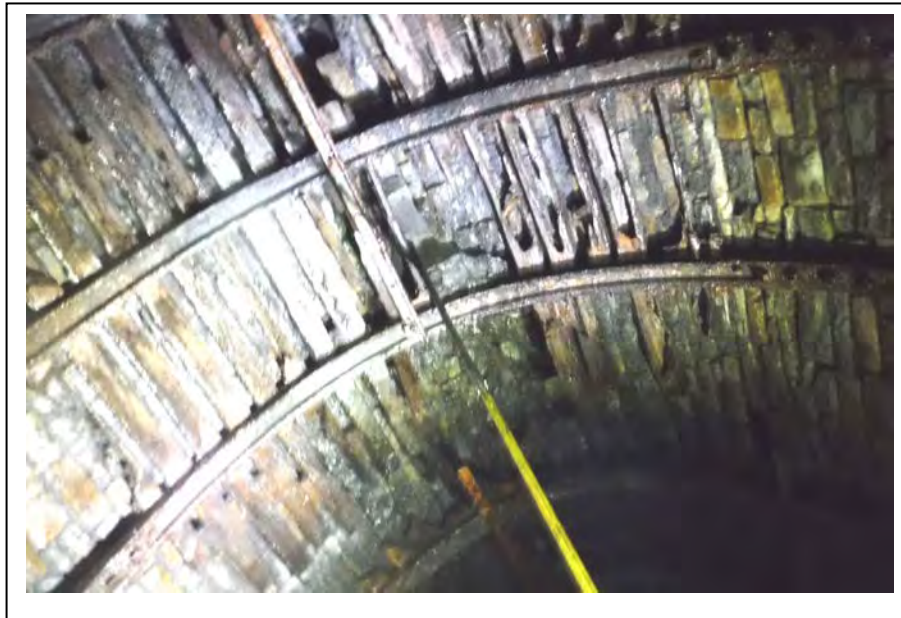
Photograph no 19: Crown at 94m (Ribs 19-20) Loss of section 600 wide x 340 deep max
