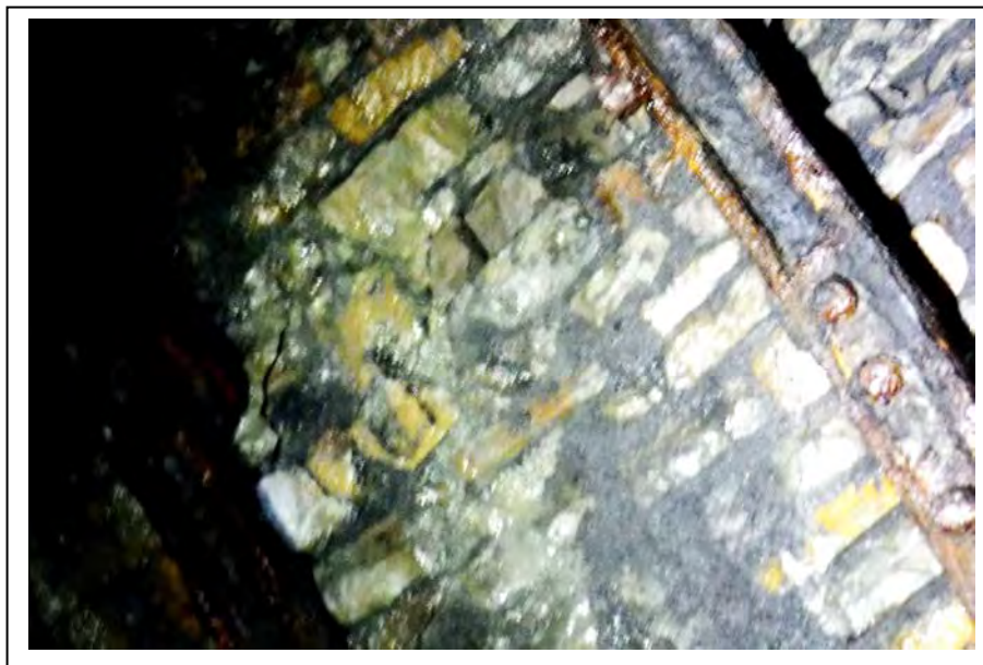
Photograph no 28: U/S haunch at 129m (Ribs 56-57) Spalling to 75 x 0.5m 2
