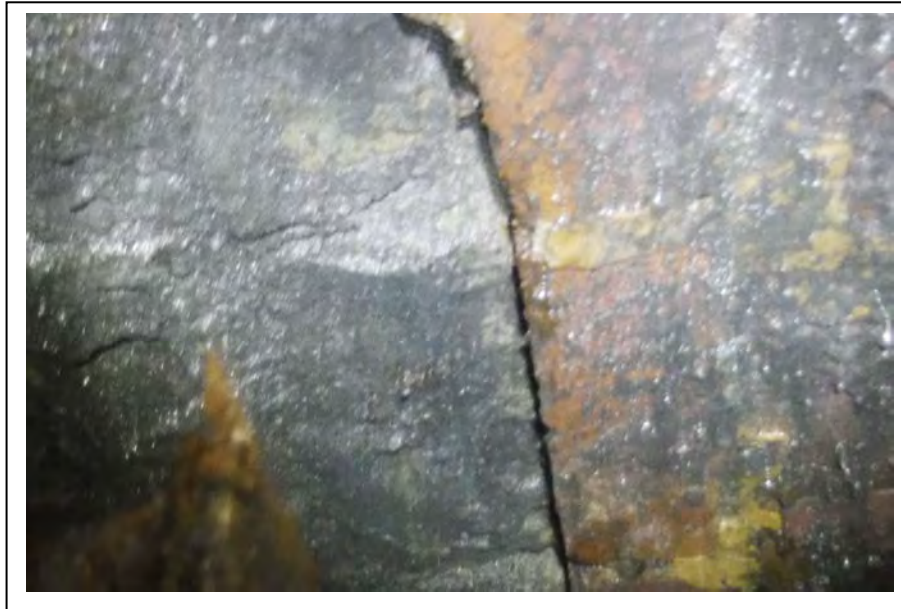
Photograph no 93: Crown at 864m – 866m (Ribs 54-56) Slight bulge/ discontinuity to repair
