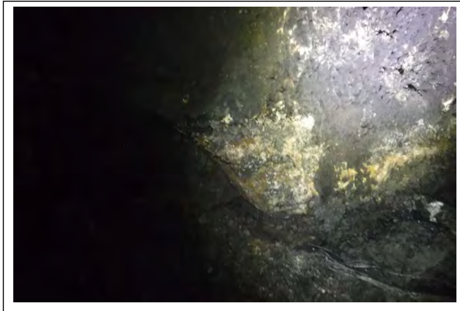
Photograph no 57: Relieving arches heavily spalled due to poorly compacted concrete (Typical view)
