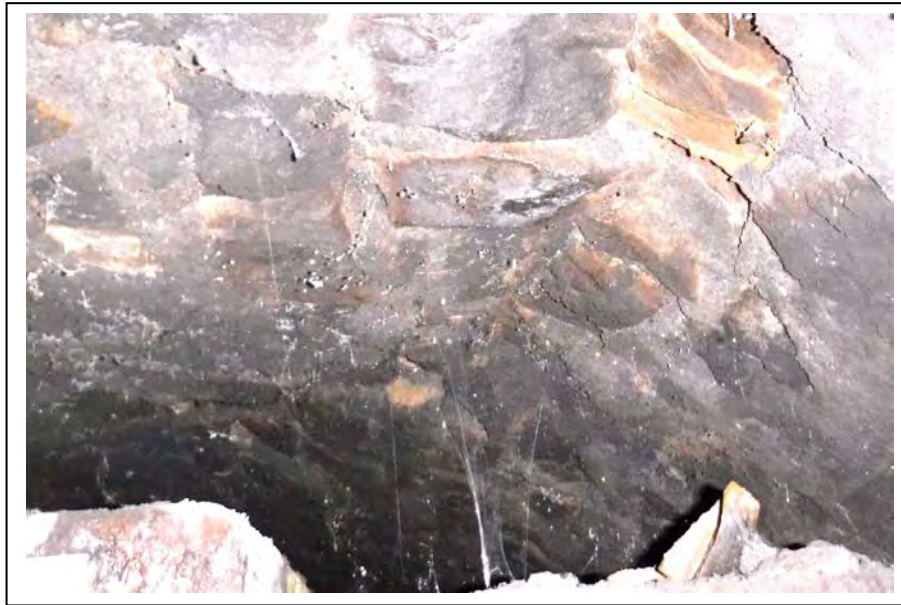
Photograph no C39: Arch flattened over Cwg No 2 Hinge pronounced in this area
