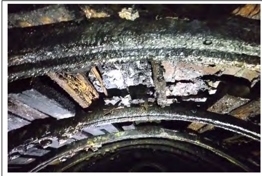
Photograph no 83: Crown at 854m (Ribs 40-41) Spalling 120 deep x 500 wide
