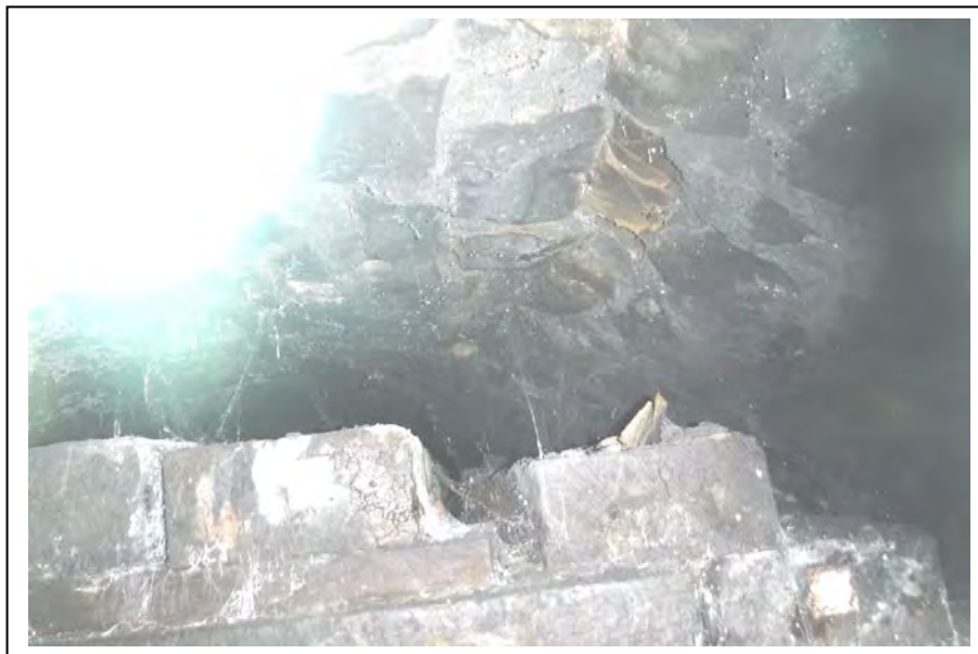
Photograph no C42: Arch flattened over Cwg ② Hinge pronounced in this area
