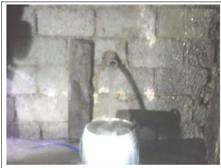
Photograph no 166: Water flowing from blocked section of tunnel behind diaphragm wall
