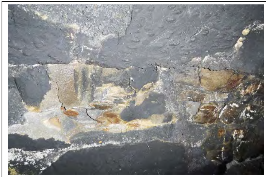
Photograph no C27: Crown at 1950m Spalling along hinge line to 50 deep
