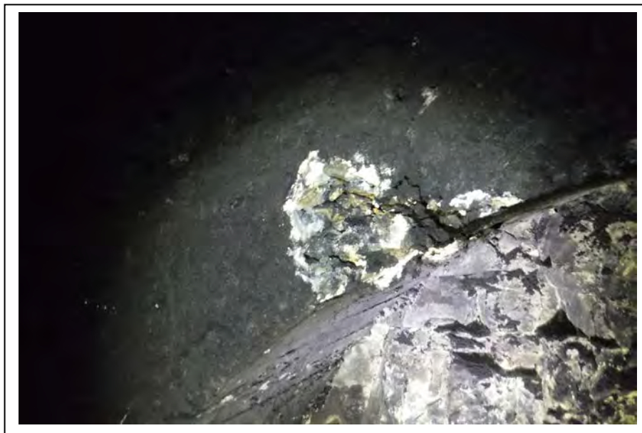
Photograph no 124: D/S at 1225m Spalling 90 x 0.1m 2 to relieving arch
