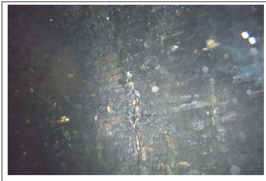
Photograph no 202: Soft material (timber) noted to haunches at sites of previous down-pipe fixings (typical)
