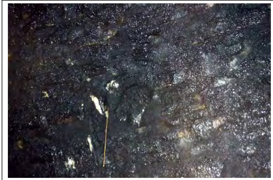
Photograph no 193: D/S haunch at 3061m Old timber packs to drainage line
