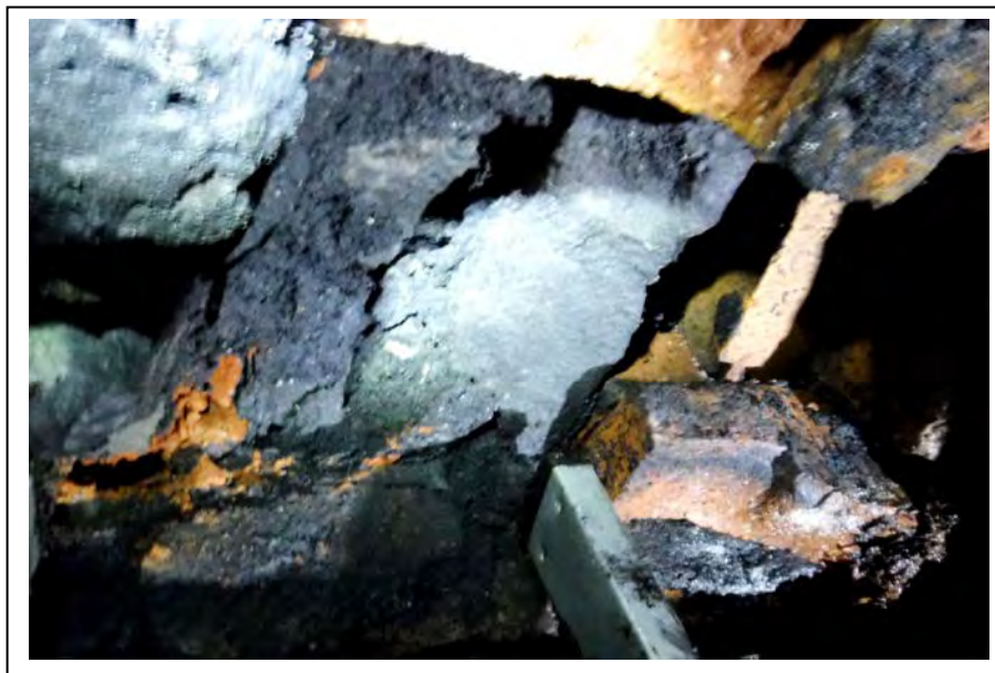
Photograph no 102: U/S upper haunch at 982m (Ribs 44-45) Loss of section 0.5m 2 x 180 deep max
