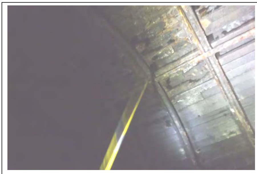
Photograph no 104: Minor spalling to D/S haunch at 1000m
