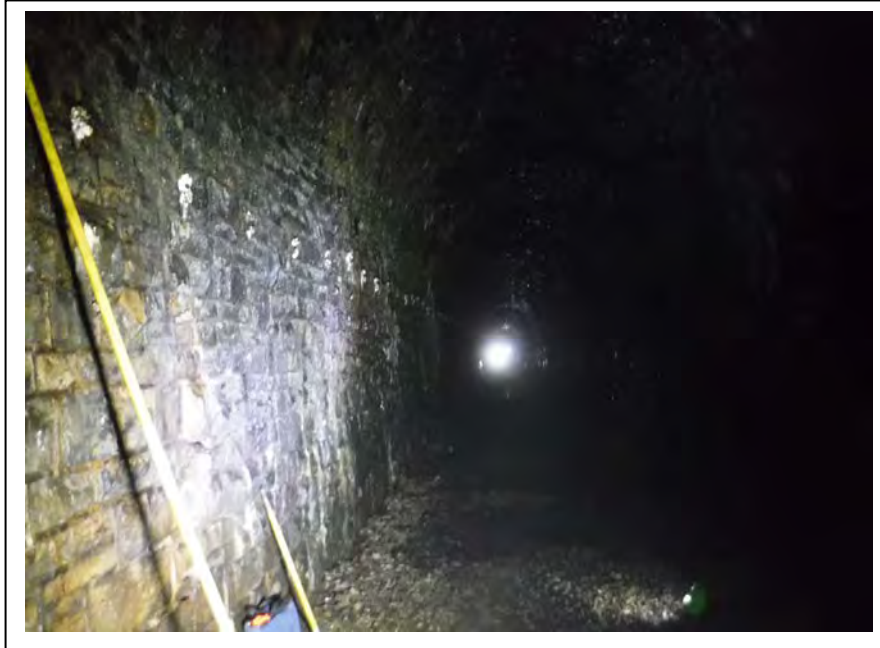
Photograph no 3: Water running at 5m D/S sidewall
