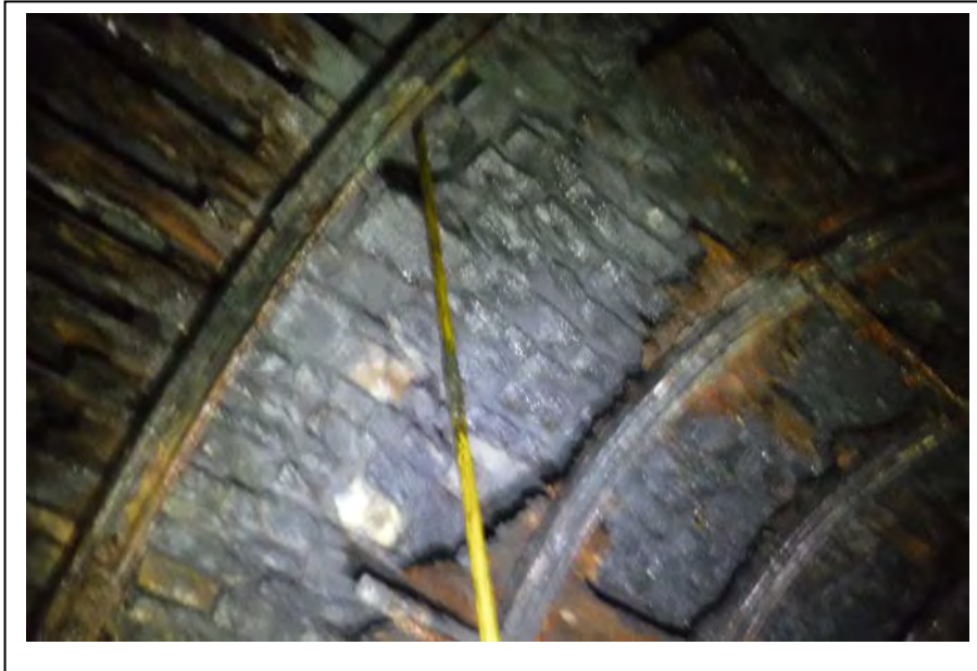
Photograph no 23: Crown at 112m Deep loss of section to DS crown 350 deep
