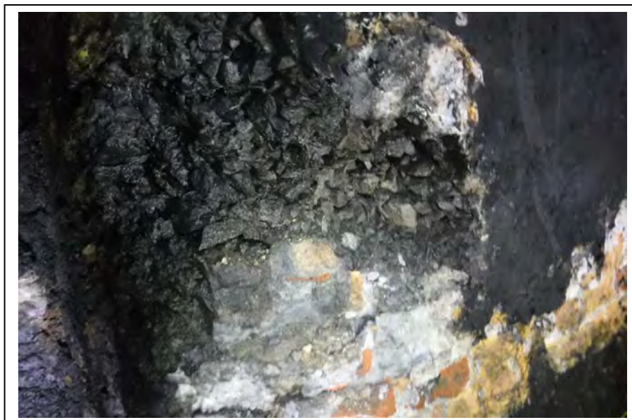
Photograph no 142: U/S refuge at 2430m Spalling to quoin and sidewall 250 deep x 1000 high x 580 wide
