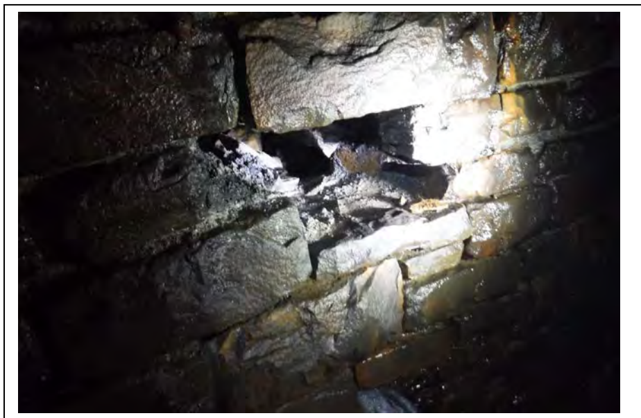
Photograph no 12: D/S sidewall at 52m Loss of section 800 high x 450 wide x 250 deep
