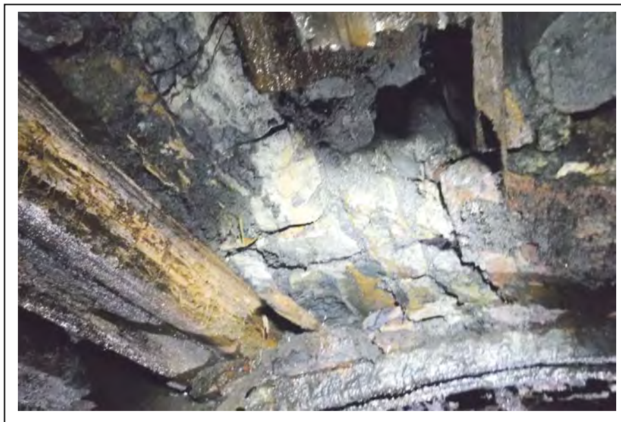
Photograph no 82: Crown at 854m (Ribs 40-41) Spalling 250 deep x 1m wide
