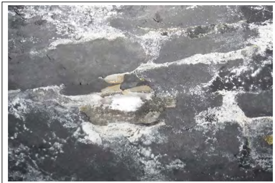
Photograph no C24: Hinge at CE of Cwg1 at 1948m
