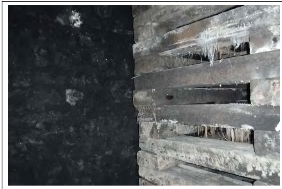
Photograph no C16: Cwg ③ LE DS sidewall
