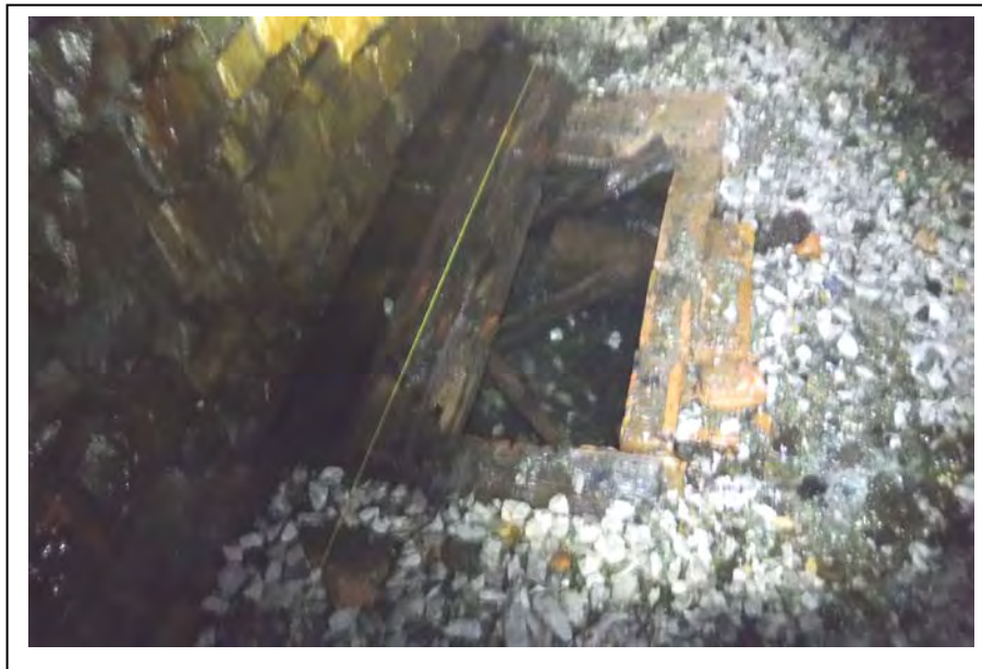
Photograph no 54: U/S sidewall at 230m Drainage full low flow
