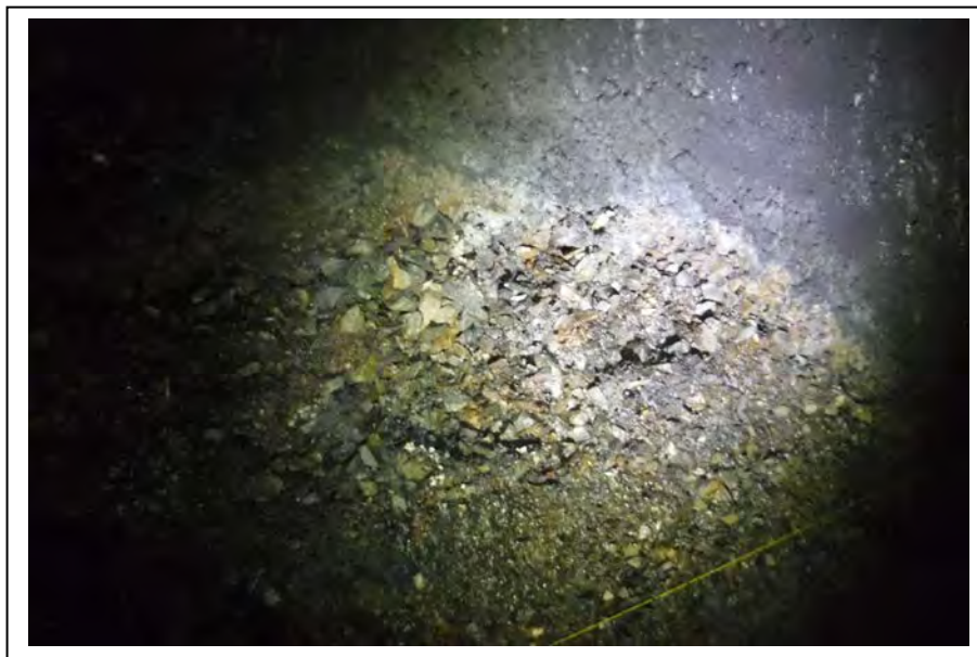
Photograph no 56: Relieving arches heavily spalled due to poorly compacted concrete (Typical view)
