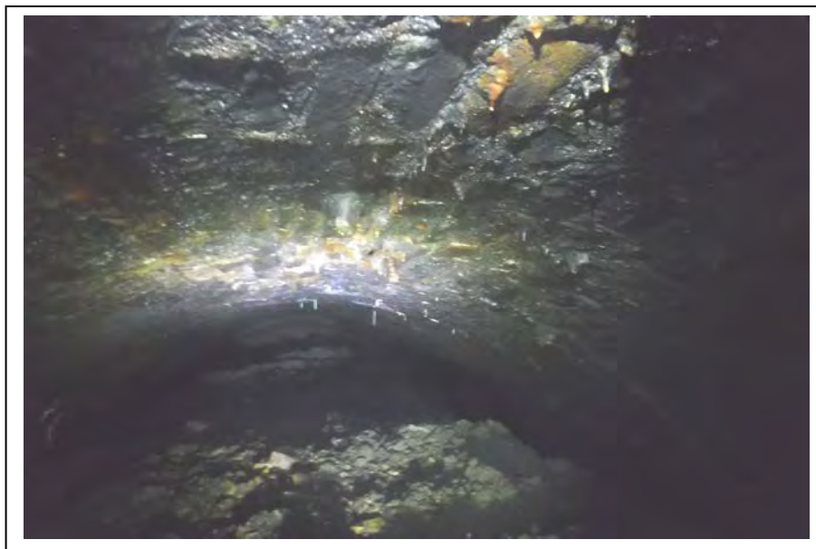
Photograph no 210: Crown to D/s haunch at 3018m Area of visible flattening of barrel form Firm to hammer
