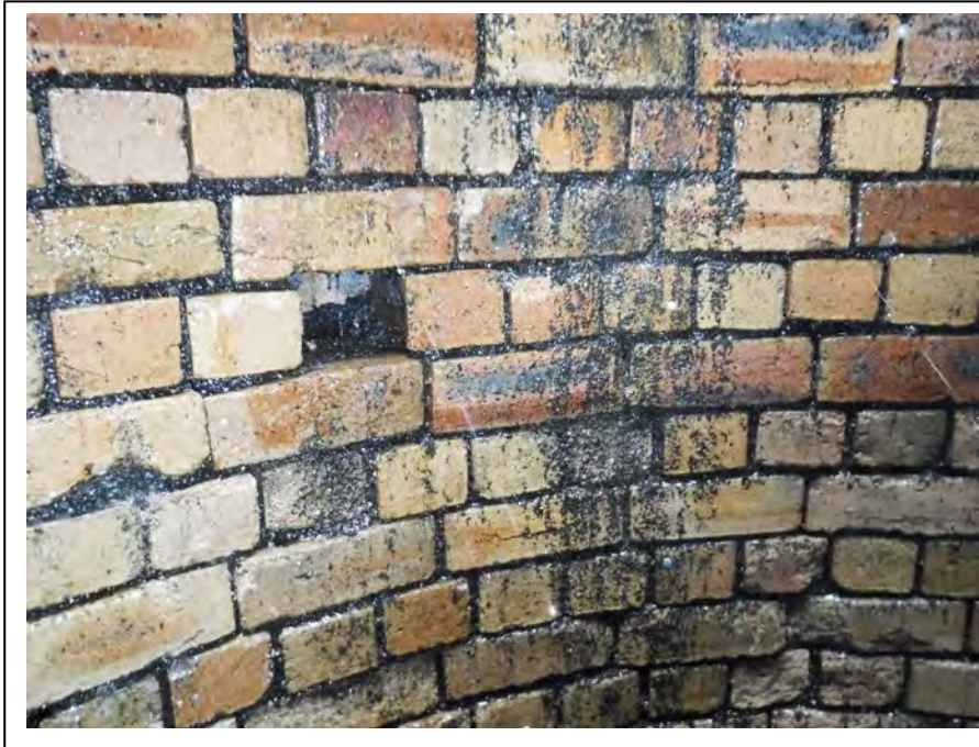
Photograph no 173: New slab level - 2.25m Bricks cut out for platform support during original construction Lower shown
