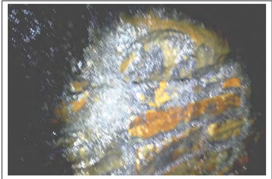
Photograph no 149: U/S sidewall 2600m – 2665m Widespread areas of soft mortar to sidewalls (where wet) Underlying concrete sound
