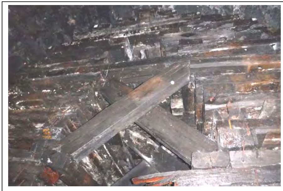
Photograph no C6: Cwg ① CE crown
