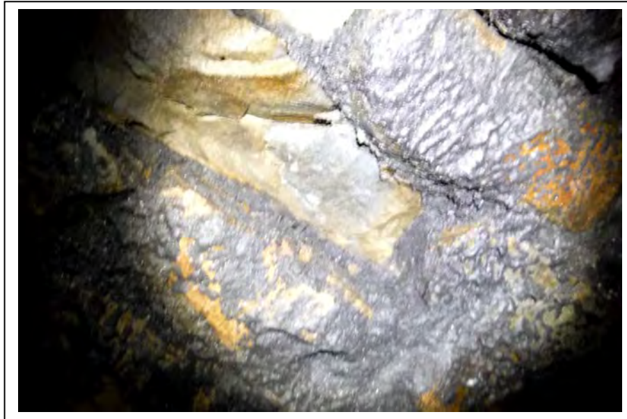
Photograph no 87: Crown at 856m (Ribs 42-43) Spalling 130 deep x 400 wide
