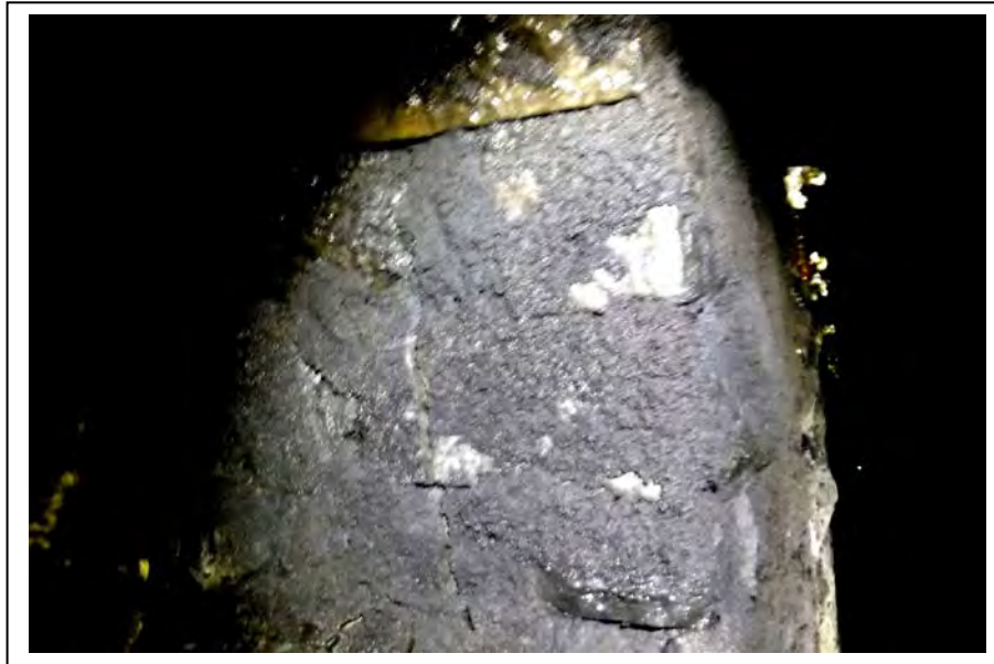
Photograph no 117: D/S refuge at 1040m Intrados is also fractured to 10mm
