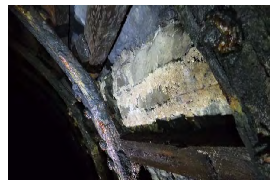
Photograph no 32: DS haunch at 148m (Ribs 79-80) Repair to haunch separation in rough concrete
