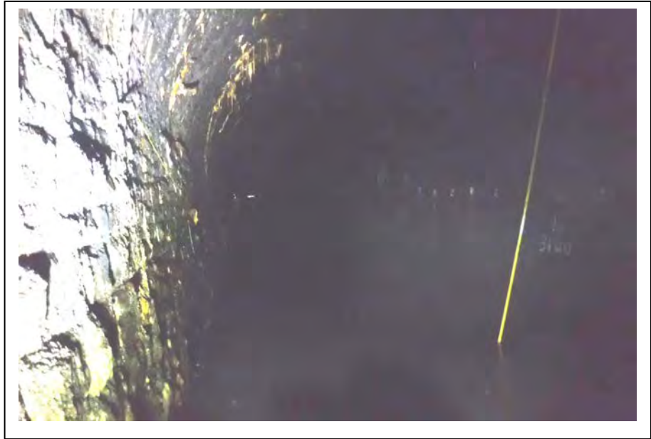
Photograph no 221: The whole area between diaphragm wall at 3044m and backfill is flooded to 450mm max
