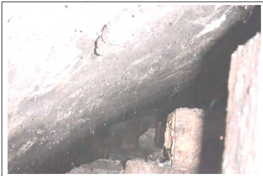
Photograph no C30: No evidence of packing to haunches of Cwg gap is typical of all elements, similar to crown
