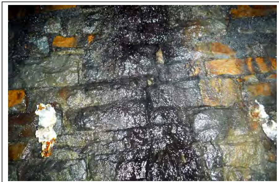
Photograph no 198: D/S sidewall at 3074m Odd open joints 120 deep along old drainage line
