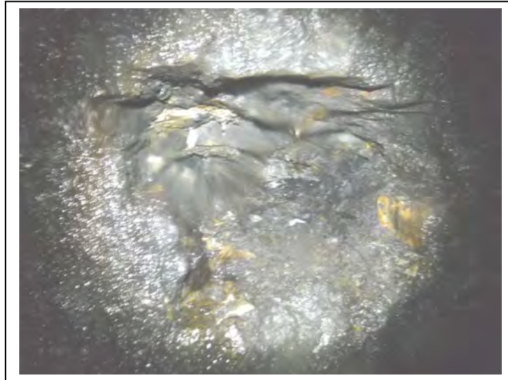
Photograph no 157: U/S sidewall at 3005m Loss of section 600 wide x 400 high x 850 deep
