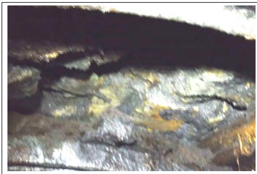
Photograph no 84: D/S crown at 853m (Ribs 39-0) Spalling to 250 deep x 1.1m wide
