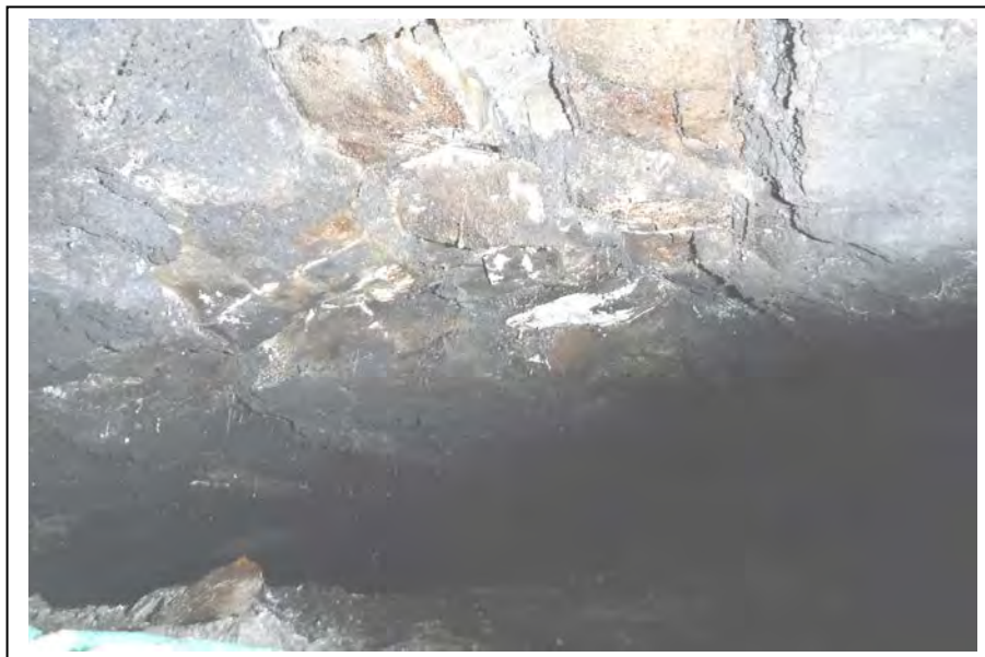
Photograph no C28: DS haunch at 1950m Hinge becomes more severe over Cwg 2
