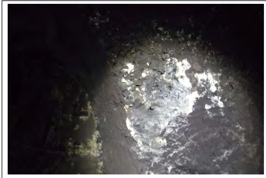
Photograph no 123: U/S at 1220m Spalling 90 x 0.1m 2 to relieving arch
