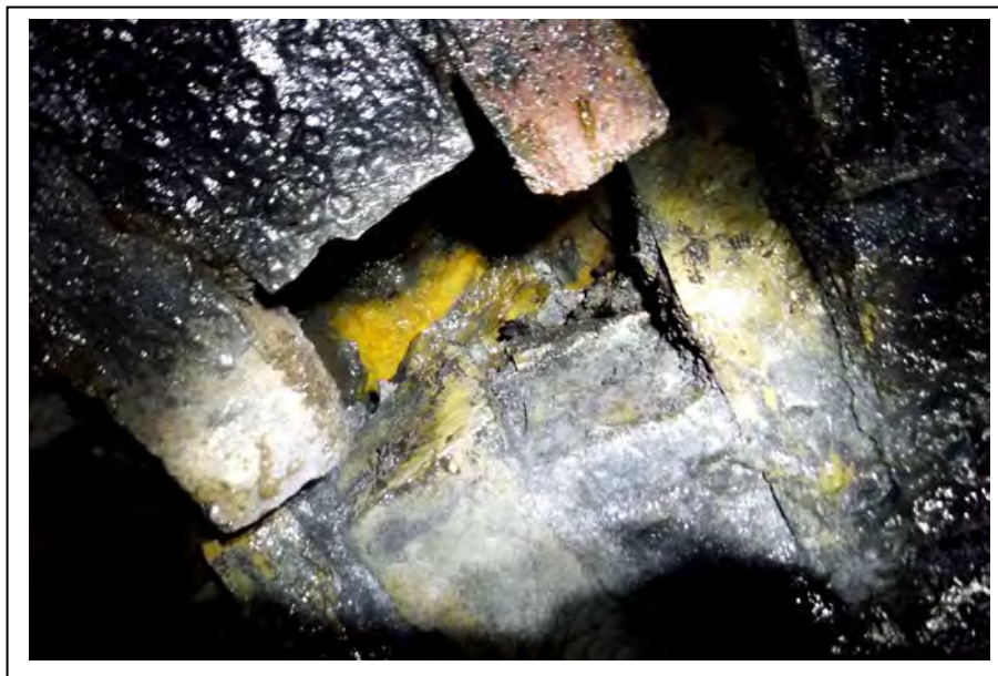
Photograph no 96: Crown at 866m (Ribs 56-57) Void > 1500 deep
