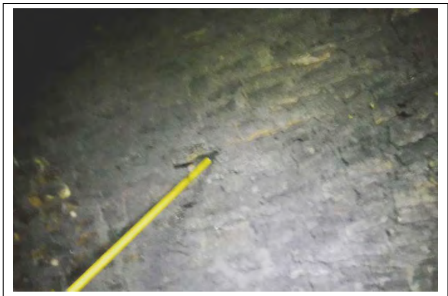
Photograph no 150: D/S haunch at 2725m Isolated linear loss of section to 60mm
