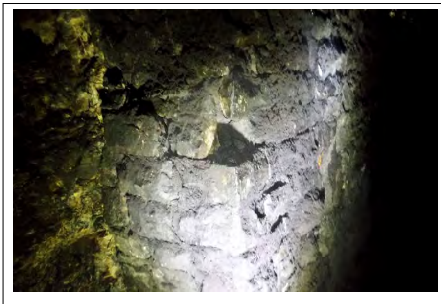
Photograph no 114:D/S refuge at 1040m: Missing stone to D/S quoin
