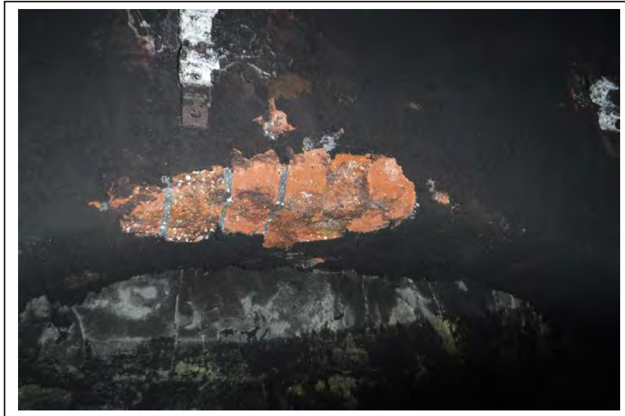
Photograph no 129: D/S relieving arch at 1385m Spalling 50 x 0.1m 2 to soffit
