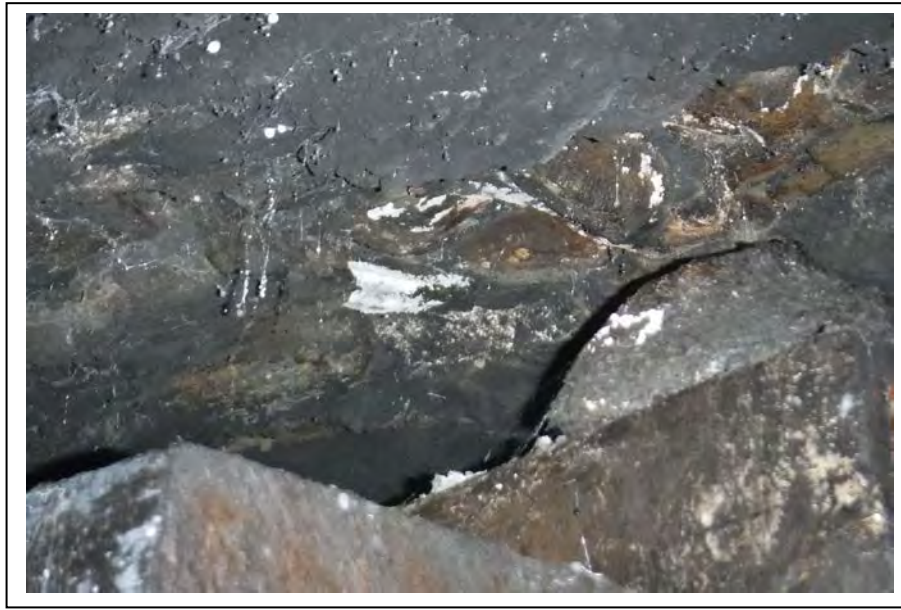
Photograph no C31: Secondary hinge at DS haunch at 1951m
