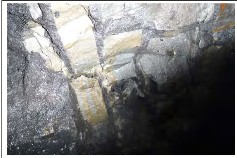
Photograph no 99: Crown at 981m (Ribs 42-43) Loss of section 1m 2 to 230 max
