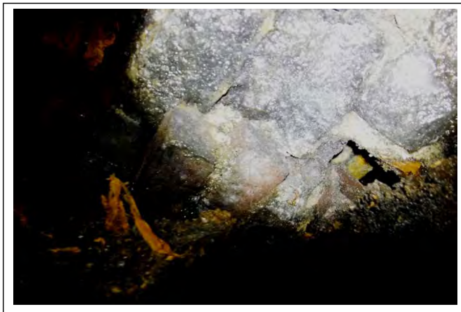
Photograph no 94: D/S haunch at 866m (Ribs 56-57) Displaced brick work to 100 max
