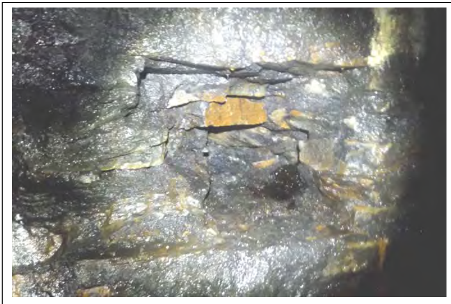
Photograph no 156: D/S sidewall at 3015m Loss of section 750 wide x 450 high x 725 deep
