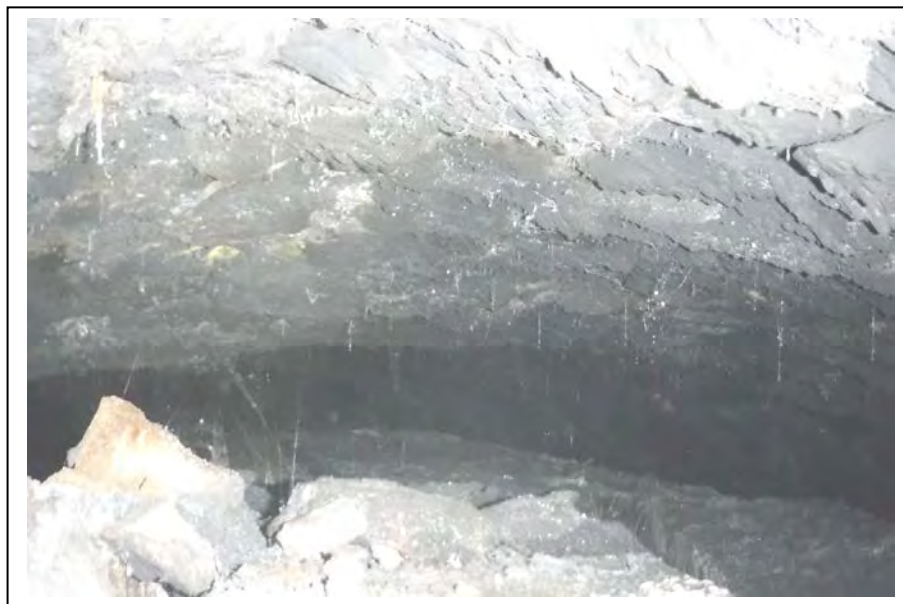
Photograph no C34: Flattening of arch at 1951m is typical
