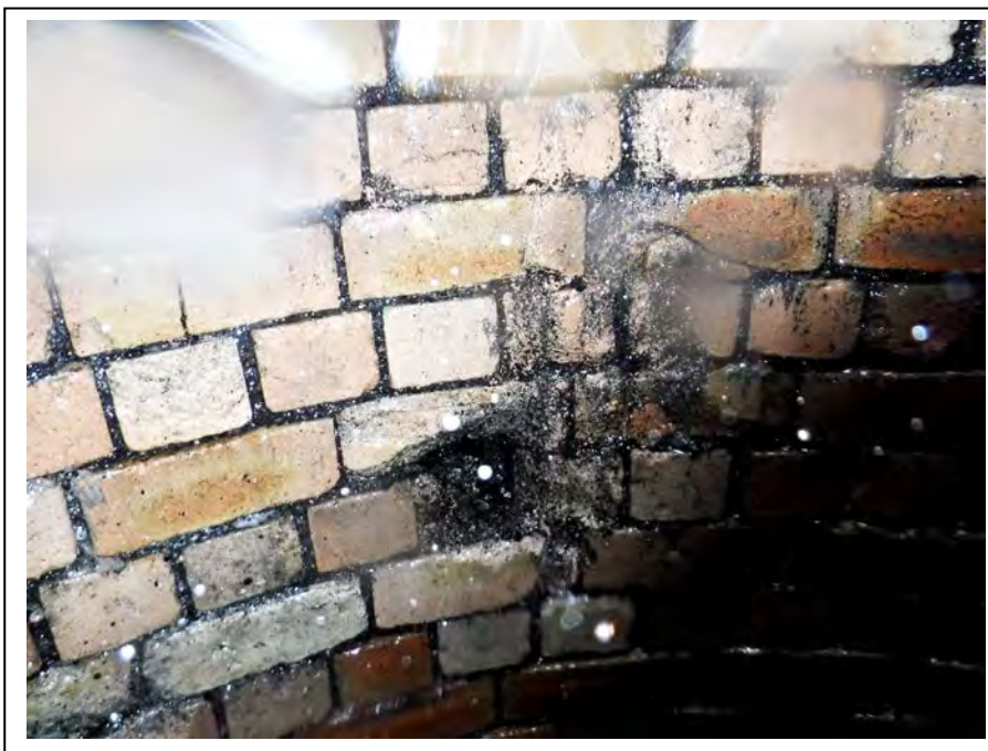
Photograph no 176: New slab level at 4.75m Single brick spalled to 15
