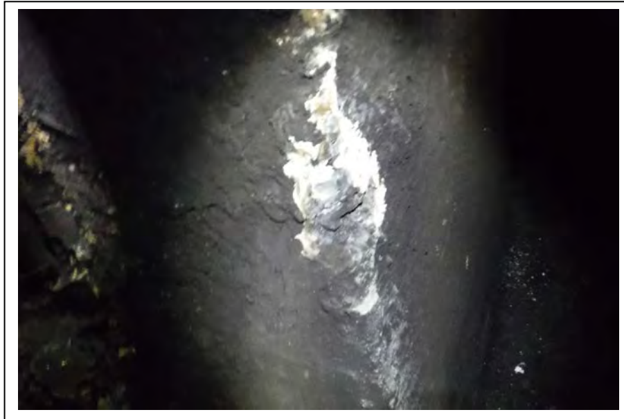
Photograph no 121: Relieving arches to D/S sidewall between 1160m and 1232m are in good condition However, the pier quoins have widespread areas of loose rough concrete (poorly compacted) Larger defects are noted individually
