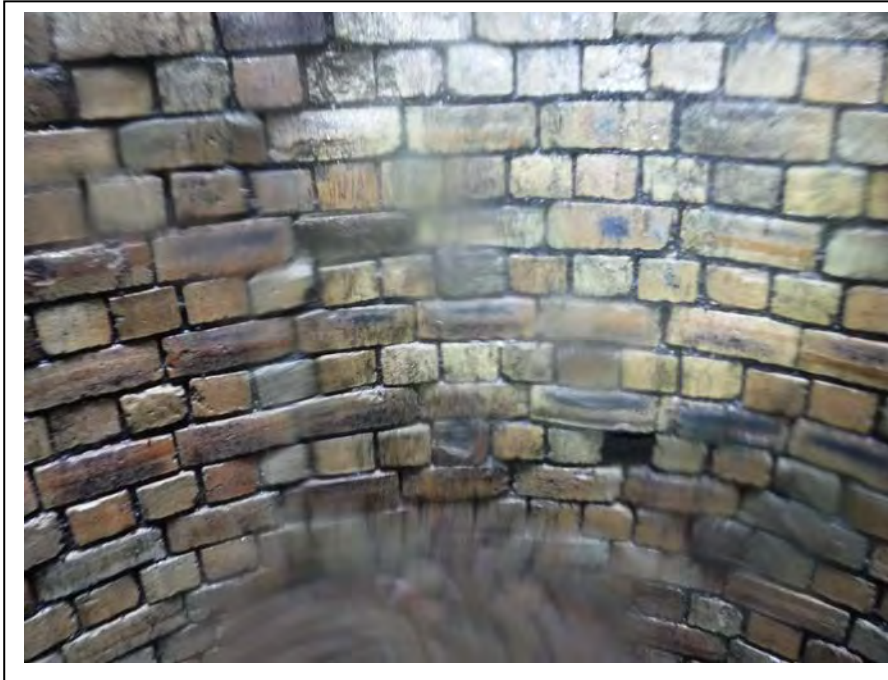
Photograph no 177: Measured from new shaft slab level - 10.0m Cut outs and irregular facework typical throughout Example shown at 5.5m
