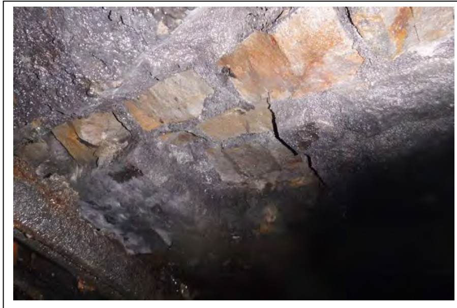
Photograph no 101: D/S haunch at 980m – 982m (Ribs 42-44) Loss of section 3m 2 to 230 max
