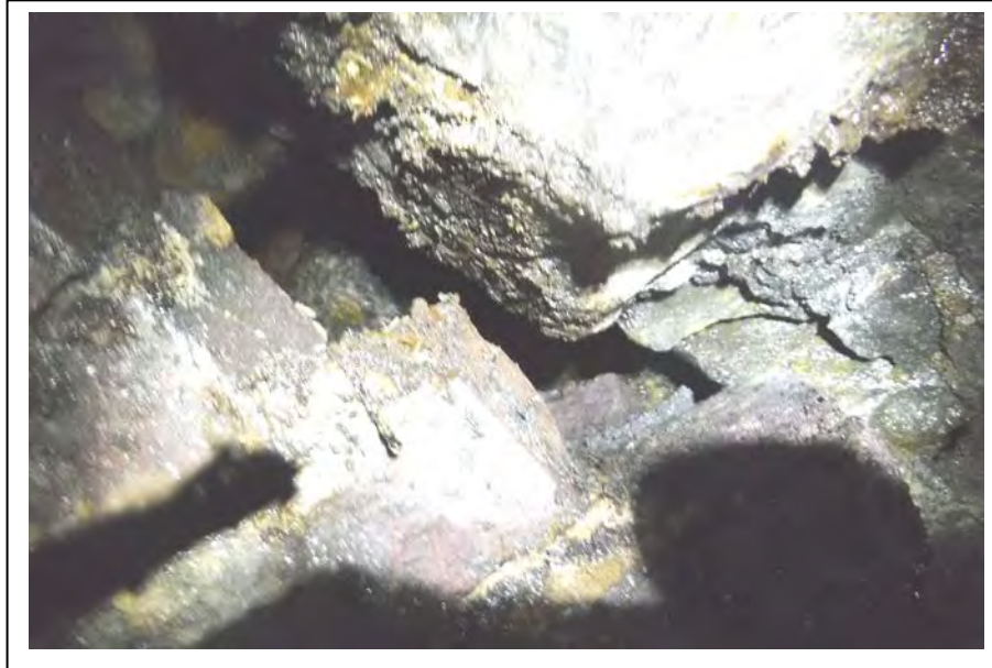
Photograph no 95: D/S haunch at 866m (Ribs 56-57) Void > 800 deep
