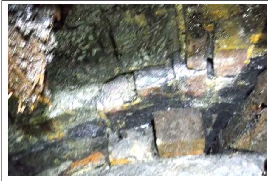
Photograph no 91: Crown at 863m (Ribs 53-54) Displacement of section to brick repair
