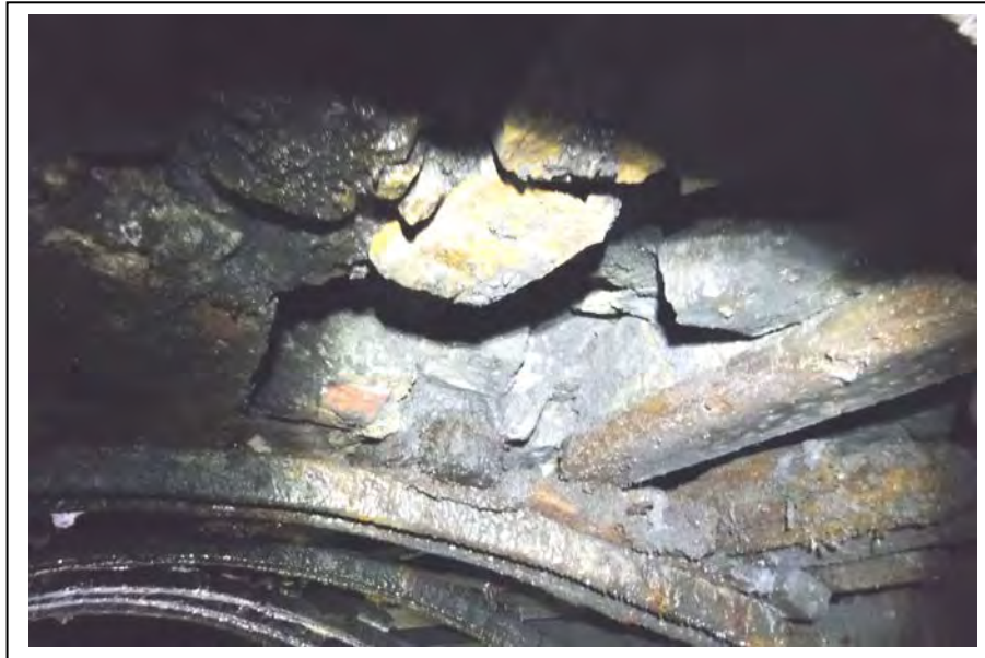
Photograph no 81: Crown at 853m (Ribs 39-40) Spalling to 250 deep x 1.1m wide
