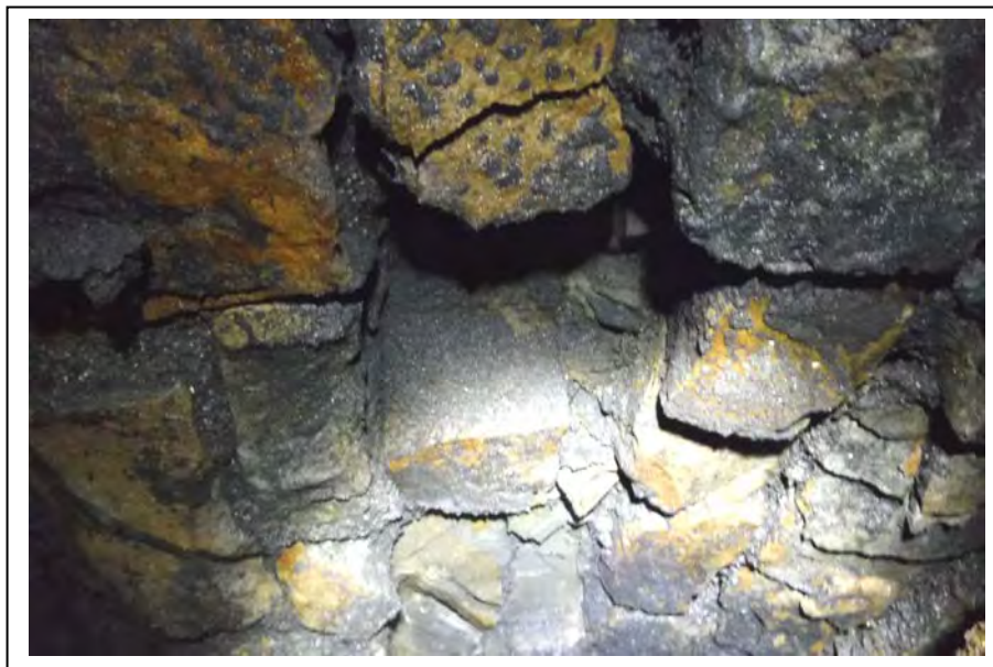
Photograph no 86: Crown at 855m (Ribs 41-420) Spalling 130 deep x 400 wide
