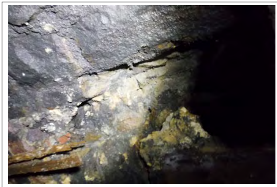
Photograph no 90: Loose "feathered in" repair to top of U/S haunch/ U/S crown at 858m 400 wide x 150 deep x 180 long
