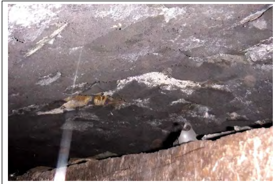
Photograph no C23: Loss of section along hinge line at 1947m Approx 0.1m 2 , appears 75 deep
