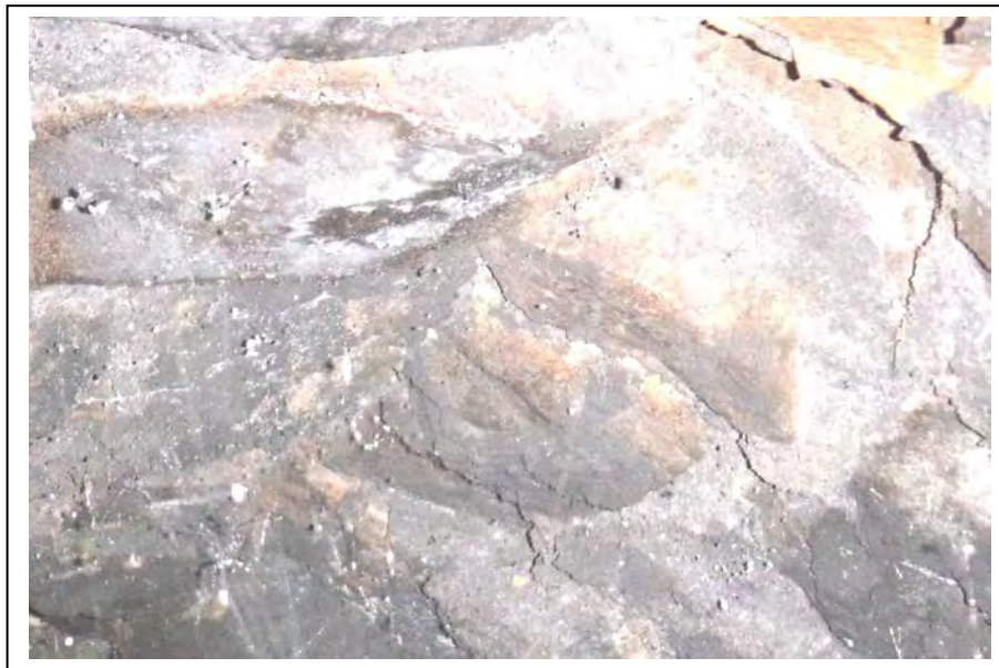
Photograph no C41: Arch flattened over Cwg ② Hinge pronounced in this area
