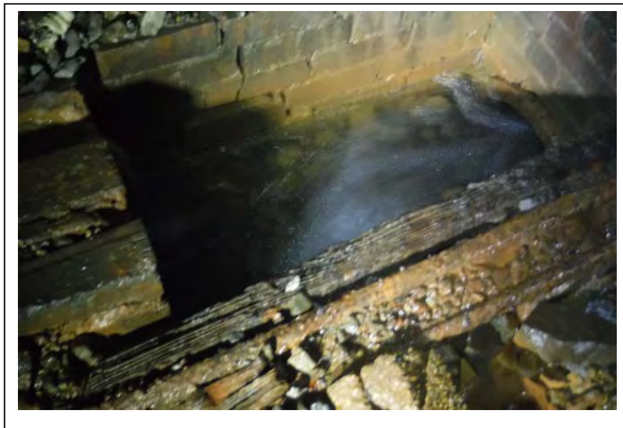
Photograph no 8: U/S sidewall at 35m Drainage flowing, all full bore (uncovered)
