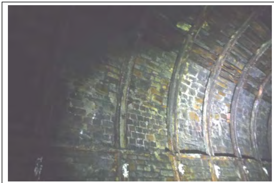
Photograph no 38: D/S haunch at 160m (Ribs 92-95) (shown) Line of misalignment visible from ground level
