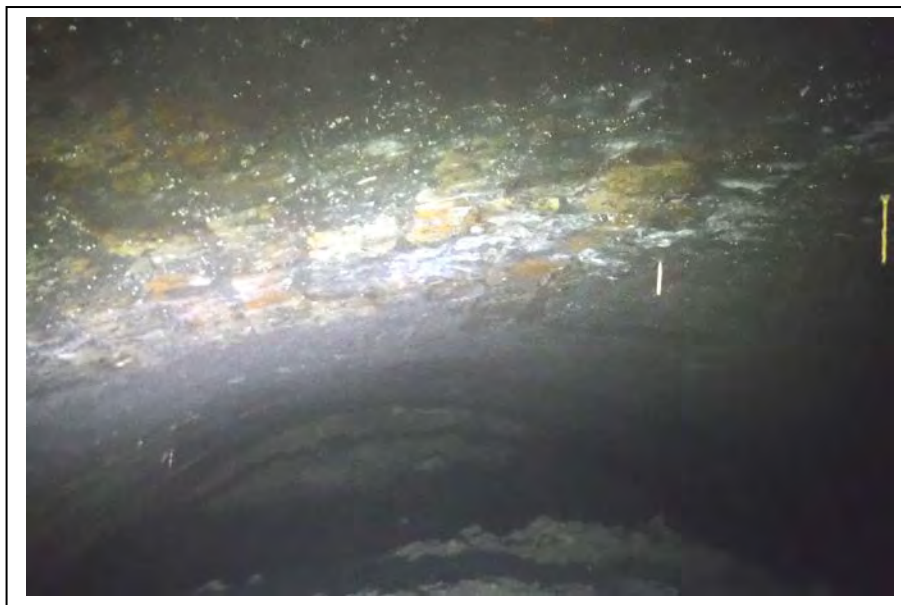
Photograph no 212: Crown to D/S haunch at 3018m Area of visible flattening of barrel form Firm to hammer
