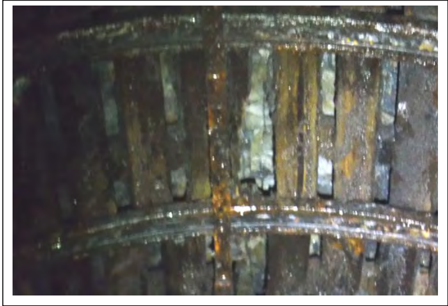
Photograph no 15: Ribs 6 – 8 Loss of section 600 wide x 180 x 75 deep Removed
