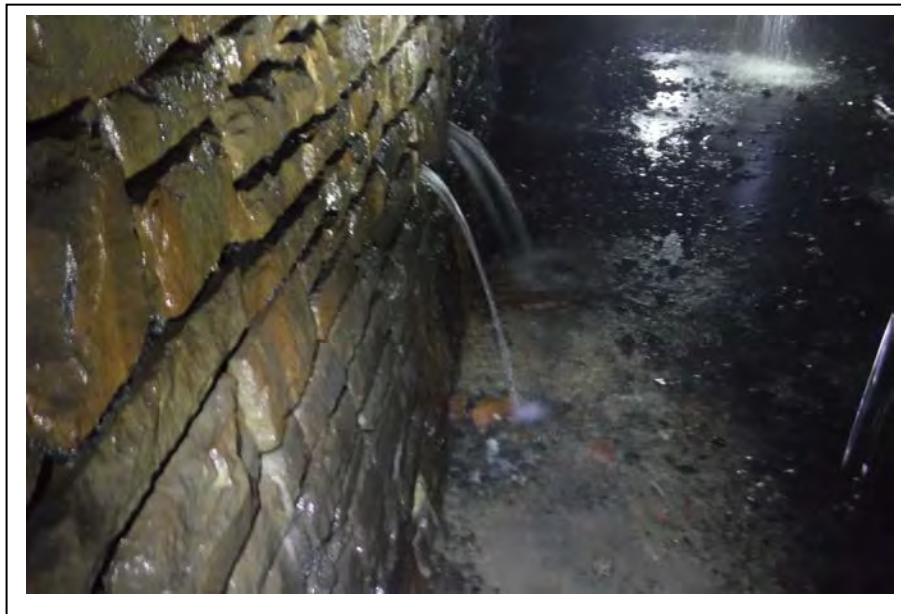
Photograph no 10: D/S sidewall at 45m Water running
