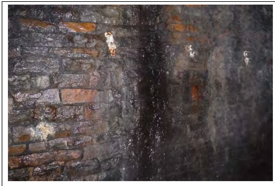
Photograph no 196: D/S haunch at 3074m Water running
