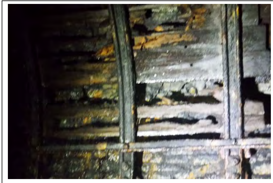
Photograph no 27: D/S haunch at 126m (Ribs 52-53) Loose material removed 200 deep over 3m 2
