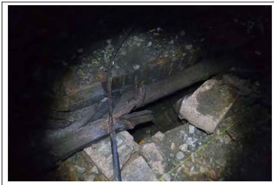
Photograph no 14: U/S sidewall at 65m Drainage flowing at full capacity
