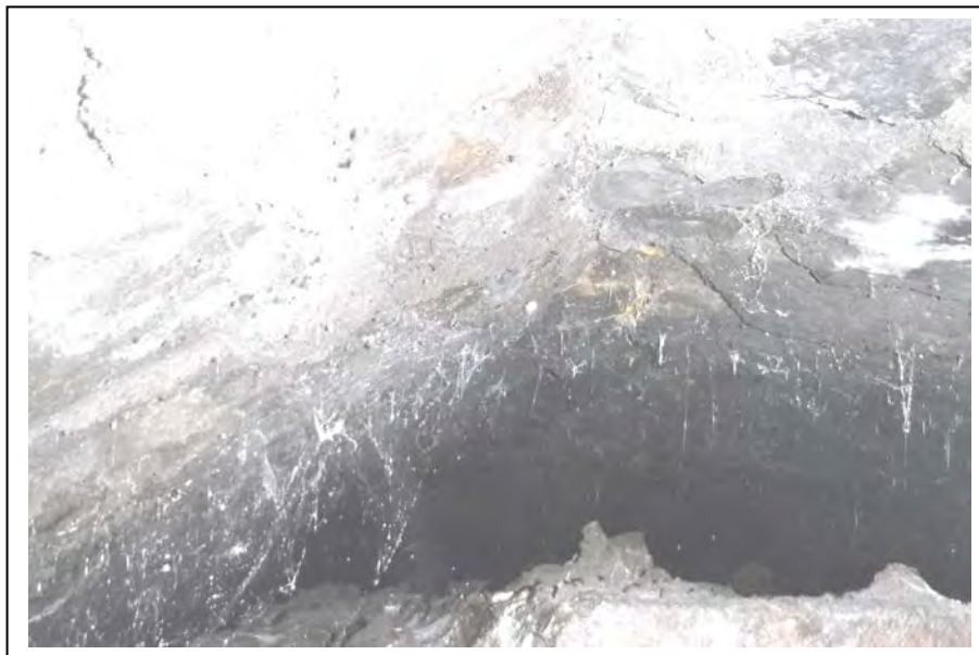
Photograph no C44: Hinge remains pronounce above LE of Cwg ③
