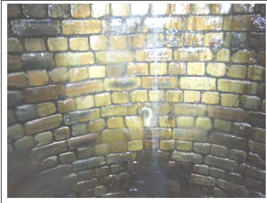
Photograph no 179: Water running from inlet at 8.5 – 10m Down-pipe remains to lower section Brickwork very wet throughout below inlet level
