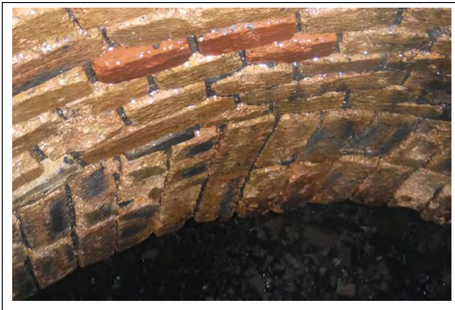
Photograph no 180: Rings in soffit at 11m below shaft level 225 thick with water staining Open joints to 15
