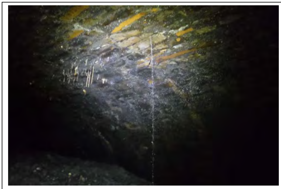
Photograph no 208: Water running to U/S haunch at 3104m
