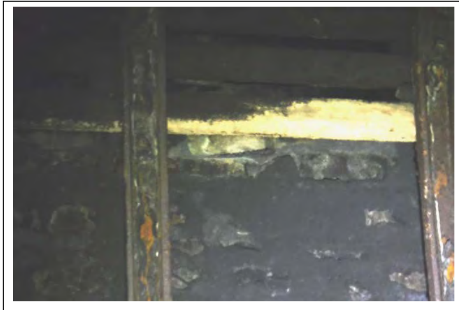
Photograph no 45: U/S haunch at 148 – 172m Defects similar to D/S haunch Separation of feathering is of much lower severity (typical view)
