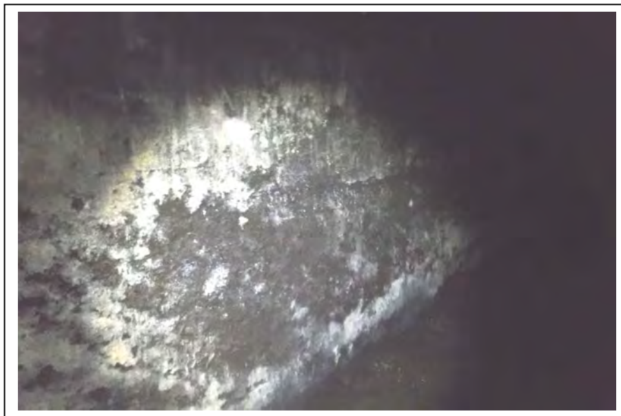
Photograph no 136: D/S sidewall at 1890m Good
