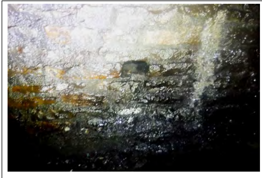
Photograph no 153: D/S sidewall at 2995m Loss of section 450 wide x 280 high x 230 deep
