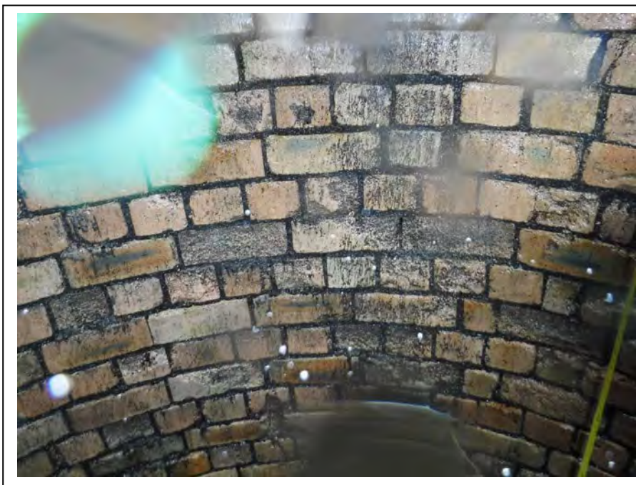
Photograph no 174: New slab level at 3.75m Odd open joints to 20
