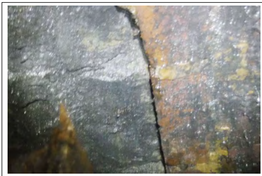
Photograph no 92: Crown at 866m (Ribs 55-56) Displacement of section to brick repair
