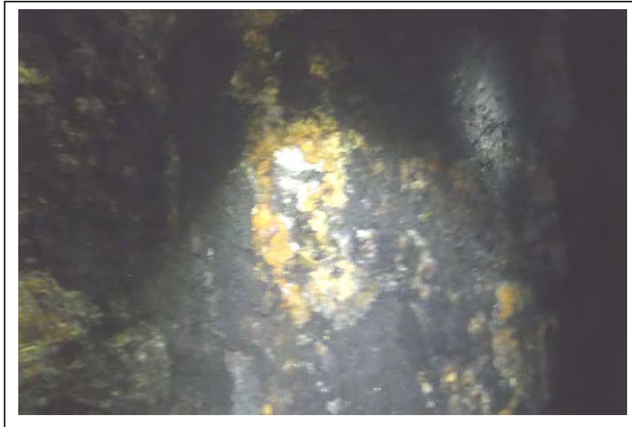
Photograph no 137: U/S refuge at 2060m Soft render around refuge (Typical)
