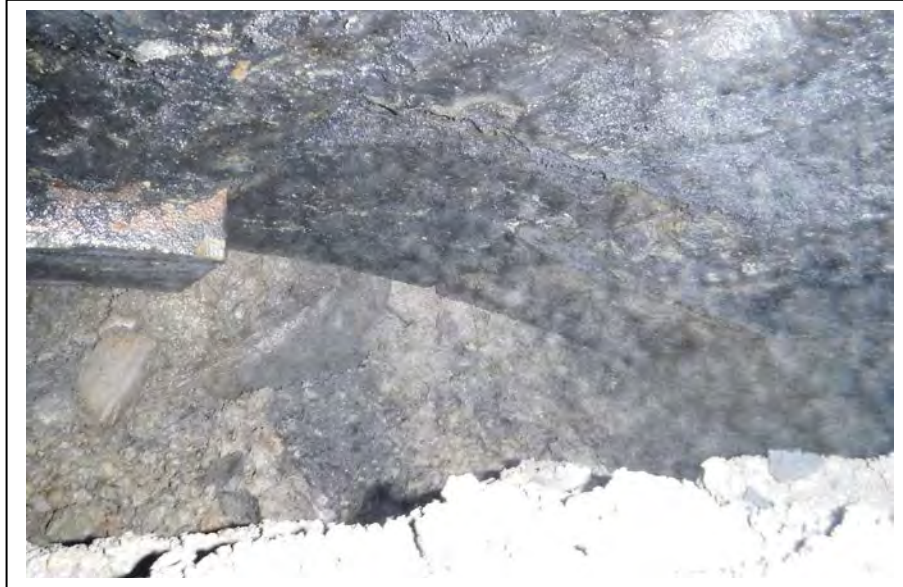
Photograph no 213: U/S voussoir haunch at 3132m Voussoirs to haunch in very good condition Wet
