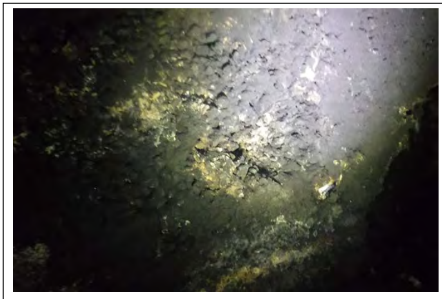
Photograph no 58: Relieving arches heavily spalled due to poorly compacted concrete (Typical view)
