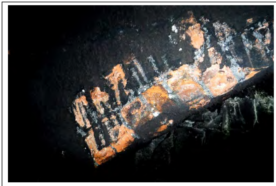
Photograph no 128: D/S relieving arch at 1385m Spalling 40 x 0.25m 2
