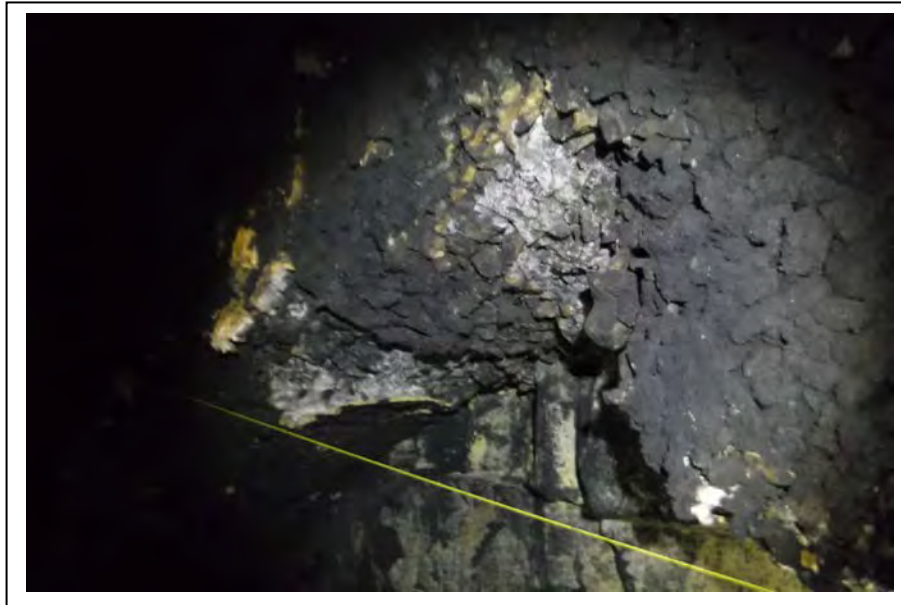
Photograph no 59: Relieving arches heavily spalled due to poorly compacted concrete (Typical view)
