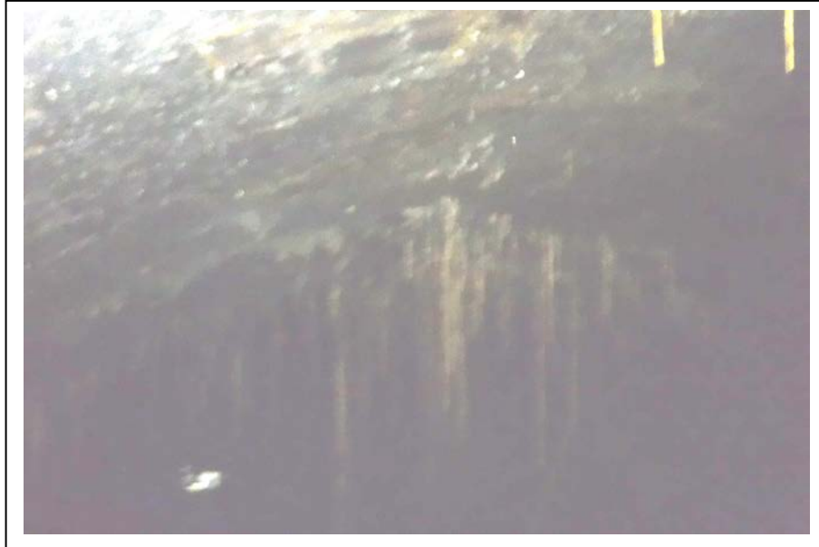
Photograph no 205: Haunch to haunch at 3100m Possible deformation of crown (may have dropped 50-100) Firm to hammer
