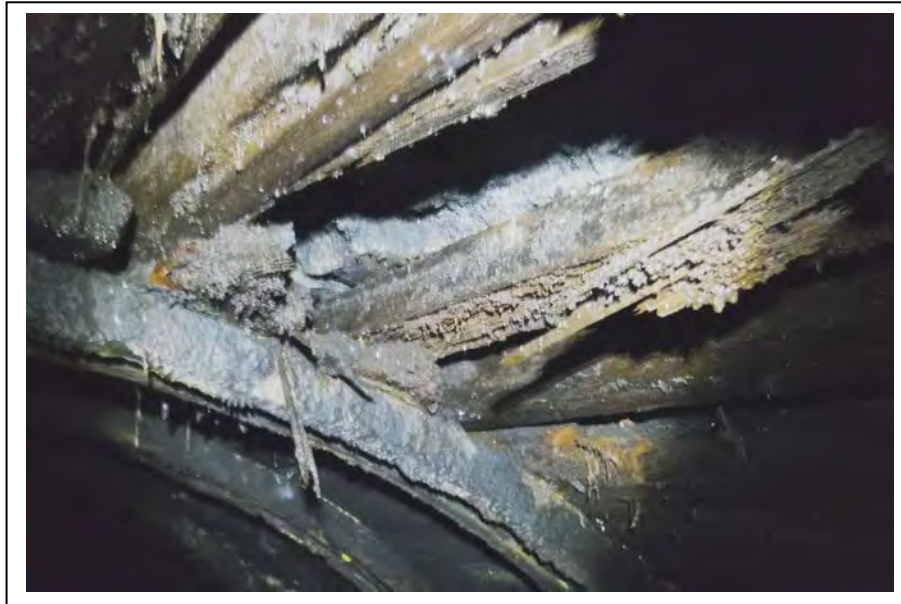
Photograph no 79: Crown at 851m (Ribs 37-38) Spalling to 250 deep
