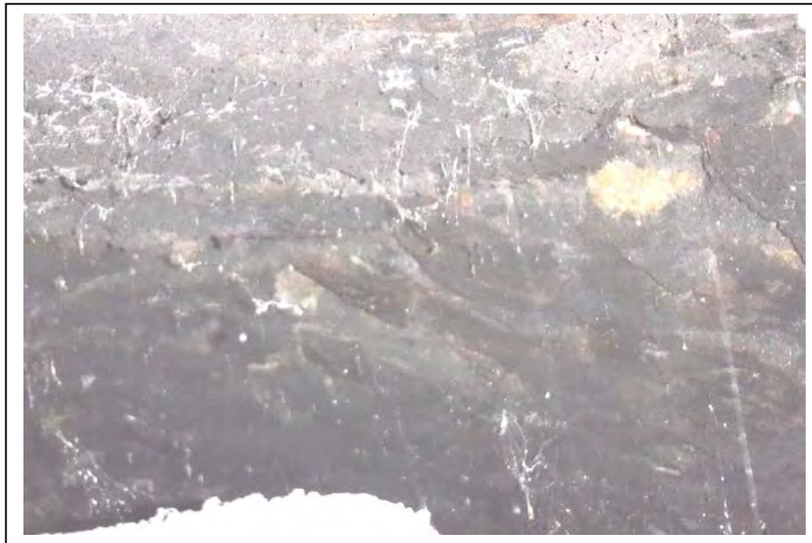
Photograph no C40: Arch flattened over Cwg ② Hinge pronounced in this area
