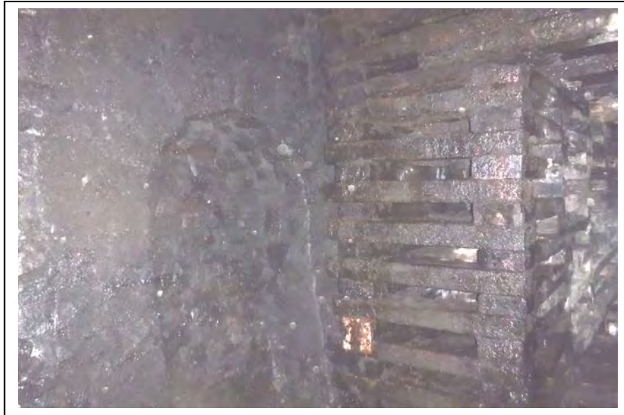
Photograph no C19: Cwg ③ CE US sidewall
