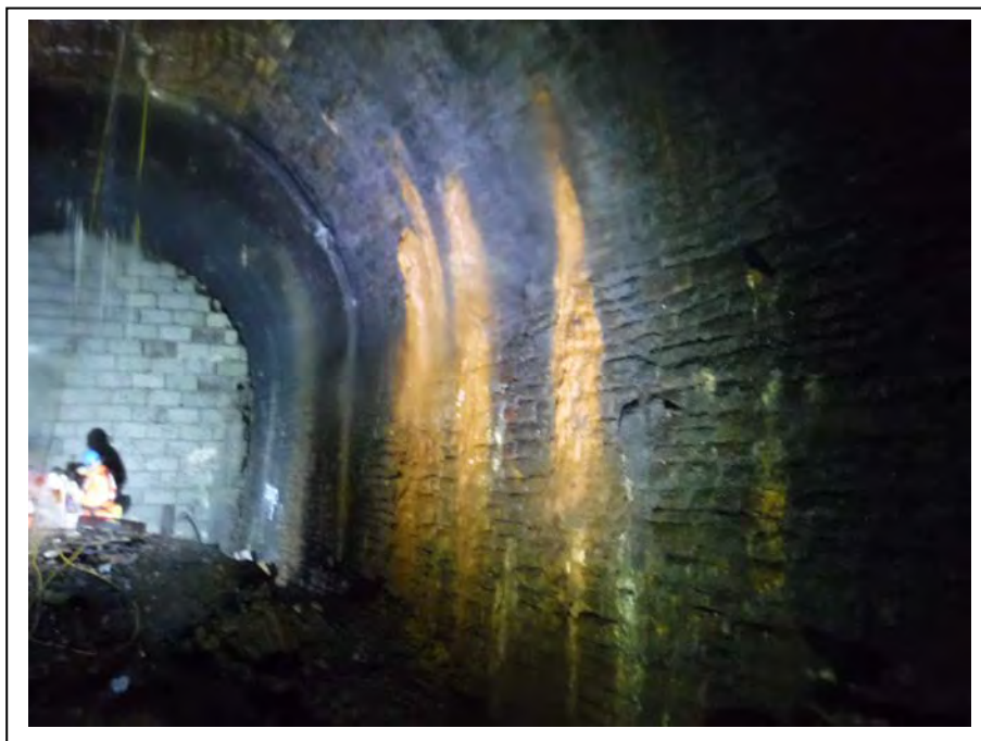
Photograph no 160: D/S sidewall and haunch at 3035m Water staining
