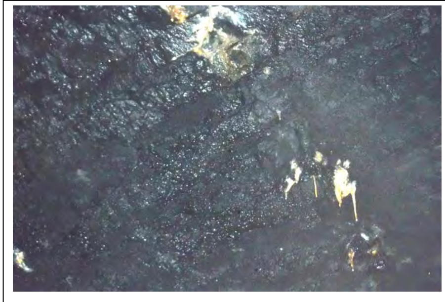
Photograph no 197: U/S haunch at 3074m Water running at line of old drainage
