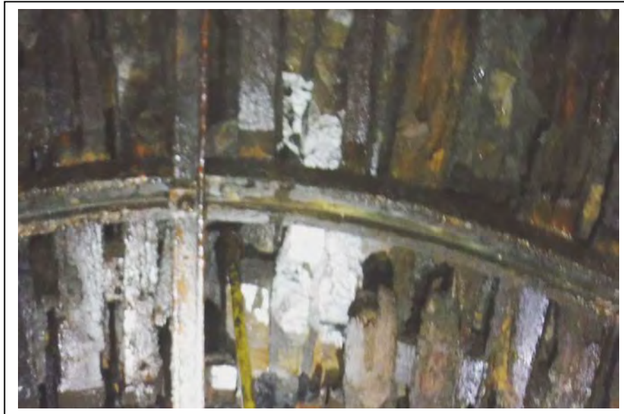
Photograph no 17: Crown between ribs 18 and 19 Loss of section 600 wide x 200 max deep
