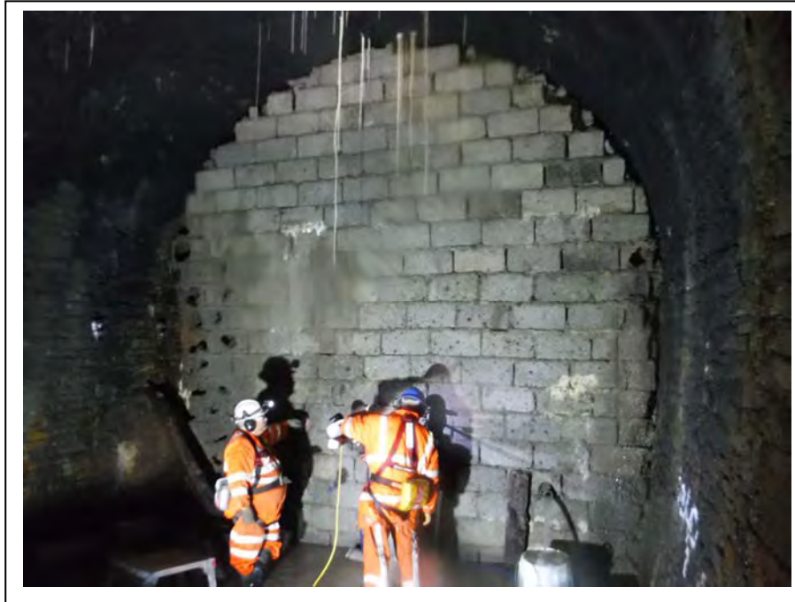
Photograph no 165: Diaphragm wall at 3042m (blockwork backed with mass concrete) To full height (Coring in progress)
