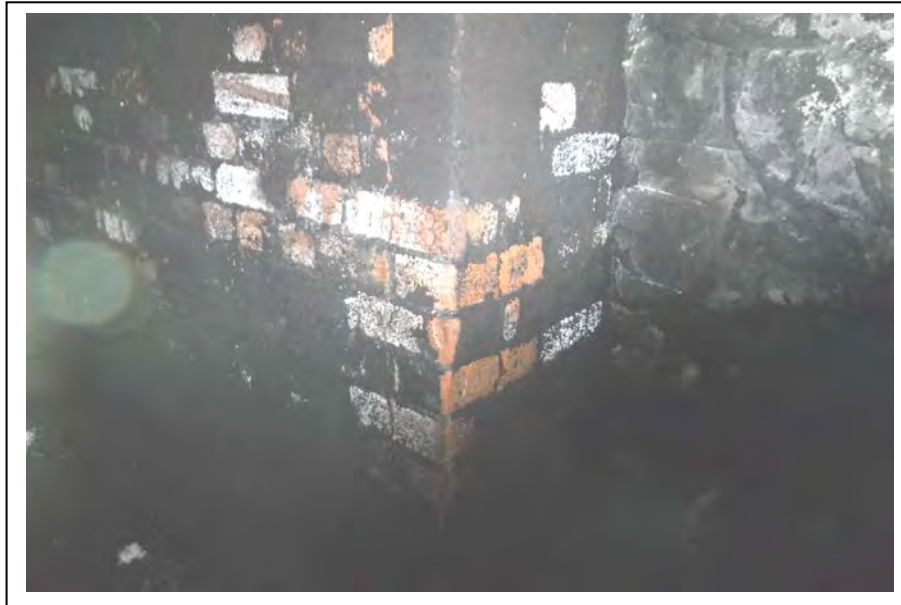
Photograph no 127: D/S relieving arch at 1370m 2no vertical fractures to relieving arch pier open 5mm on either side of quoin
