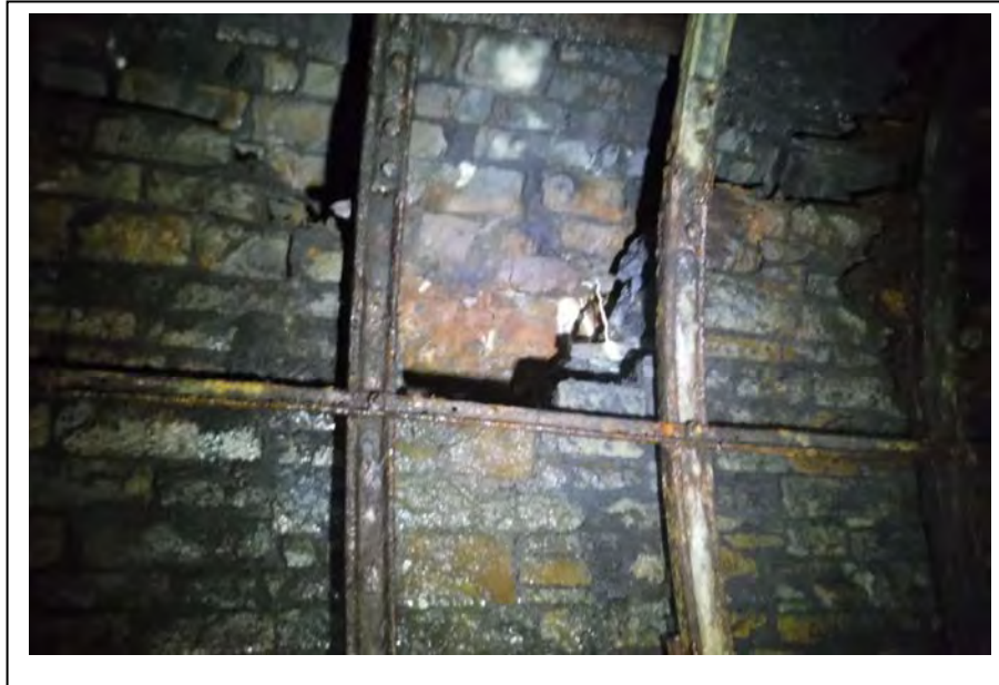
Photograph no 35: D/S haunch at 152m (Ribs 80-81) Loss of section 900 wide x 500 deep (to natural rock)
