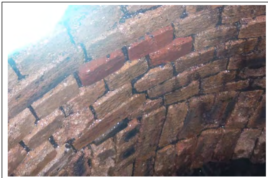
Photograph no 182: Shaft at 11m Open joints to 20mm above extrados with odd losses to cut bricks
