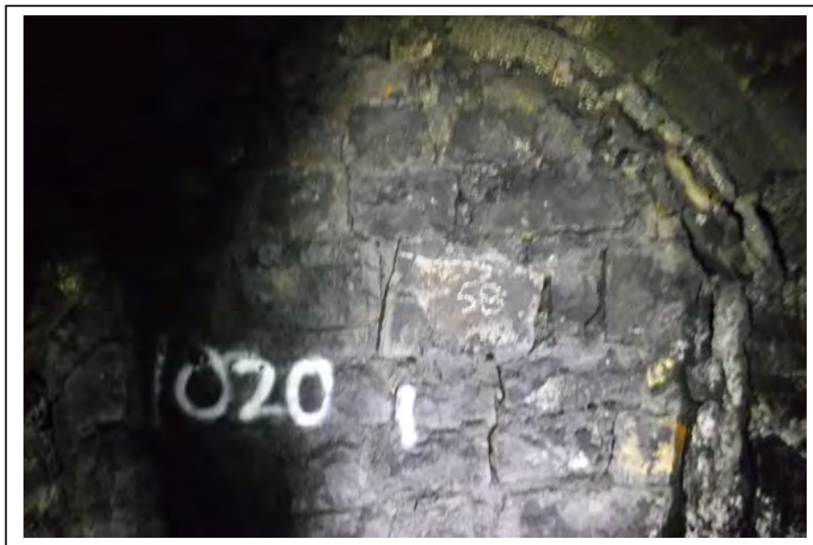
Photograph no 106: D/S refuge at 1020m Vertical step joint fracture to refuge rear wall with loose brickwork adjacent 900 long
