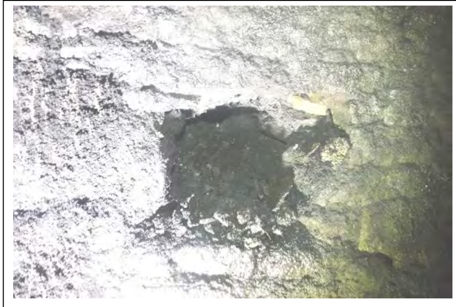
Photograph no 155: U/S sidewall at 2995m Loss of section 400 wide x 350 high x 500 deep
