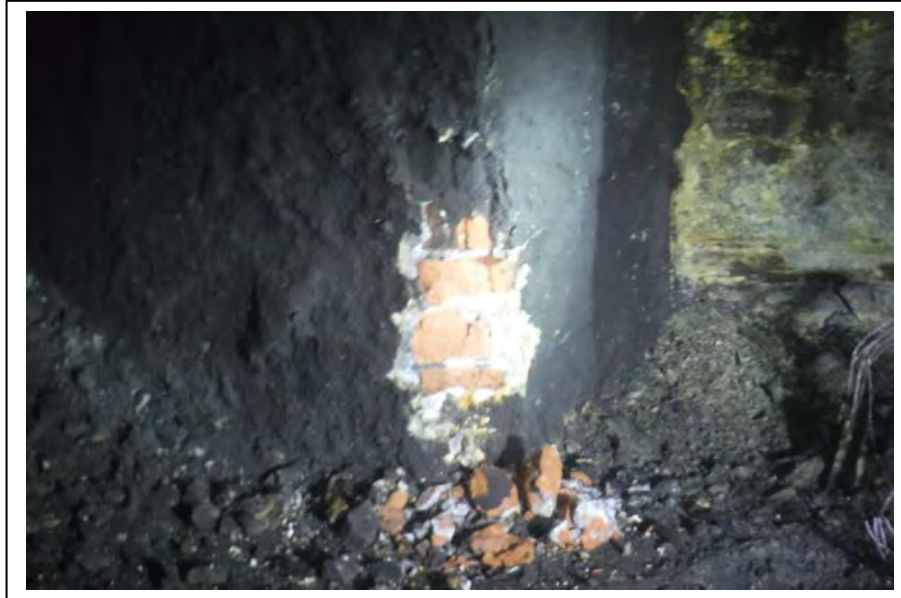
Photograph no 141: D/S refuge at 2395m Spalling 50 to DL refuge quoin
