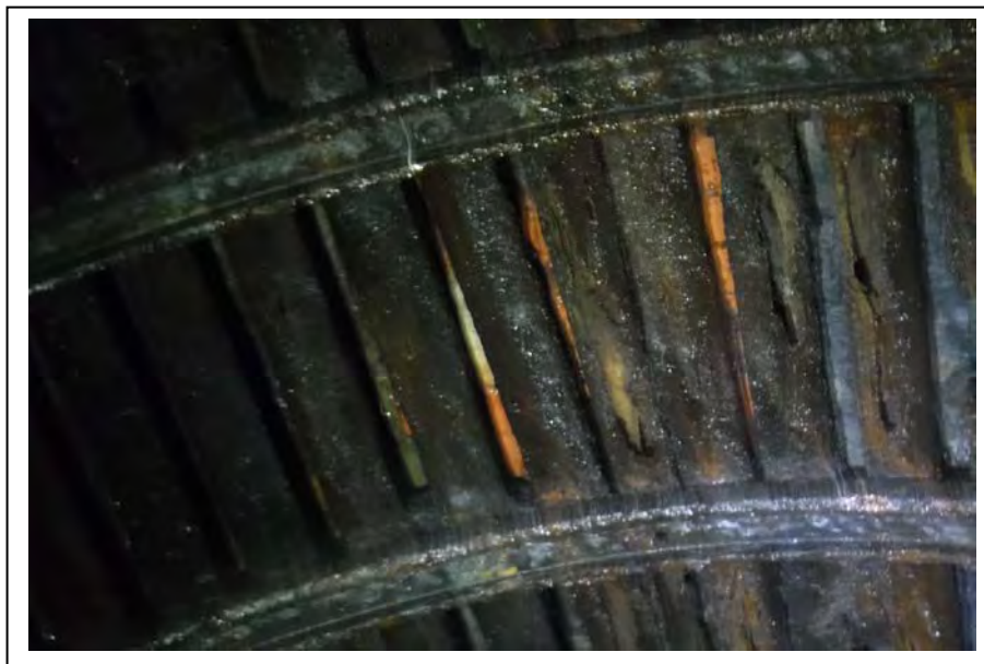
Photograph no 26: Crown at 124m Brick repair noted between ribs 50 & 51 Sound when tapped
