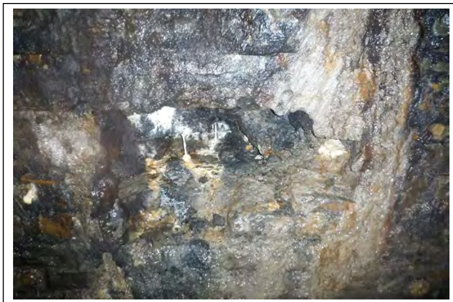
Photograph no 190: U/S sidewall at 3056m Loss of section 860 wide x 500 high x 500 deep
