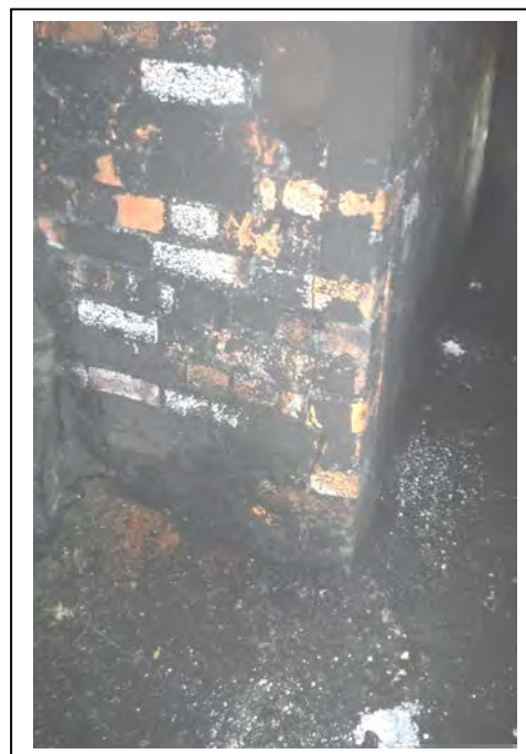
Photograph no 126: Relieving arch at 1365m 2no vertical fractures to relieving arch pier open 10mm on either side of quoin
