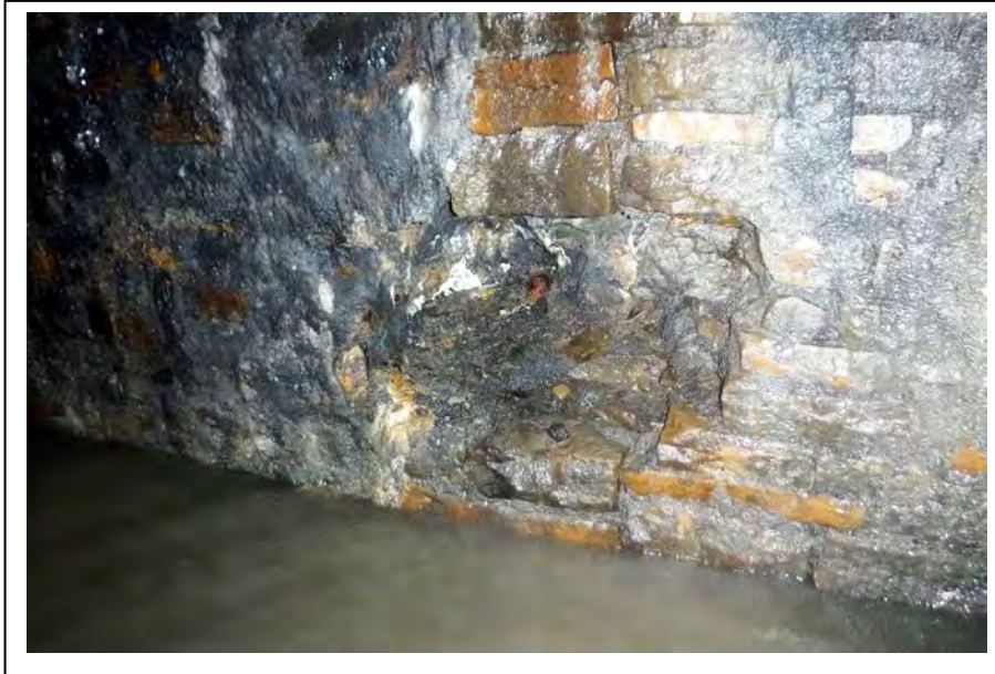
Photograph no 191: D/S sidewall at 3056m Loss of section 1000 wide x 500 high x 650 deep
