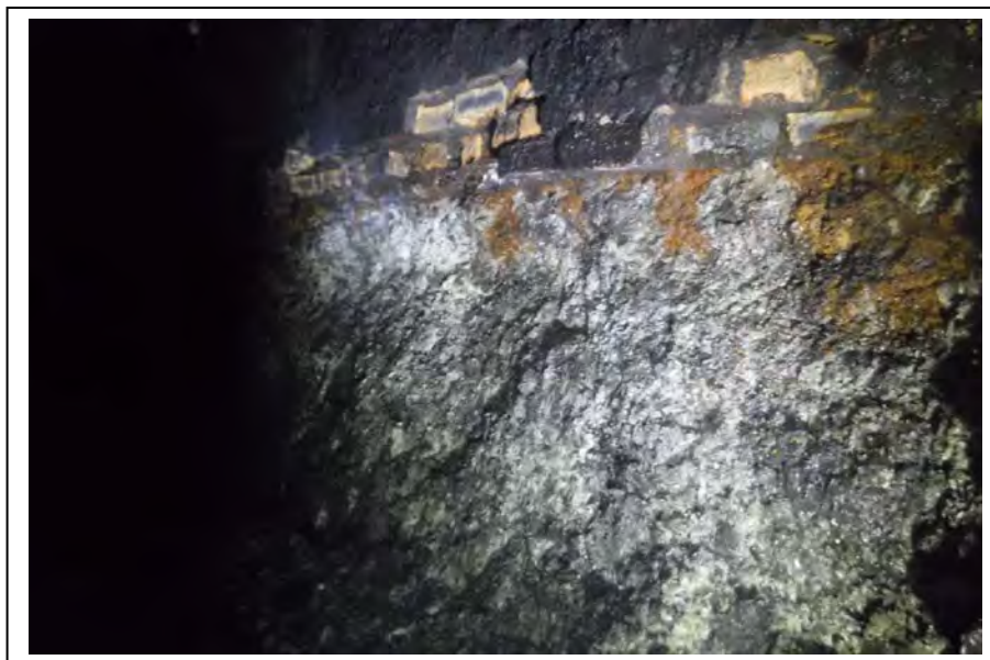
Photograph no 146: D/S sidewall at 2575m Failing brickwork repair 2500 wide x 1330 high x 200 deep
