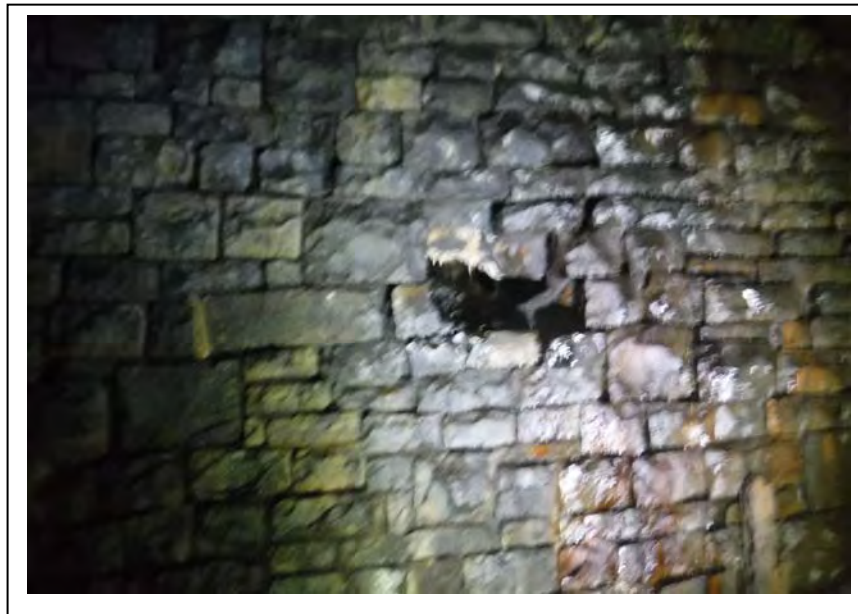
Photograph no 6:U/S sidewall at 25m Loss of section 440 high x 510 wide x 600 deep
