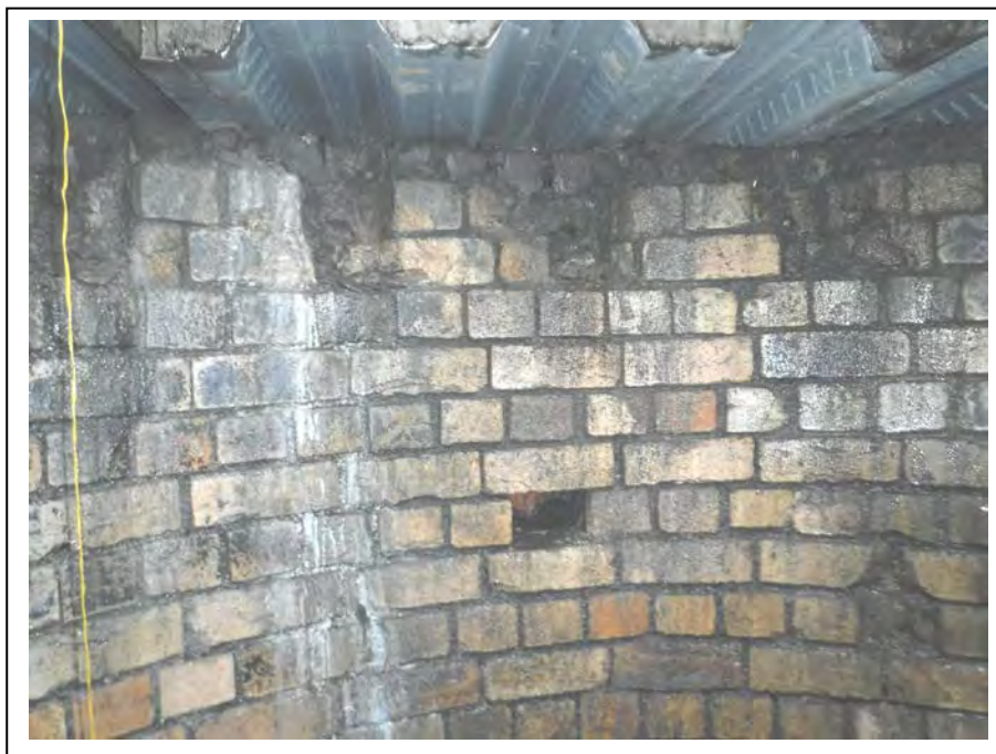
Photograph no 170: New slab level - 0.75m: Bricks cut out for platform support during original construction (no timber remains)
