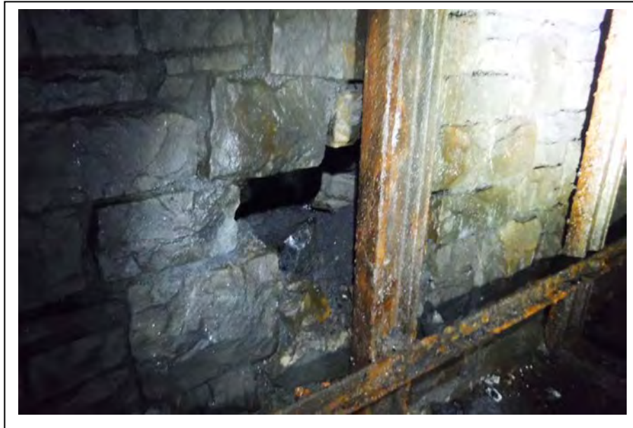
Photograph no 47: U/S sidewall at 195m (Ribs 127-128) Loss of section 400 high x 500 wide x 600 deep
