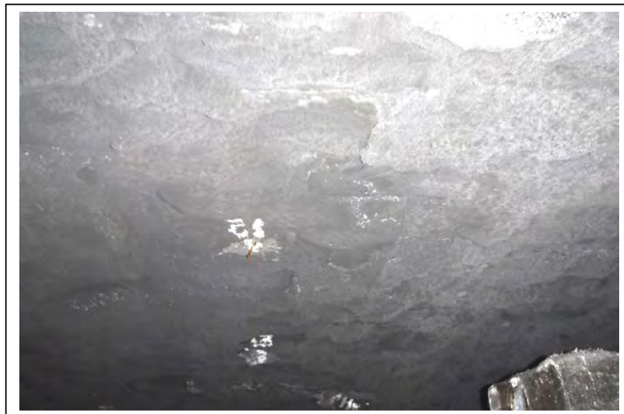
Photograph no C20: Barrel at LE of Cwg is firm
