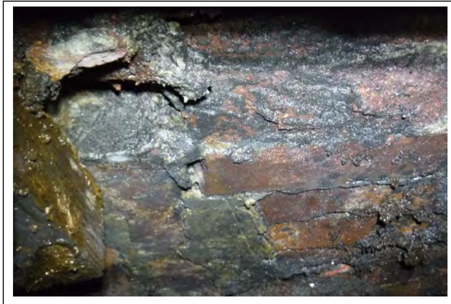
Photograph no 85: Crown at 854m (Ribs 40-41) Spalling 120 deep x 500 wide
