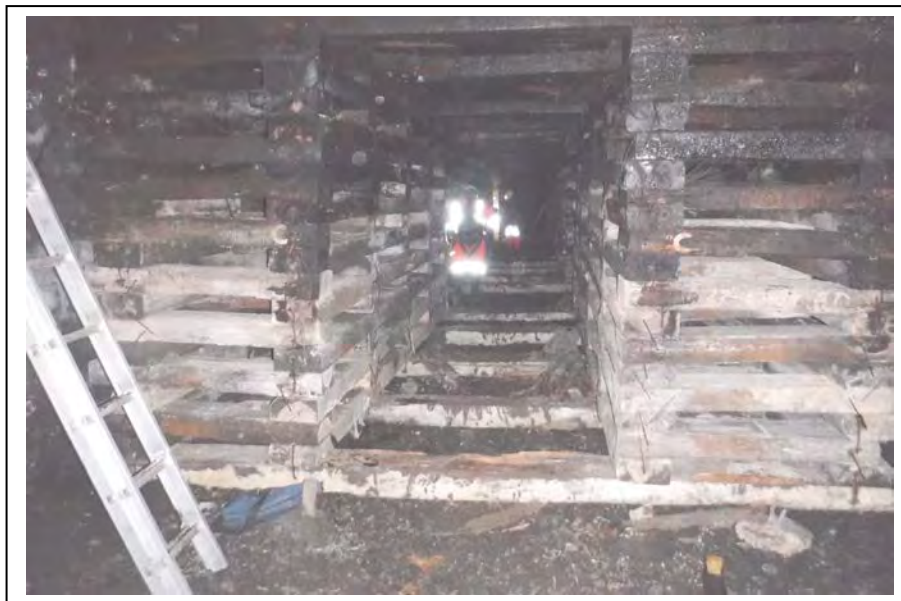
Photograph no C2: Cwg ① LE crown
