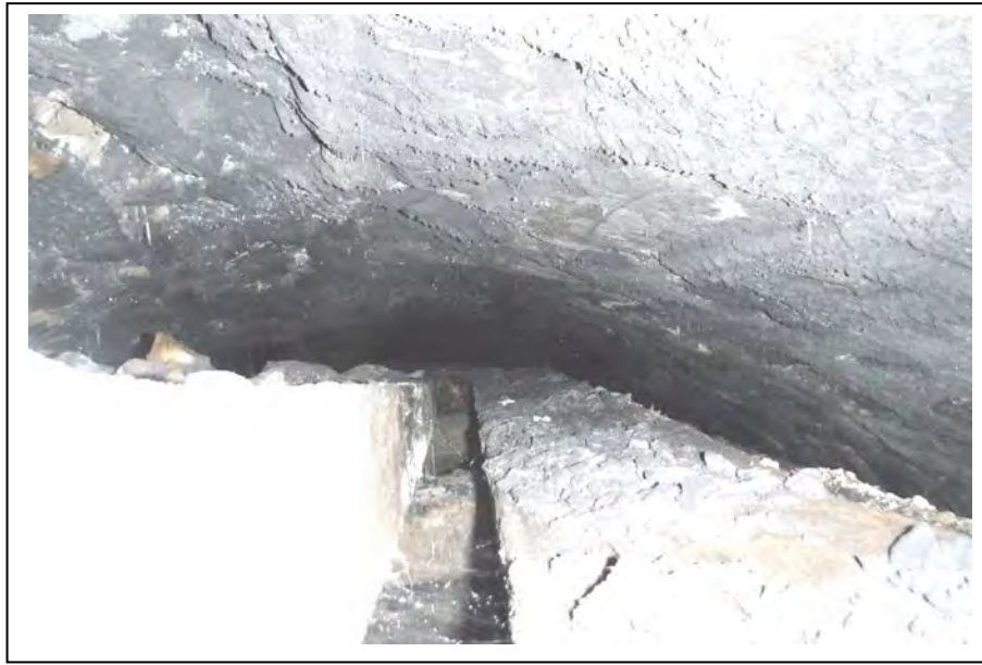
Photograph no C37: No evidence of packing to US haunch/ crown 1952m shown
