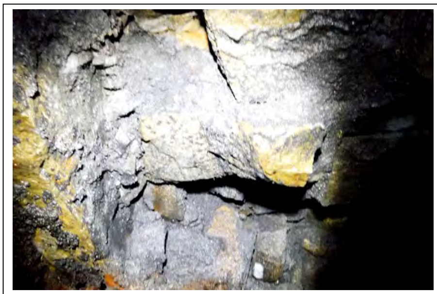
Photograph no 80: Crown at 852m (Ribs 38-39) Spalling to 150 deep
