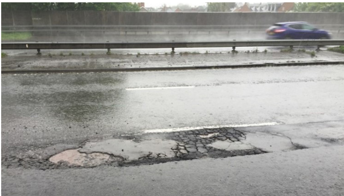
Fig.21 Example of waterproofing failure on the SRN causing surfacing breakdown
