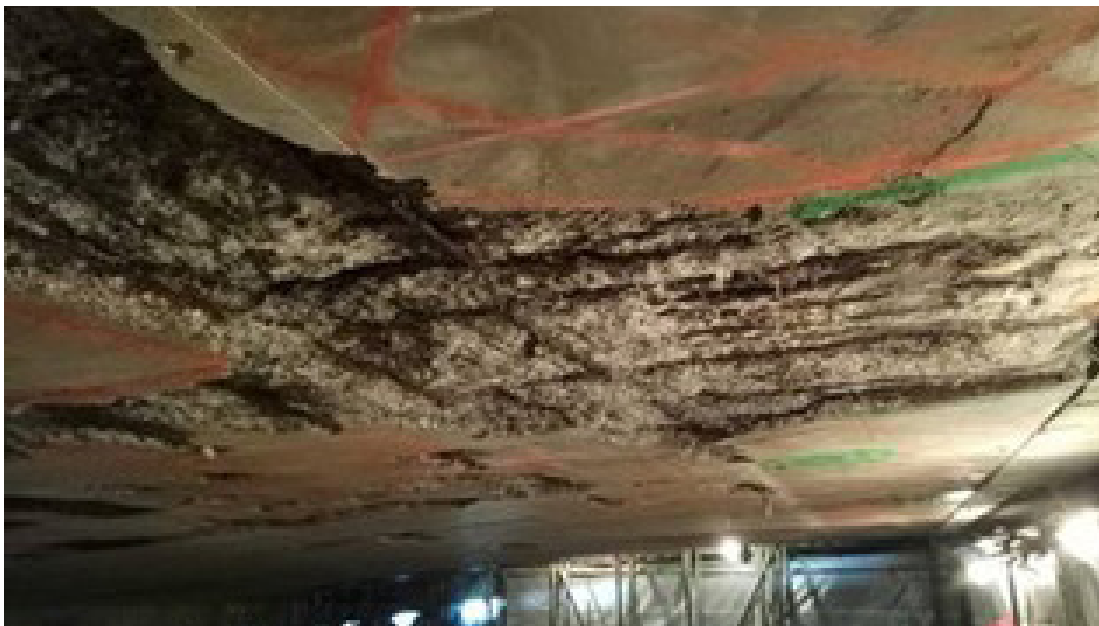
Fig.22 M4 Tawe River Bridge showing severe corrosion of bridge reinforcement
