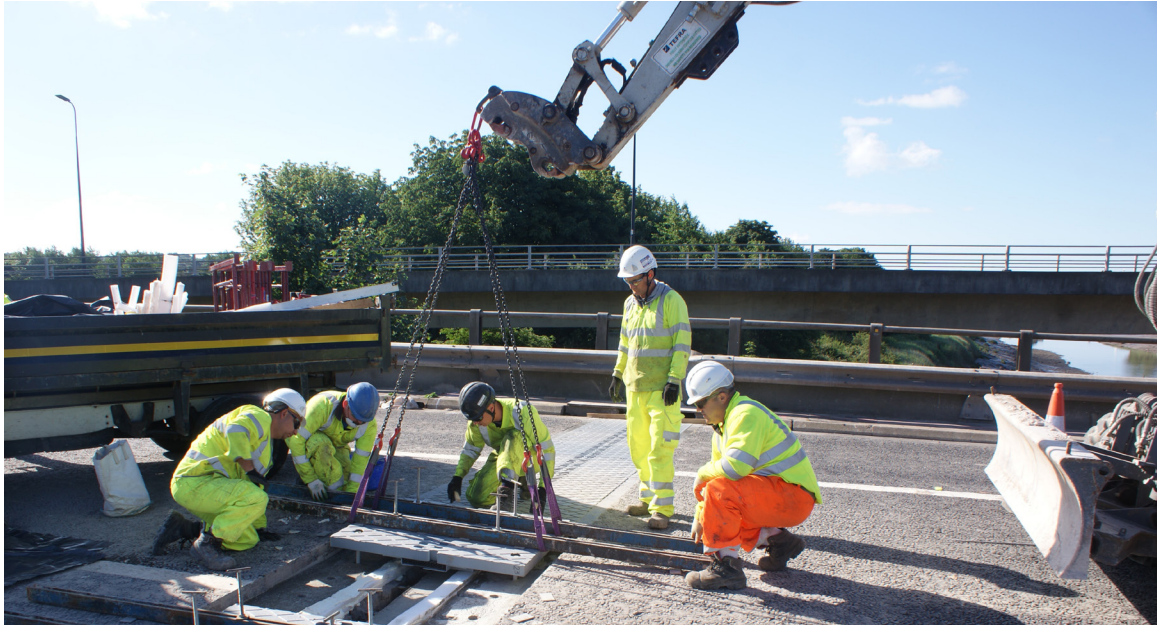
Fig.19 shows an effective maintenance intervention as bridge joint replacement M4 Usk Bridge
