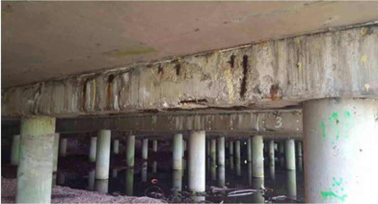
Fig.14 Severe concrete deterioration on the M4 Maplas Viaduct
