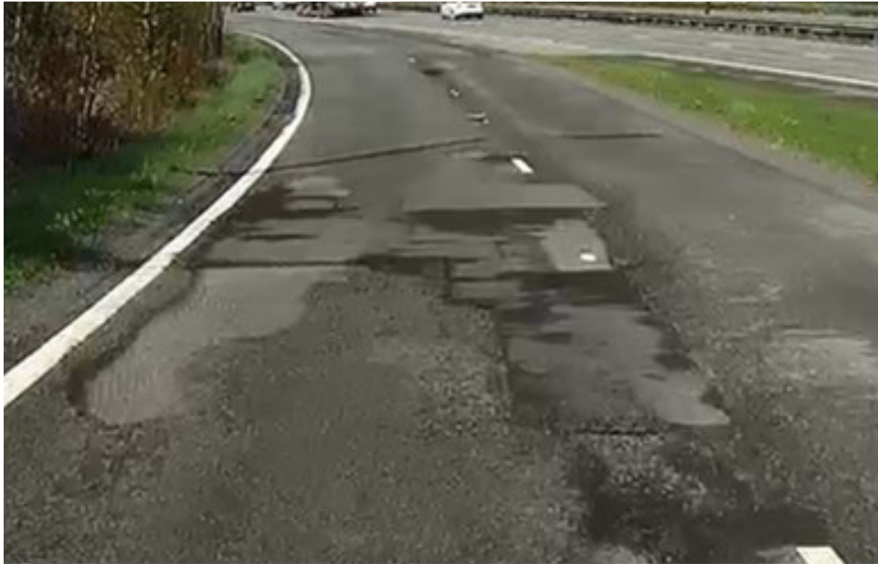
Fig.3 Example of the deteriorating condition of the SRN
