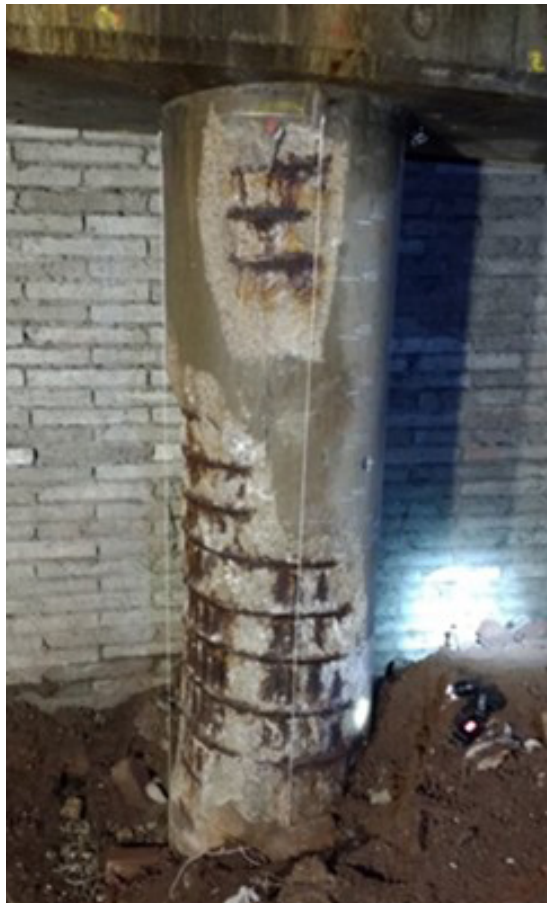
Fig.20 M4 Malpas example of severe concrete deterioration on a bridge pier
