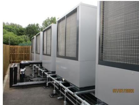
Inside the heat pump compound
