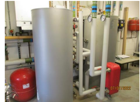
Solar thermal & hot water service cylinders 35
