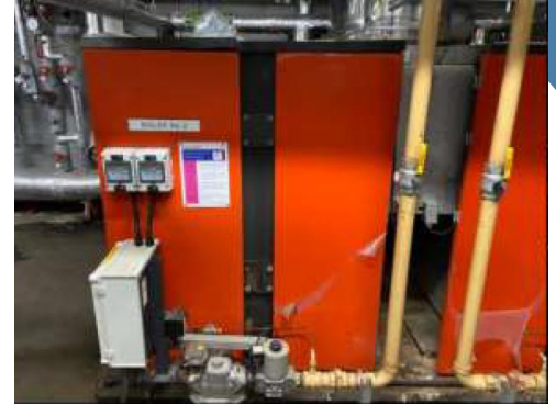
Existing gas boilers
