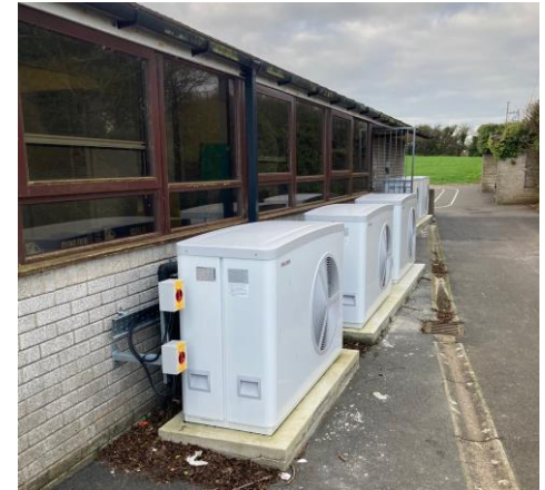
New air source heat pumps located outside the existing boiler room
