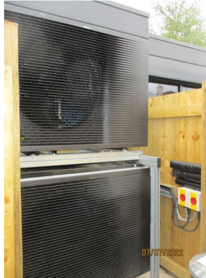
External heat pumps
