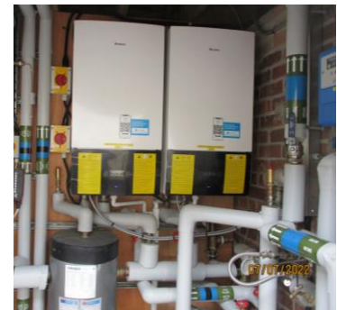
Supplementary direct electric boilers
