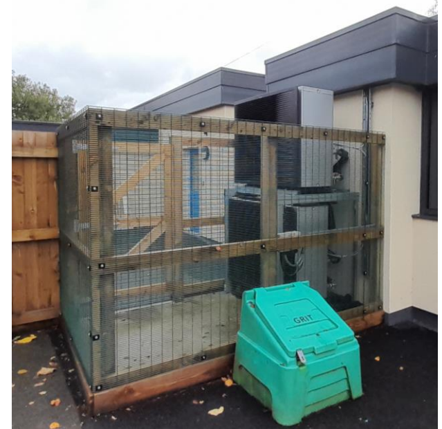
Nursery exterior with heat pump enclosure
