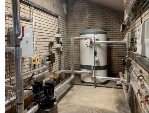
Air source heat pump pipework feeds into a buffer vessel with outflow feeding existing pipework circuits via a new pump. The buffer vessel also includes 2 x 6 kW immersion heaters.
