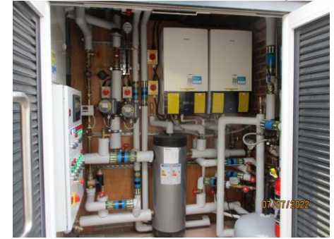
Inside the plant room
