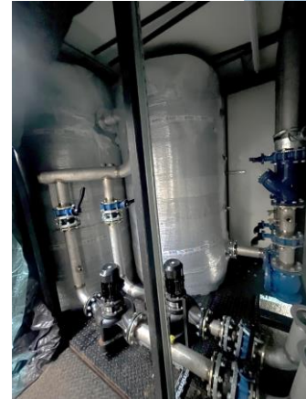
Heat pump buffer tanks within the modular plant room
