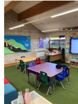
Existing pipework feeds new low temperature fan convectors. Note LED lighting has been installed.
