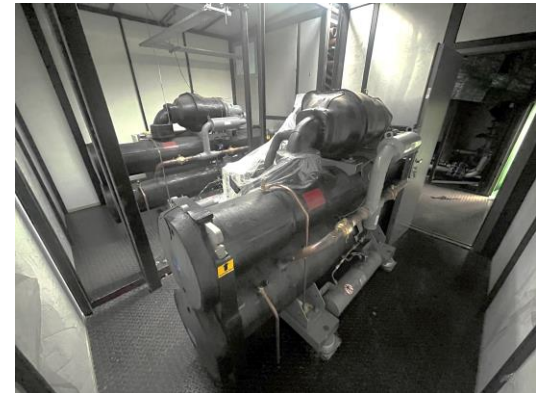
Two water source heat pumps within the modular plantroom
