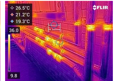
Thermal insulation is missing on brackets and valves with associated heat losses and waste. It was noted that external insulation is via domestic grade 'armaflex' and exposed brackets are causing excessive heat losses.
