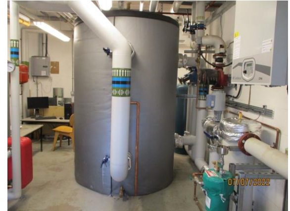
2500L Buffer vessel – now envisaged as too small to act as a heat store
