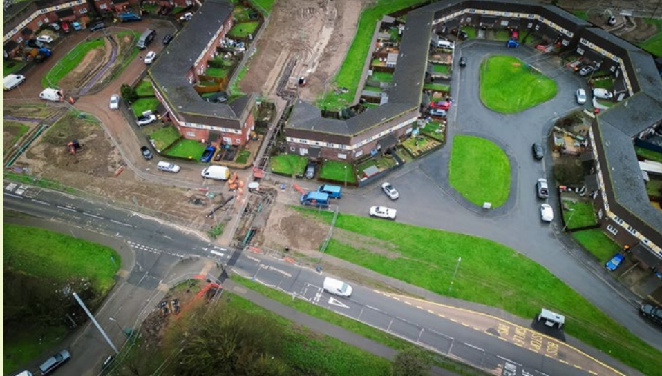
Duffryn housing heat network retrofit (image credit: Vital Energy)
