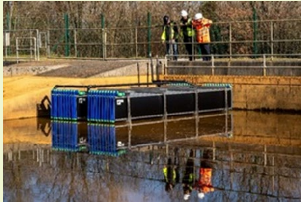
Heat exchangers at the Lindsay mine water treatment site (image credit: UK government)
