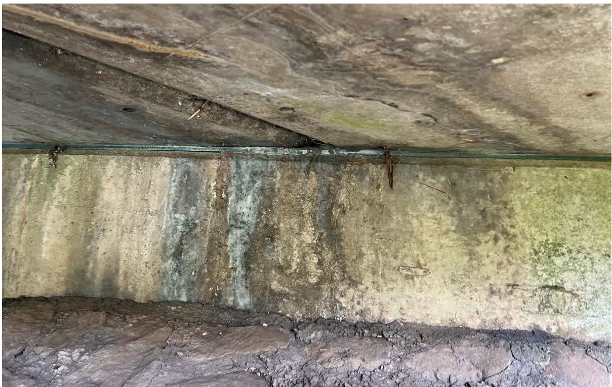
Photograph 64 - Span 3. Historic water seepage & algae staining to north abutment.
