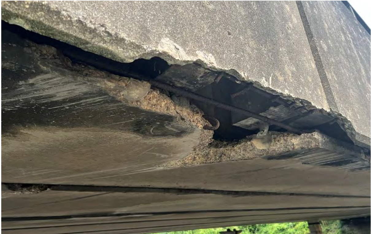
Photograph 21 - Span 2 E/B, beam 1. Area of spalling with exposed reinforcement exhibiting minor corrosion, measuring 1100x600x100mm.
