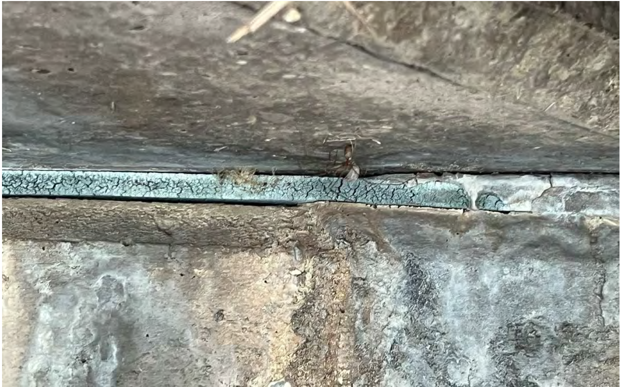
Photograph 69 - Span 3, north abutment. Minor cracking to strip bearings.
