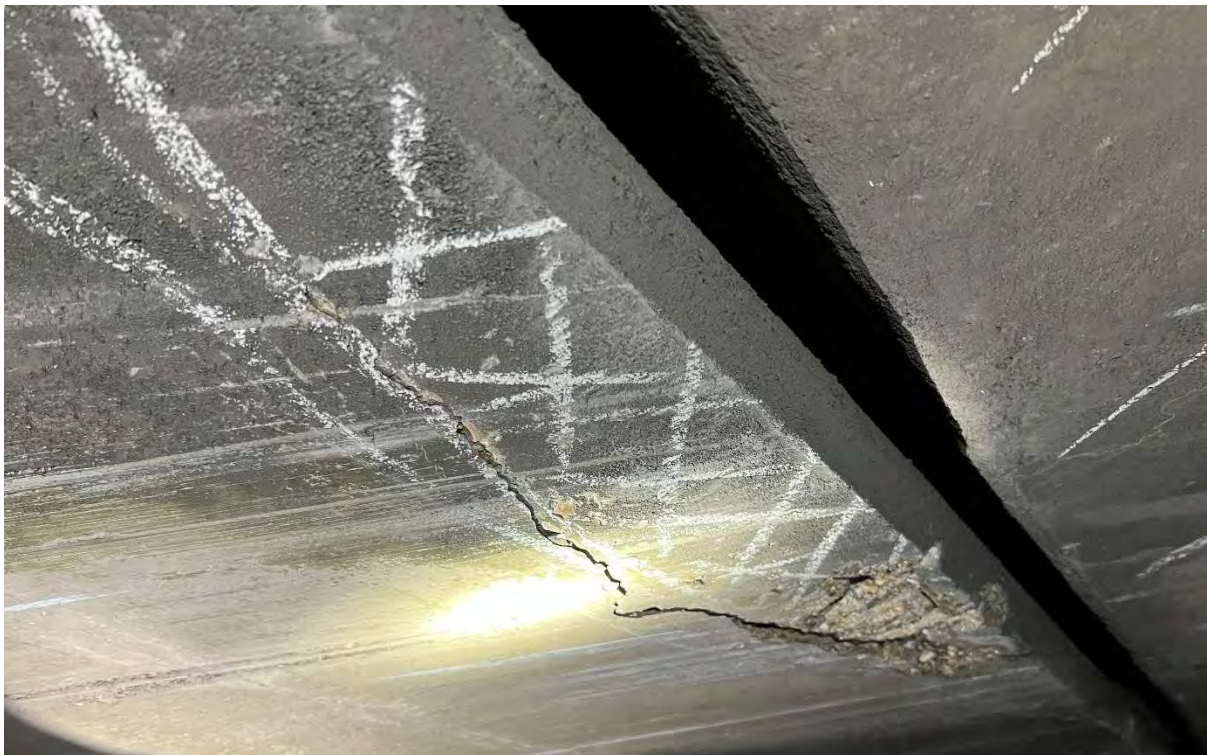
Photograph 34 - Span 2 E/B, beam 4. Area of spalling and delamination, measuring 1000x200mm.
