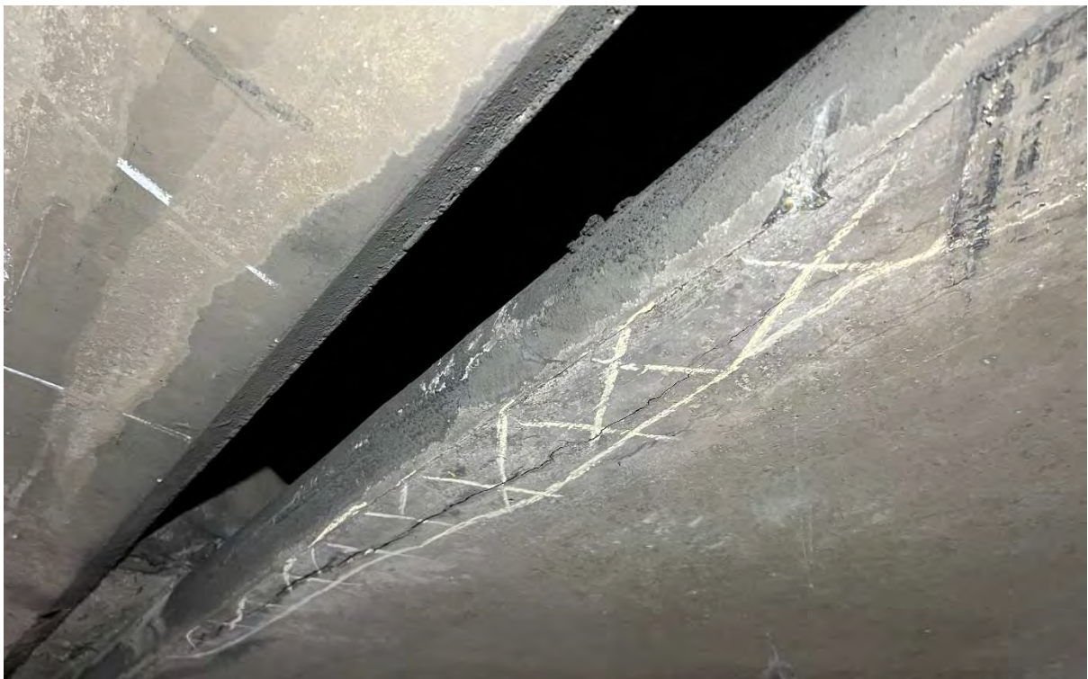
Photograph 32 - Span 2 E/B, beam 3. Area of delamination, measuring 1100x100mm.
