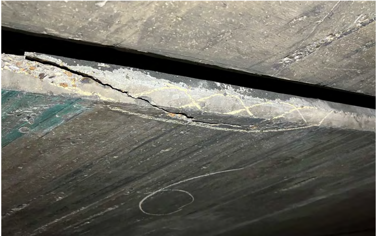
Photograph 35 - Span 2 E/B, beam 4. Area of delamination to beam soffit, measuring 600x100mm.
