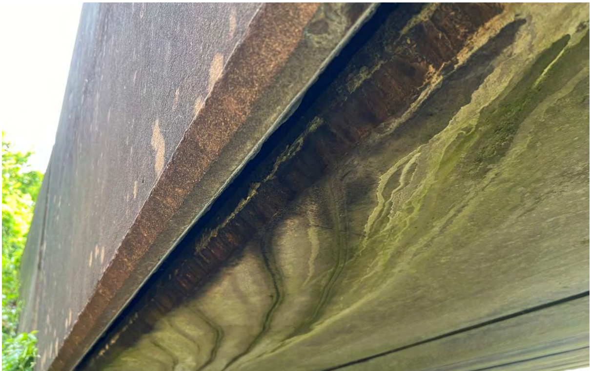
Photograph 62 - Water ingress between parapet fascia panels and deck beams.
