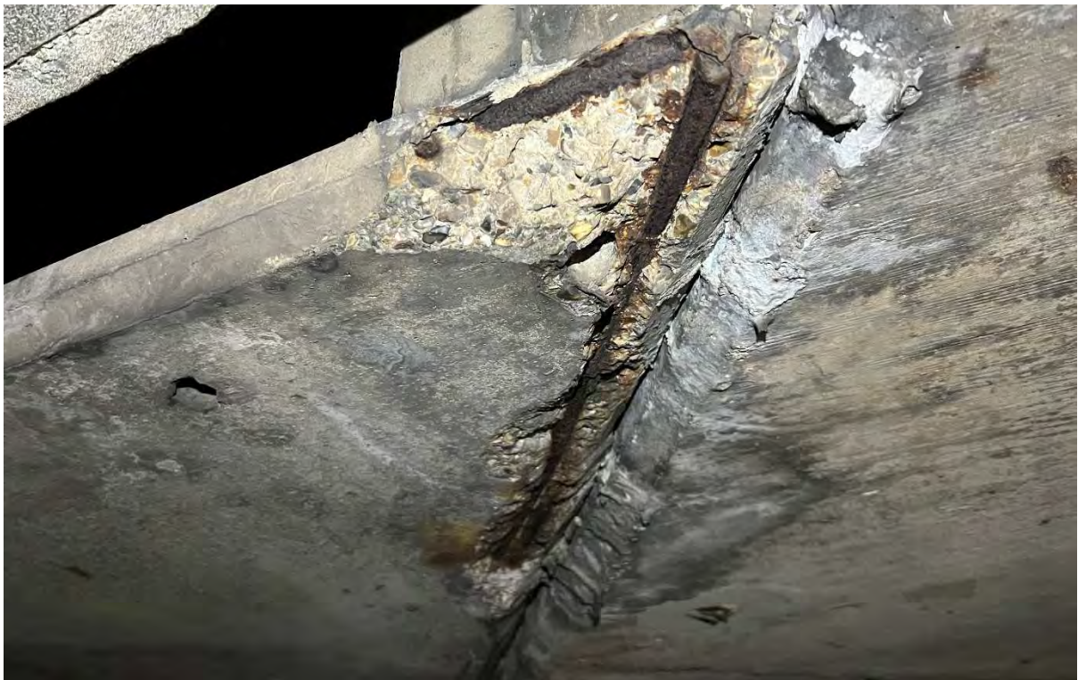
Photograph 8 - Span 1, beam 9. Area of spalling with exposed reinforcement exhibiting minor corrosion, measuring 700x100x15mm.
