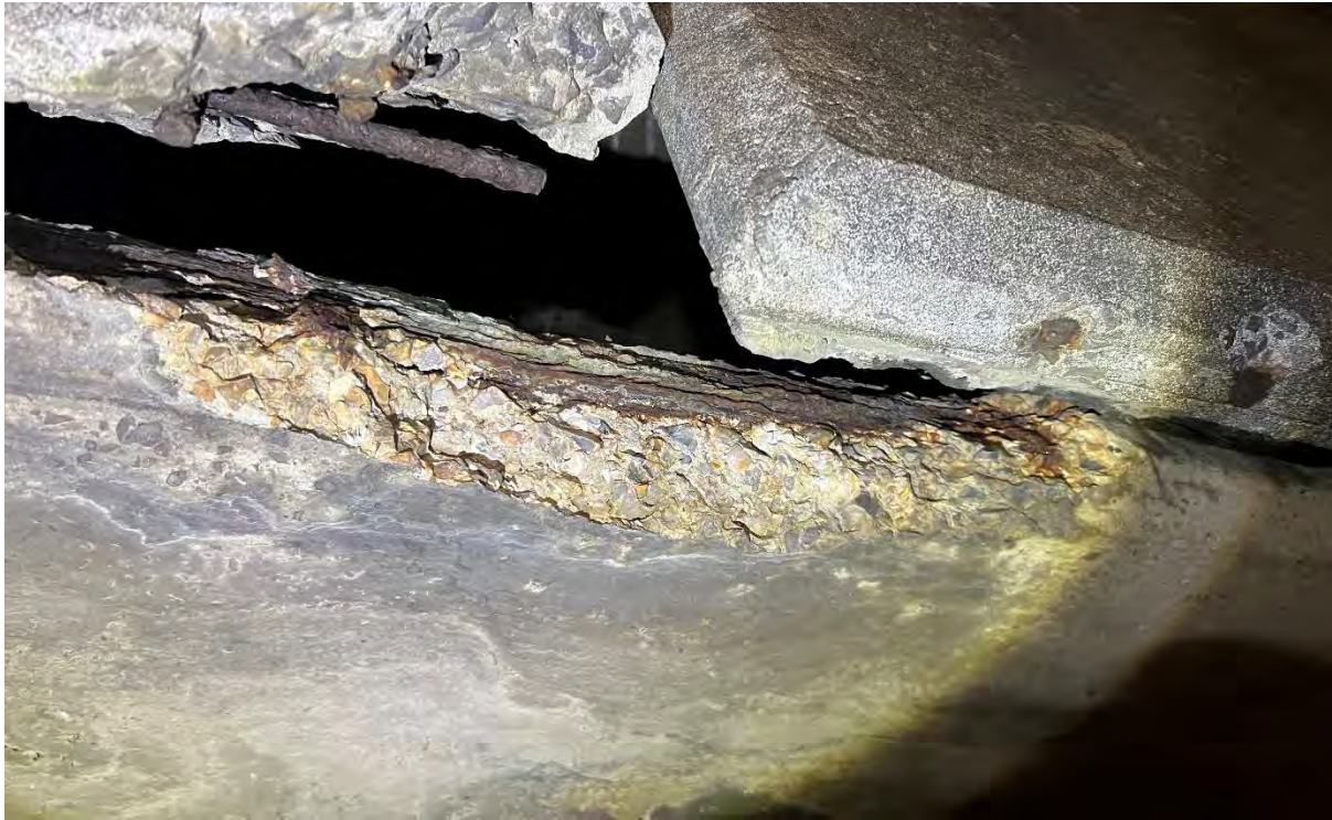
Photograph 9 - Span 2 W/B, beam 1. Area of spalling with exposed reinforcement exhibiting moderate corrosion, measuring 800x80x55mm.
