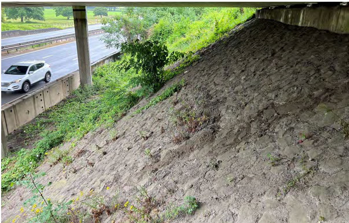
Photograph 84 - Span 1. Moderate vegetation growth to south revetment.
