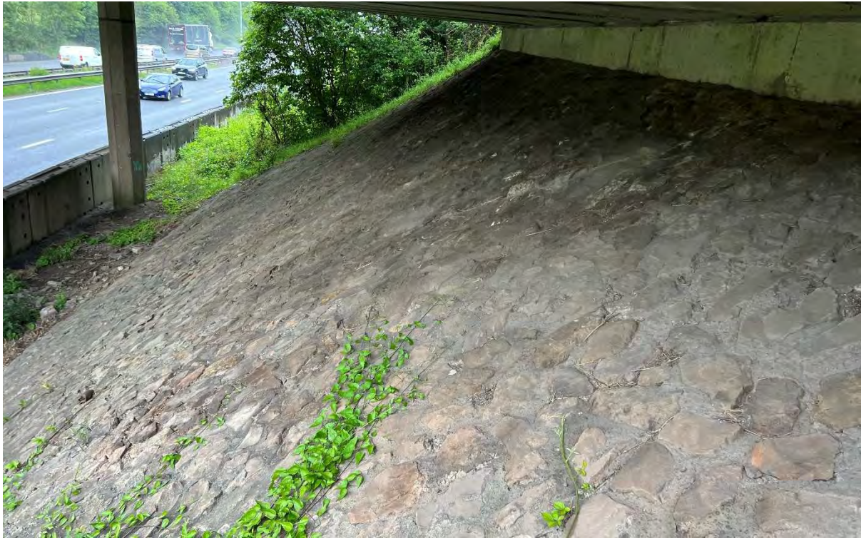
Photograph 85 - Span 3 - Minor vegetation growth to north revetment.
