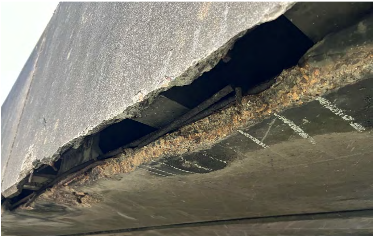
Photograph 22 - Span 2 E/B, beam 1. Area of spalling with exposed reinforcement exhibiting minor corrosion, measuring 3200x60x100mm.
