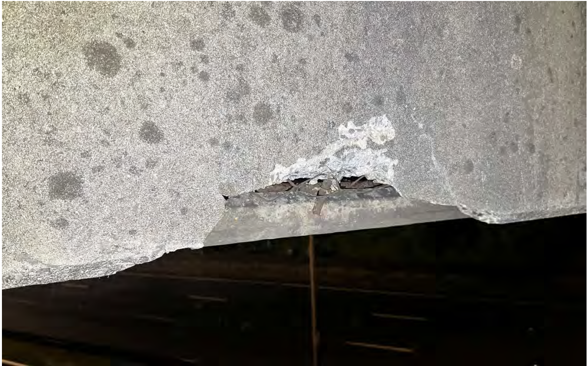
Photograph 53 - Span 2 W/B, east parapet fascia panel. Area of spalling with exposed reinforcement exhibiting minor corrosion, measuring 600x120x75mm.
