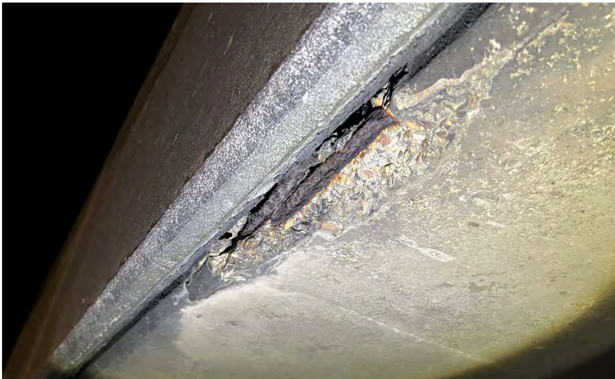
Photograph 10 - Span 2 W/B, beam 1. Area of spalling with exposed reinforcement exhibiting minor corrosion, measuring 500x80x50mm.
