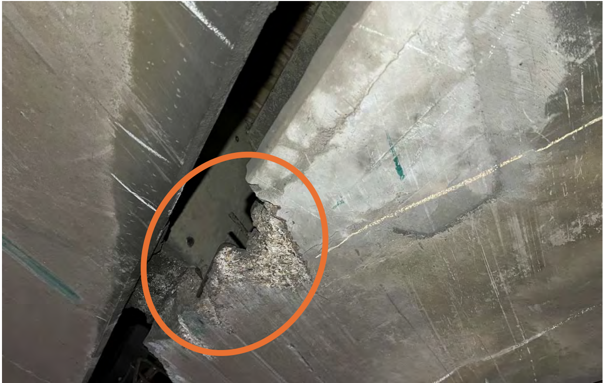
Photograph 29 - Span 2 E/B, beam 3. Area of spalling with exposed reinforcement exhibiting minor corrosion, measuring 900x120x100mm.
