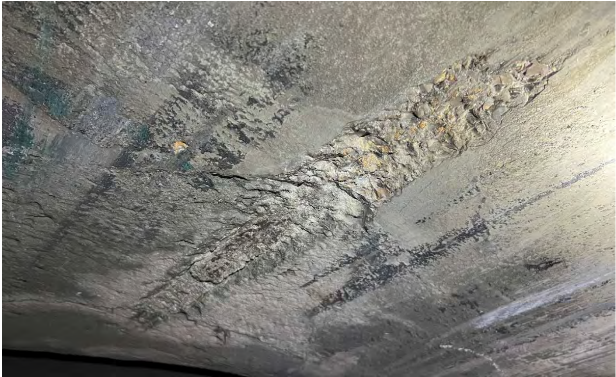
Photograph 39 - Span 2 E/B, beam 6. Area of spalling, measuring 400x100x10mm.
