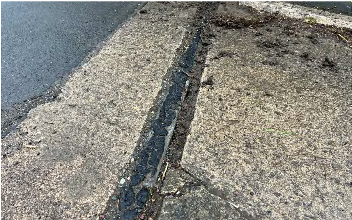
Photograph 74 - Span 1. Build-up of dirt and debris to expansion joint in footways, southwest shown.
