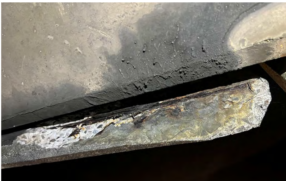
Photograph 56 - Span 2 W/B, west parapet fascia panel. Area of spalling with exposed reinforcement exhibiting minor corrosion, measuring 500x150x35mm.
