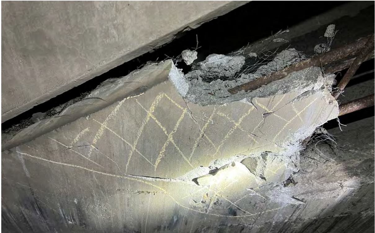
Photograph 42 - Span 2 E/B, beam 7. Area of delamination, measuring 700x500mm.
