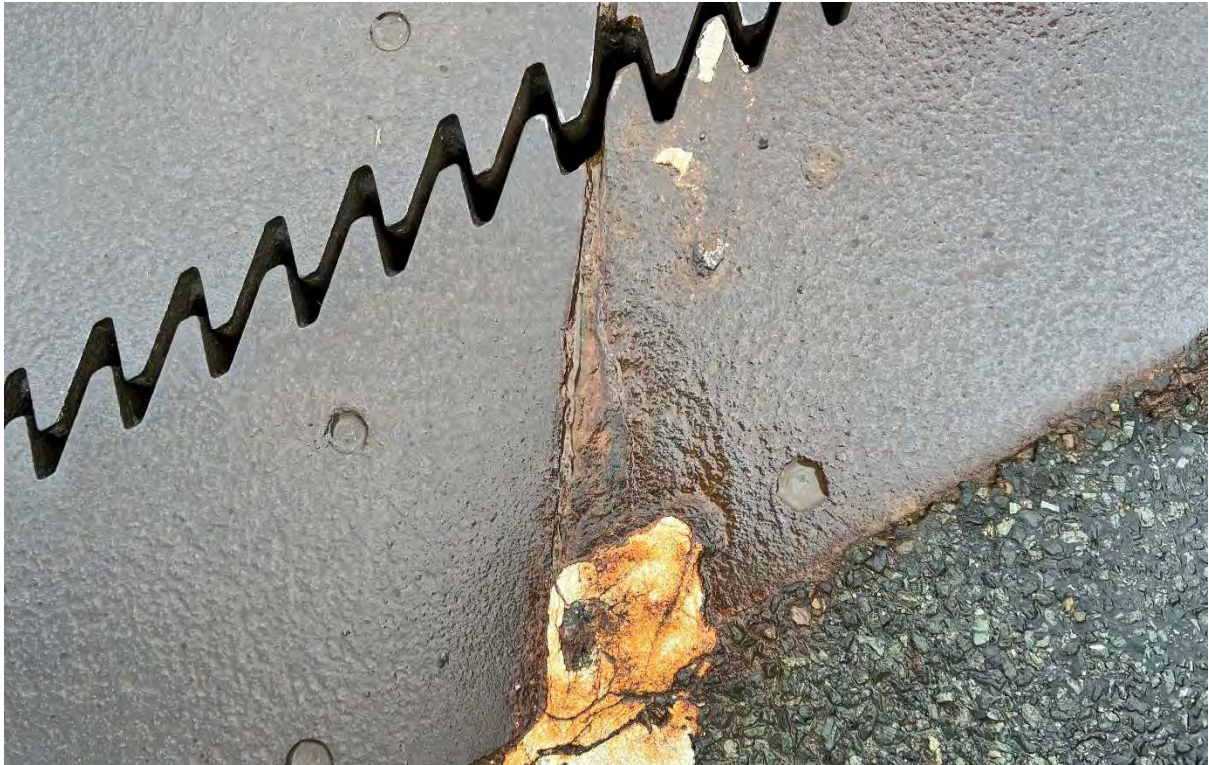
Photograph 73 - Span 1. Isolated minor corrosion to south expansion joint.
