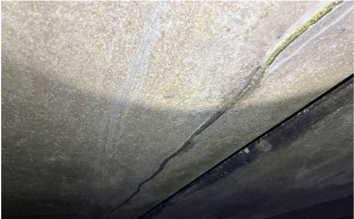
Photograph 51 - Span 3, beam 1. Calcite staining indicating water seepage through the deck.
