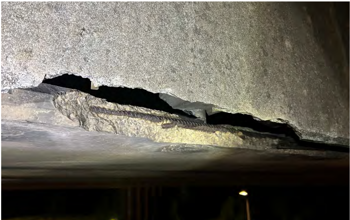
Photograph 18 - Span 2, W/B, beam 9. Area of spalling with exposed reinforcement exhibiting minor corrosion, measuring 2000x80x55mm.
