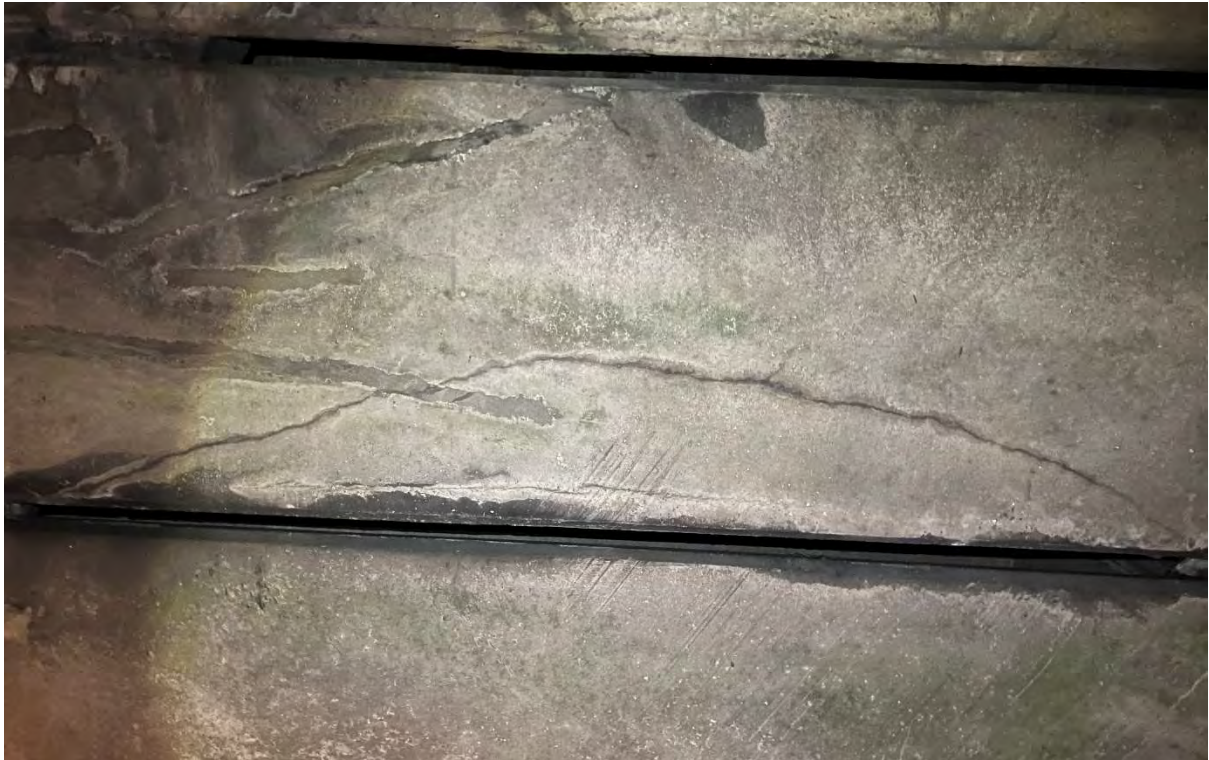
Photograph 15 – Span 2 W/B, beam 8. Longitudinal crack to deck soffit, 1200mm in length and up to 0.2mm in width.
