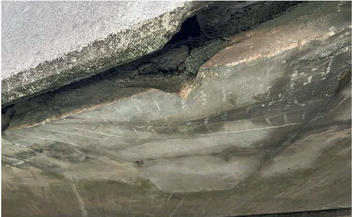
Photograph 23 - Span 2 E/B, beam 1. Area of delamination, measuring 800x150mm.
