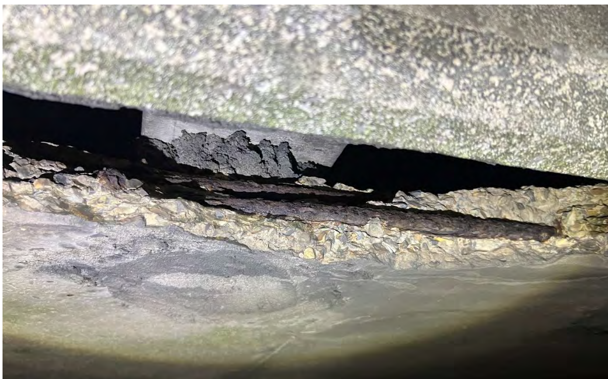
Photograph 20 - Span 2 W/B, beam 9. Area of spalling with exposed reinforcement exhibiting minor corrosion, measuring 700x80x50mm.
