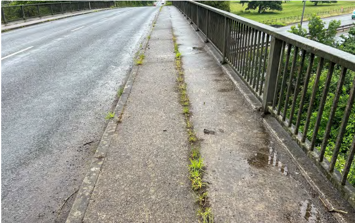
Photograph 83 - Vegetation growth and cracking to footway surfacing.
