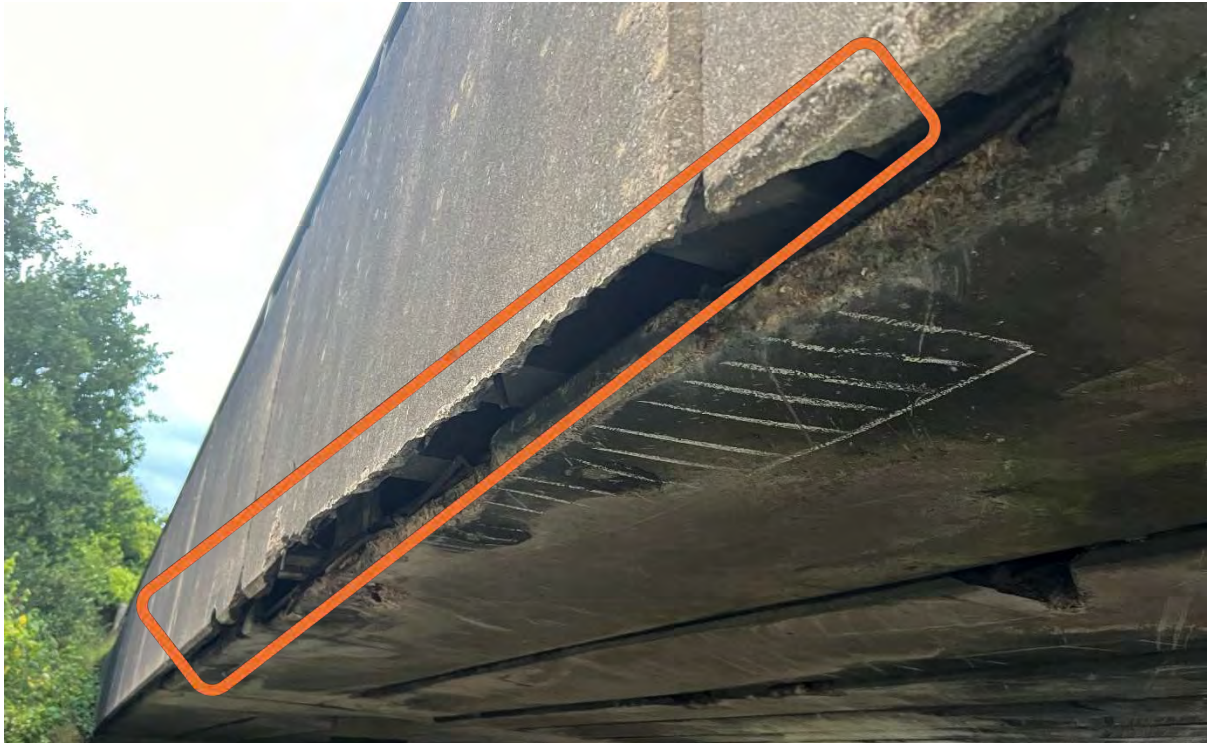
Photograph 59 - Span 2 E/B, west parapet fascia panel. Three areas of spalling exposing reinforcement exhibiting minor corrosion, measuring 1200x100x75mm, 2500x100x75mm, and 300x75x75mm.
