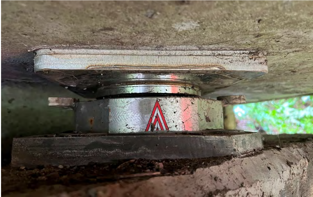
Photograph 68 - Span 1, south abutment. Isolated surface corrosion to bearings.
