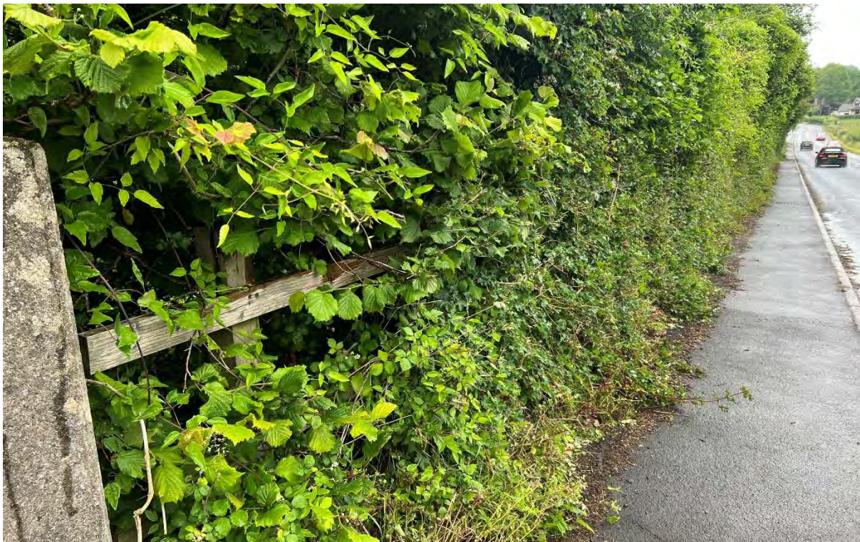
Photograph 86 - Dense vegetation growth to spans 1 & 3 approach fencing.
