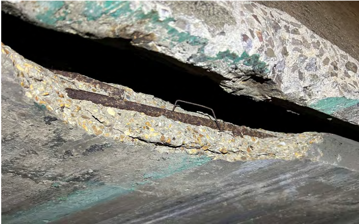
Photograph 47 - Span 2 E/B, beam 9. Area of spalling with exposed reinforcement exhibiting minor corrosion, measuring 500x200x100mm.
