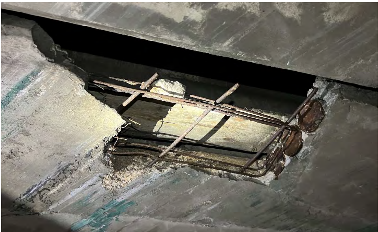
Photograph 44 - Span 2 E/B, beam 9. Area of spalling with exposed reinforcement exhibiting minor corrosion, measuring 900x500x100mm.
