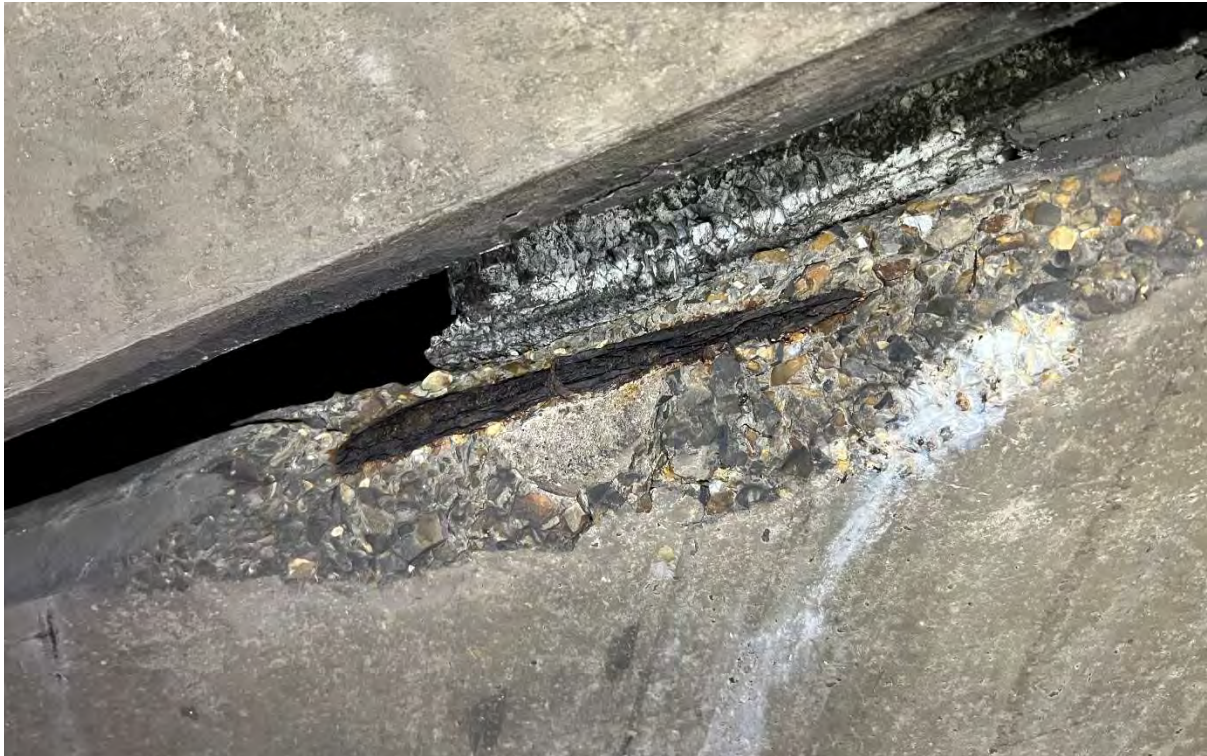
Photograph 33 - Span 2 E/B, beam 4. Area of spalling with exposed reinforcement exhibiting minor corrosion, measuring 400x40x75mm.
