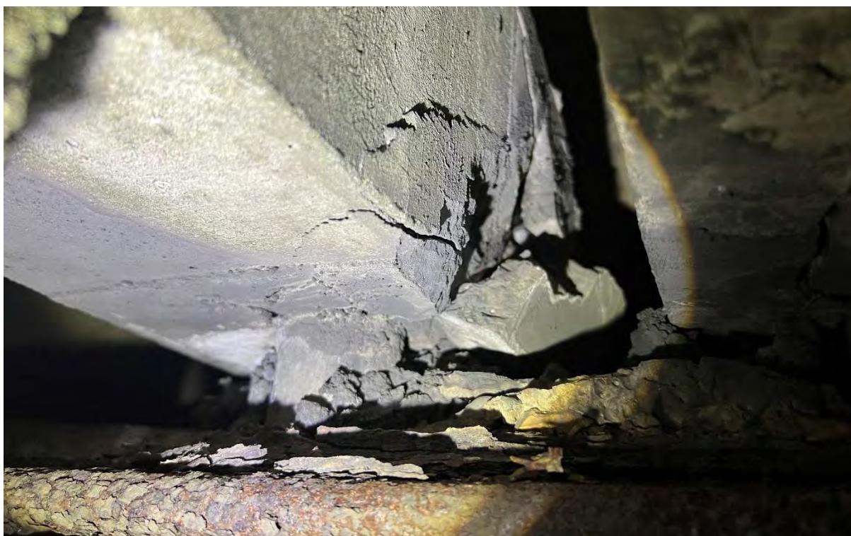
Photograph 19 - Span 2 W/B, beam 9. Area of spalling and loose concrete to edge unit connection.
