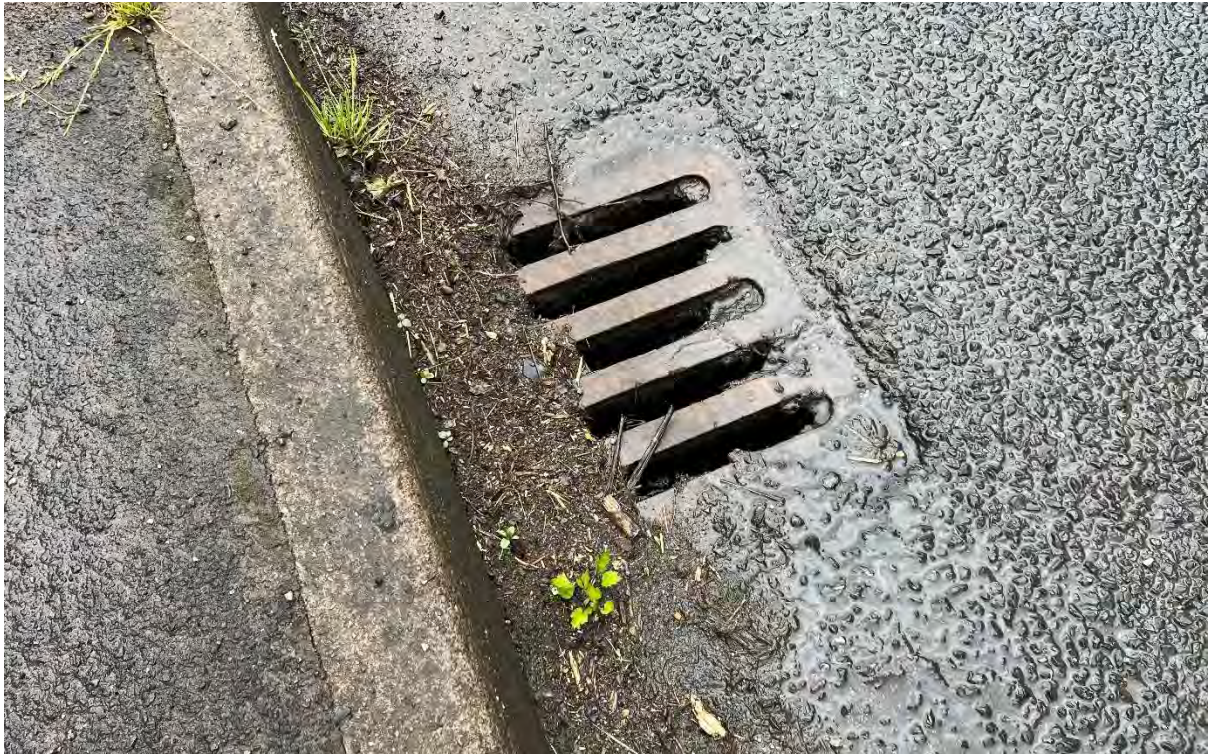
Photograph 71 – Drainage gully partially blocked by vegetation and debris.
