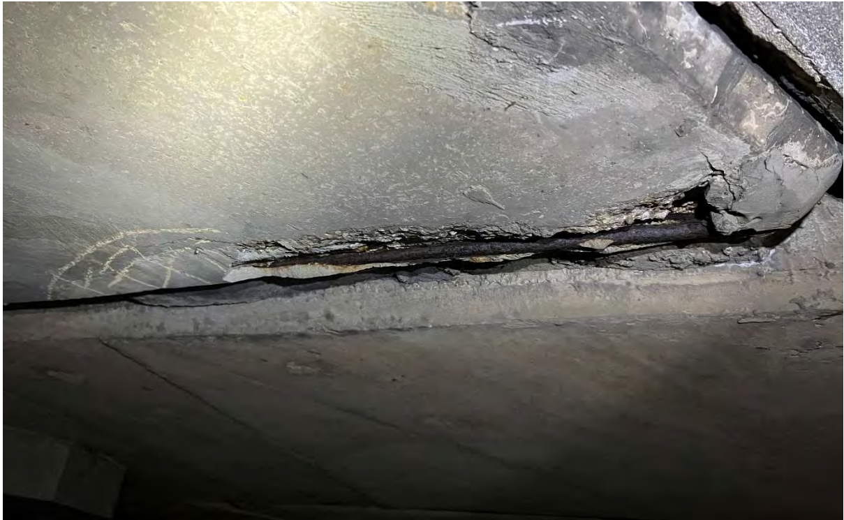
Photograph 49 - Span 2 E/B, beam 9. Area of delamination & spalling with exposed reinforcement exhibiting minor corrosion, measuring 1800x200x40mm.
