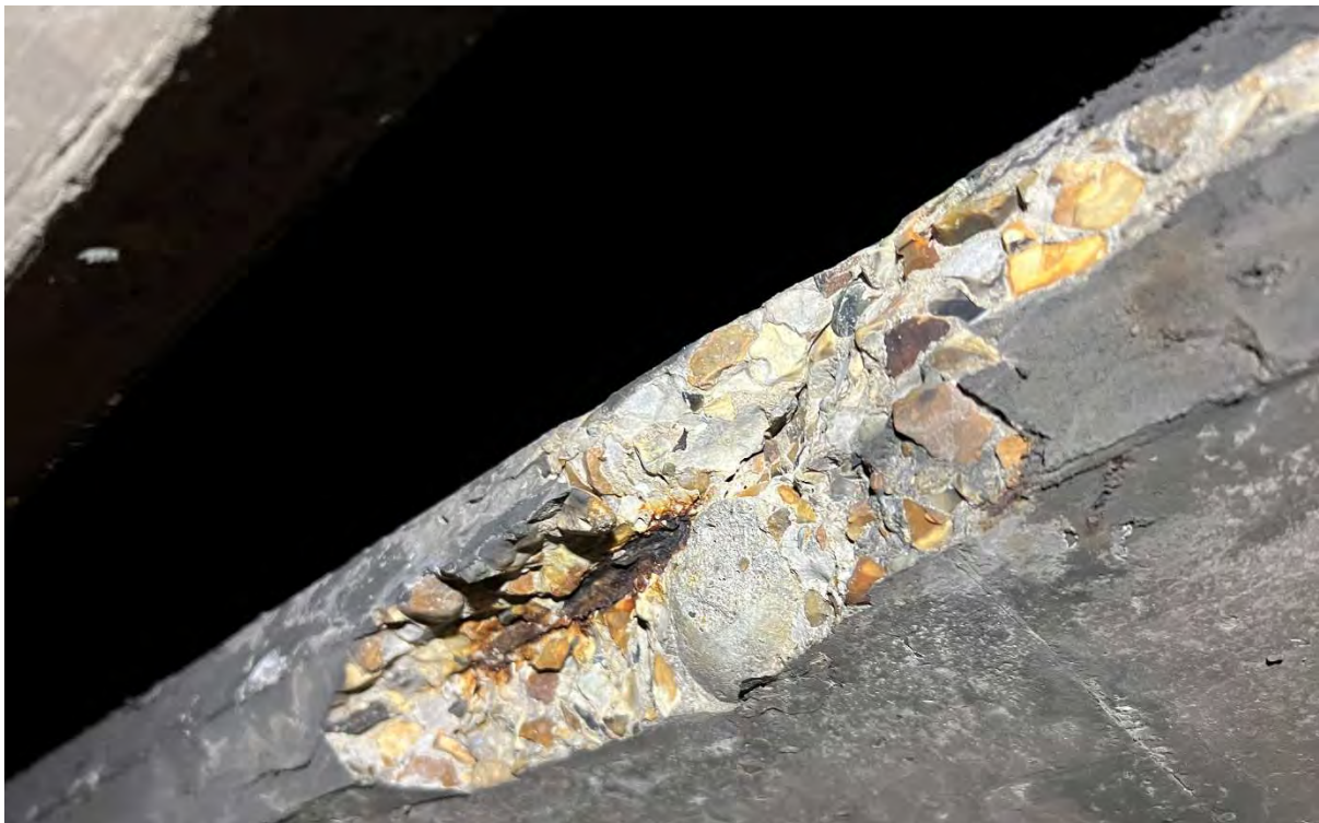
Photograph 12 - Span 2 W/B, beam 5. Area of spalling with exposed reinforcement exhibiting minor corrosion, measuring 200x60x35mm.
