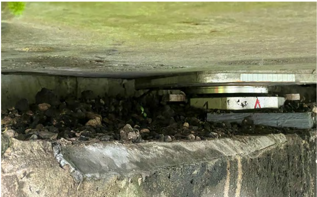
Photograph 70 - Span 1. Build-up of dirt and debris to south bearing shelf.
