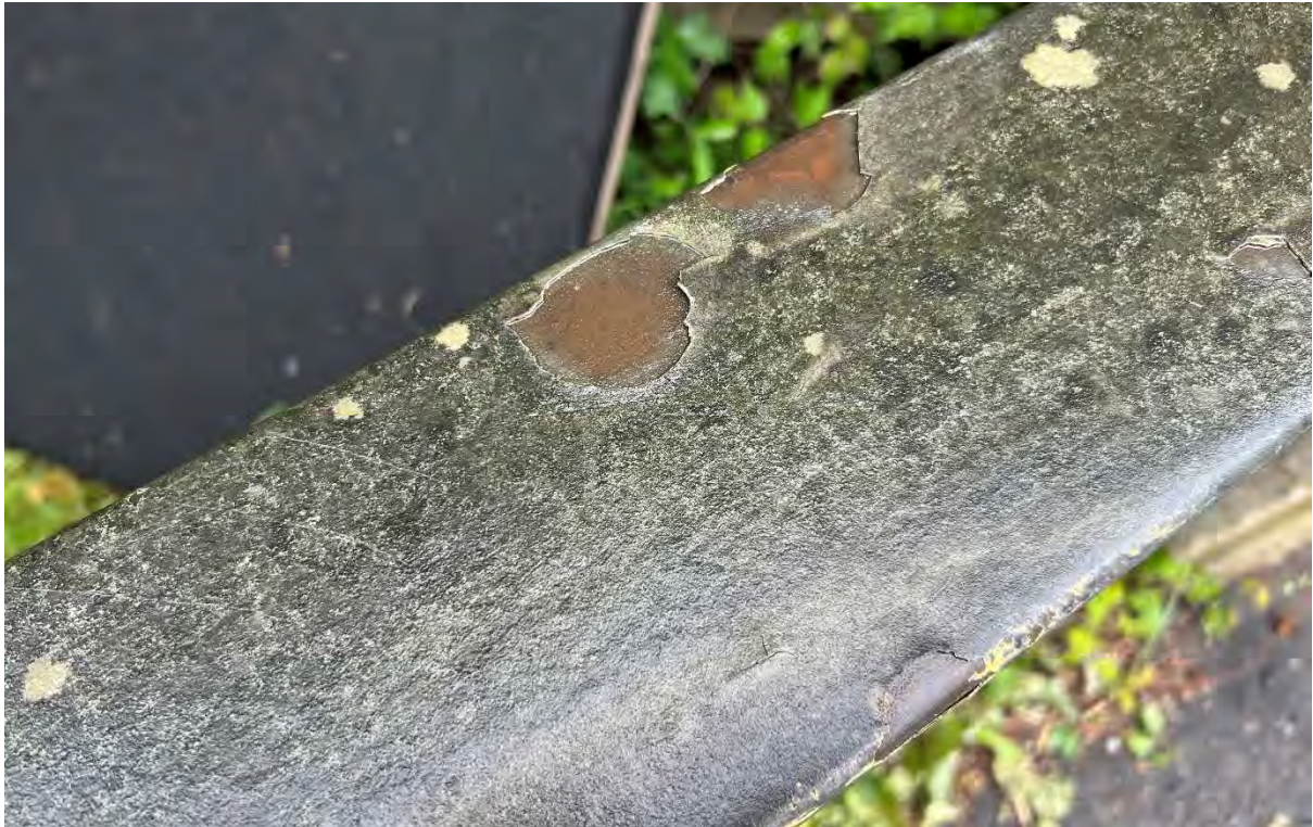
Photograph 77 - Isolated minor corrosion to parapet rails where the paint system had failed.
