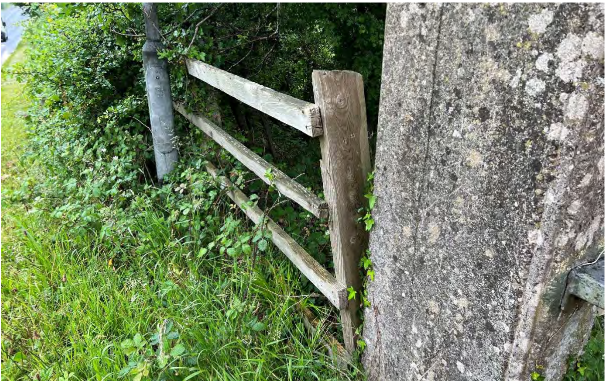
Photograph 88 - Span 3. Moderate timber decay to northeast approach fencing.
