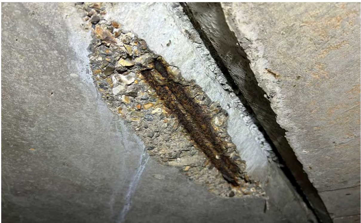
Photograph 50 - Span 3, beam 1. Area of spalling with exposed reinforcement exhibiting minor corrosion, measuring 500x120x30mm.
