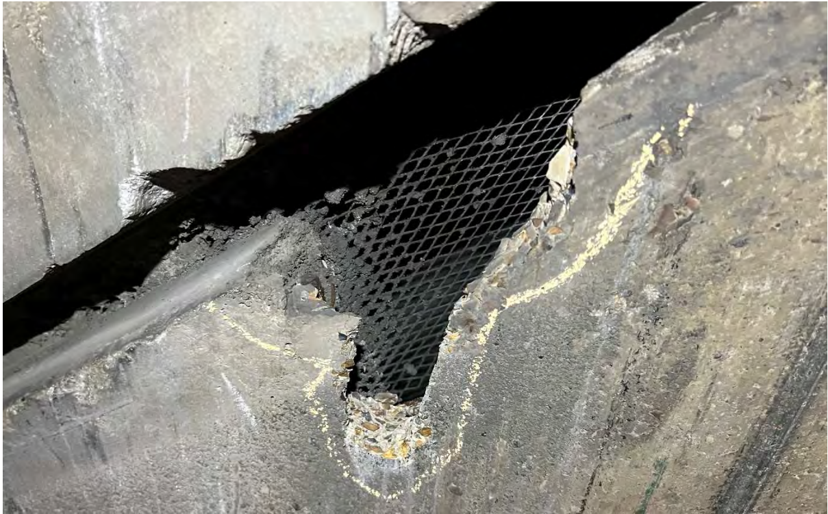
Photograph 37 - Span 2 E/B, beam 5. Area of spalling, measuring 300x400x100mm.
