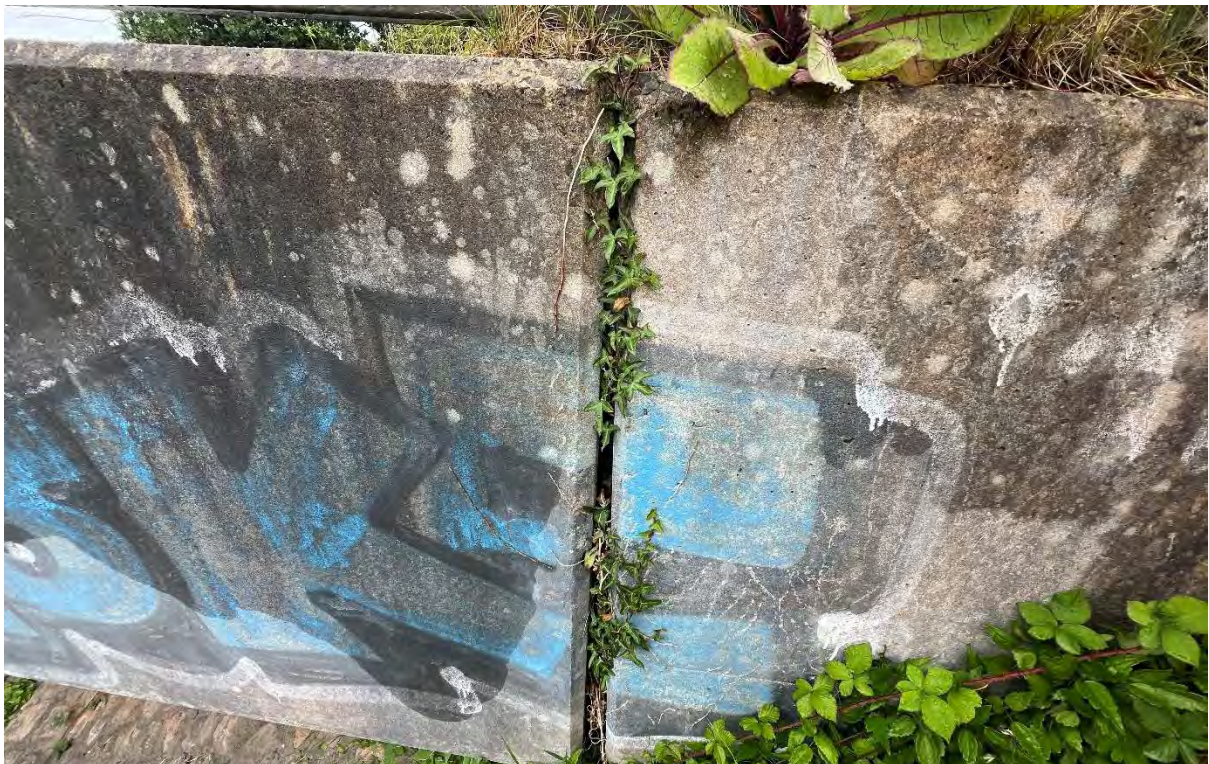
Photograph 76 - Span 3. Vegetation growth to joint between parapet panel and northeast wing wall.
