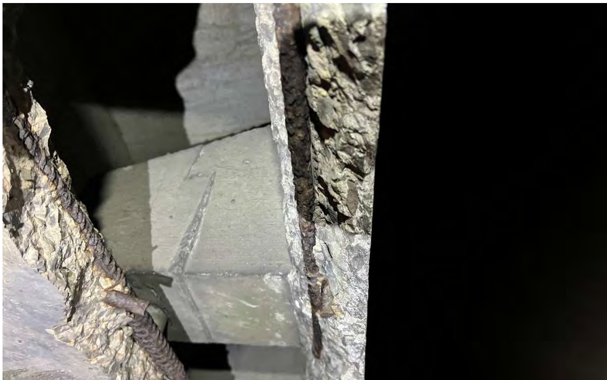
Photograph 55 - Span 2 W/B, east parapet fascia panel. Area of spalling with exposed reinforcement exhibiting minor corrosion, measuring 700x50x75mm.
