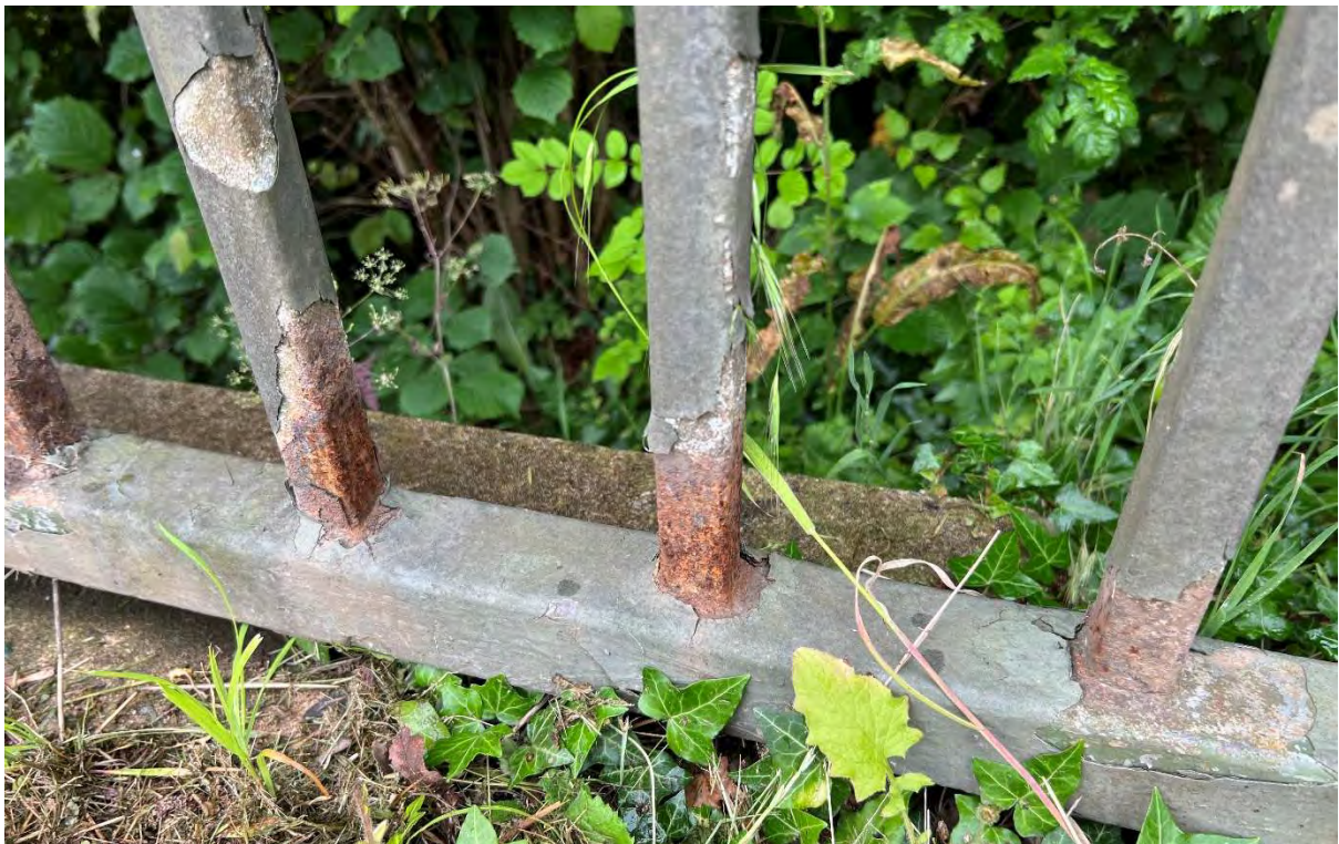
Photograph 80 - Span 1. Minor surface corrosion to southeast parapet infill bars.
