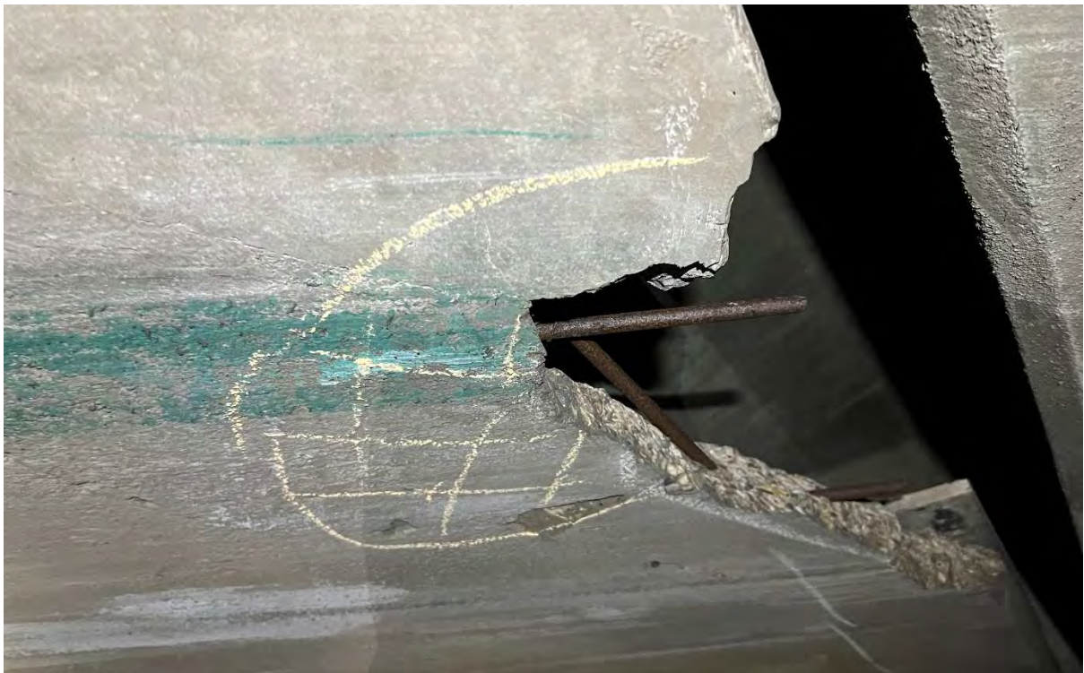
Photograph 40 - Span 2 E/B, beam 7. Area of spalling (700x200x100mm) & delamination (200x300mm) with exposed reinforcement exhibiting minor corrosion.
