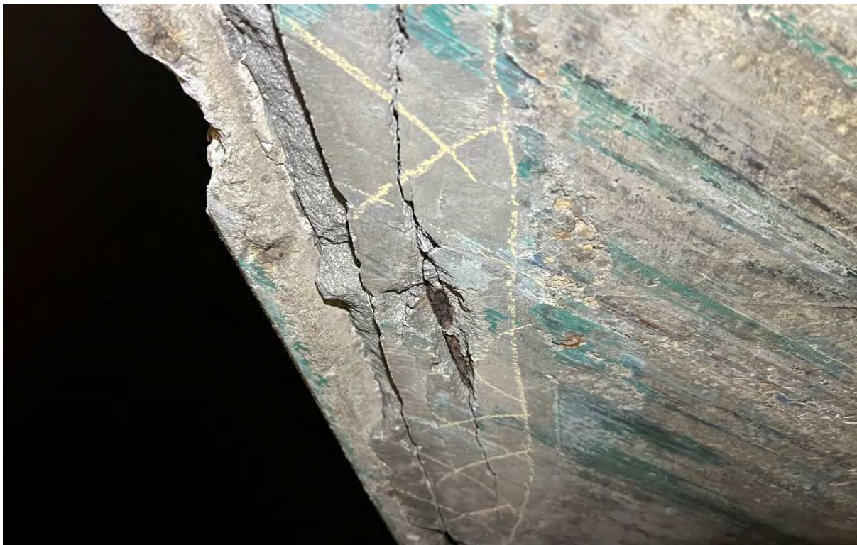
Photograph 48 - Span 2 E/B, beam 9. Area of delamination & spalling with exposed reinforcement exhibiting minor corrosion, measuring 2000x200x40mm.
