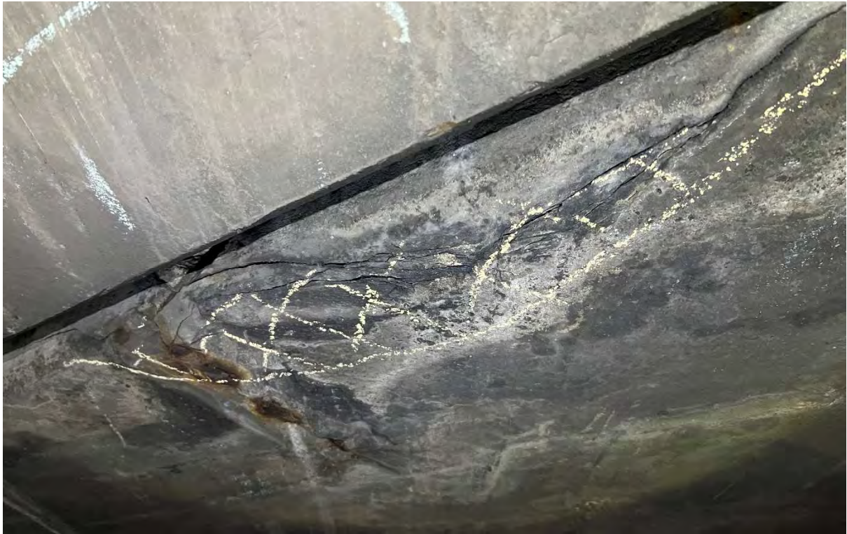
Photograph 43 - Span 2 E/B, beam 8. Area of delamination, measuring 800x200mm.
