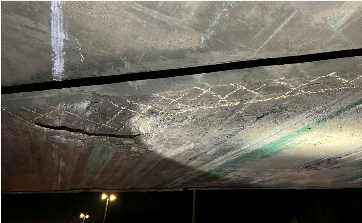
Photograph 45 - Span 2 E/B, beam 9. Area of spalling (400x200x35mm) and delamination (1100x250mm).
