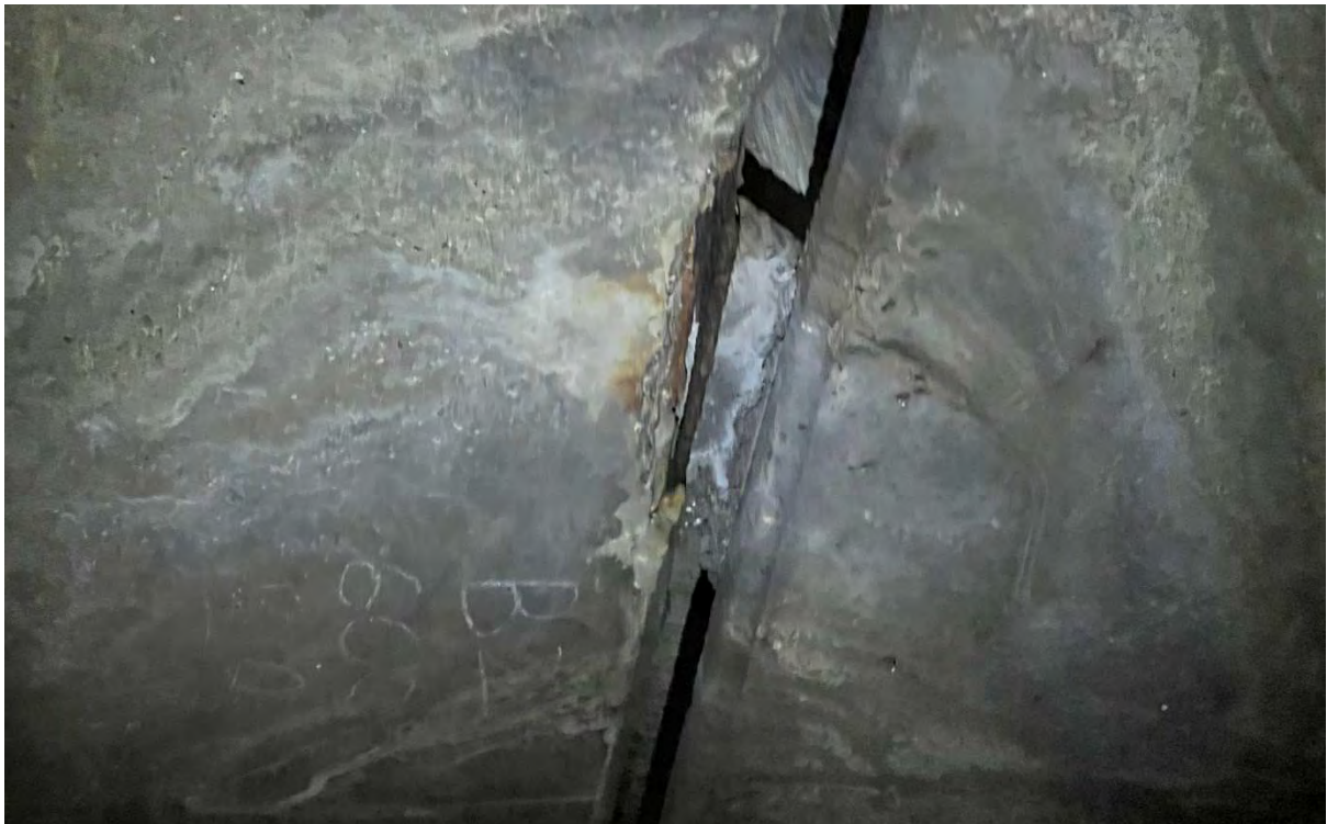
Photograph 16 - Span 2 W/B, beam 8. Area of spalling with exposed reinforcement exhibiting minor corrosion, measuring 500x80x35mm.
