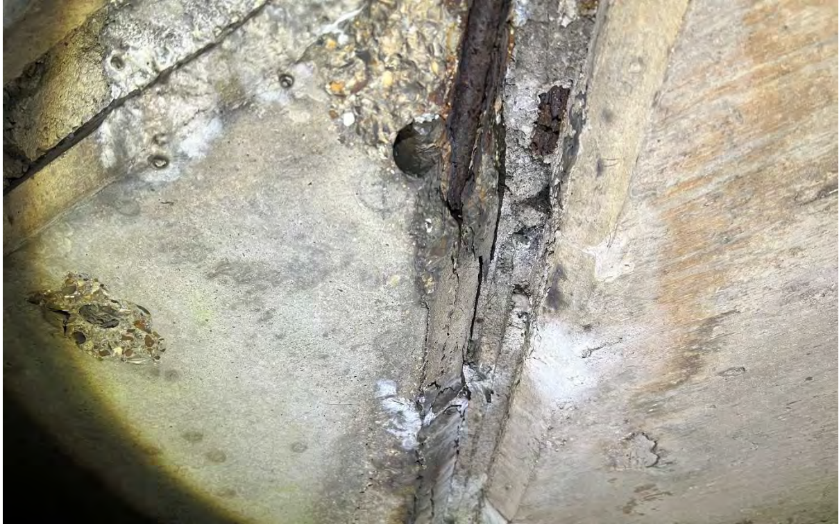
Photograph 7 - Span 1, beam 8. Area of spalling with exposed reinforcement exhibiting minor corrosion and delamination, measuring 1200x100x30mm.
