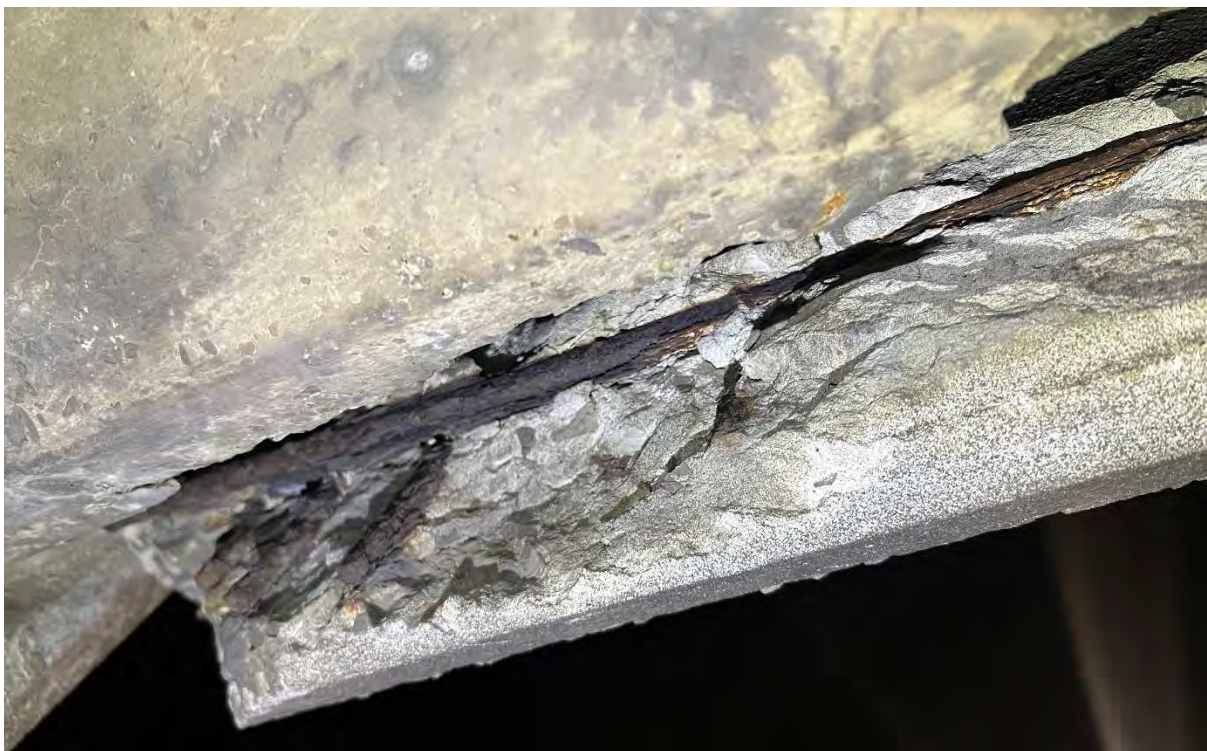
Photograph 58 - Span 2 W/B, west parapet fascia panel. Area of spalling with exposed reinforcement exhibiting minor corrosion, measuring 2600x300x20mm.
