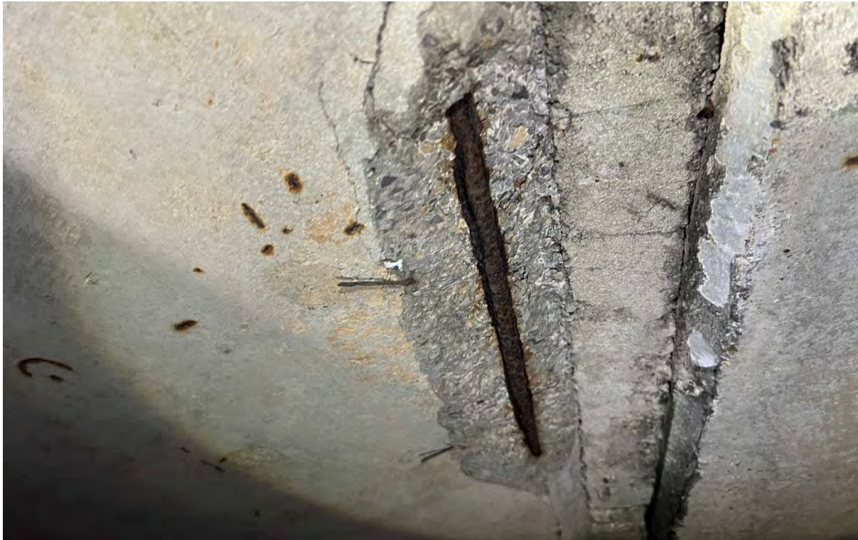
Photograph 67 - Span 2, north crosshead. Area of spalling with exposed reinforcement exhibiting minor corrosion, measuring 600x100x30mm.
