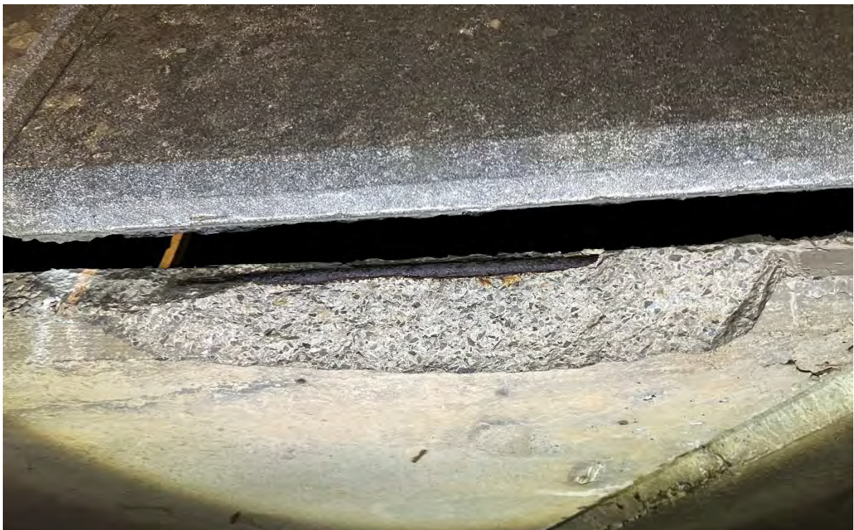
Photograph 66 - Span 1, west edge of south crosshead. Area of spalling with exposed reinforcement exhibiting minor corrosion, measuring 650x150x80mm.
