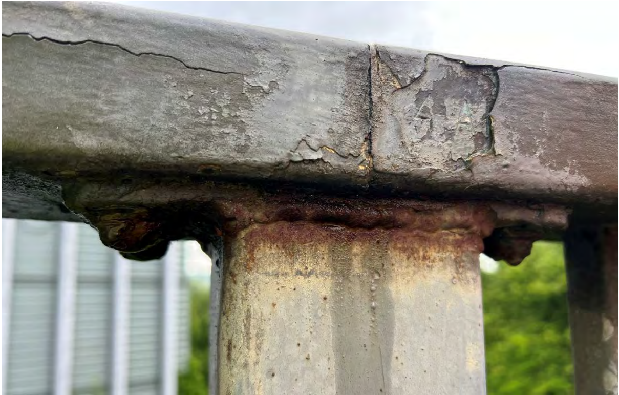
Photograph 79 - Isolated minor corrosion to parapet welded connections.
