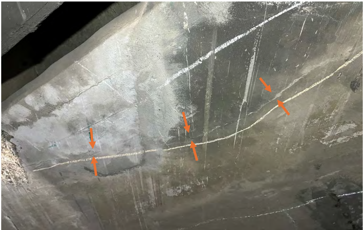
Photograph 28 - Span 2 E/B, beam 3. Longitudinal crack, measuring 1700mm in width and up to 0.2mm in width.
