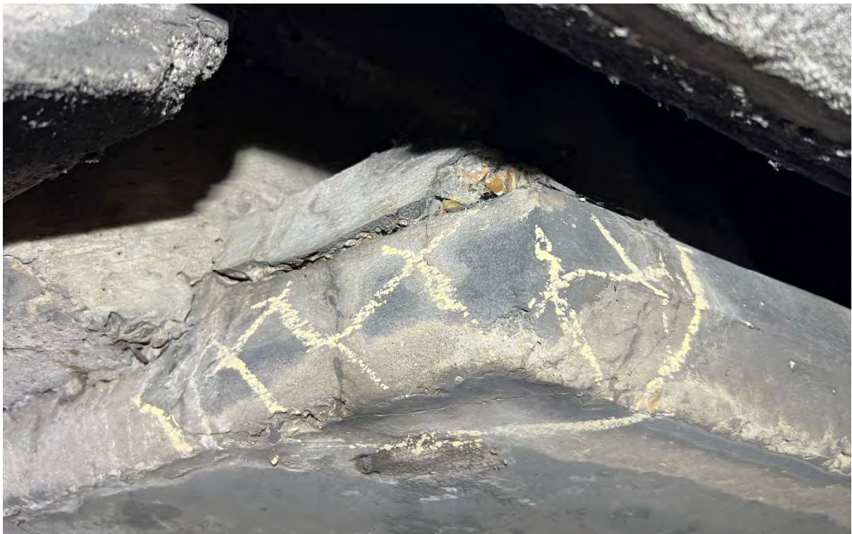
Photograph 24 - Span 2 E/B, beam 1. Area of delamination to end of beam, measuring 200x150mm.
