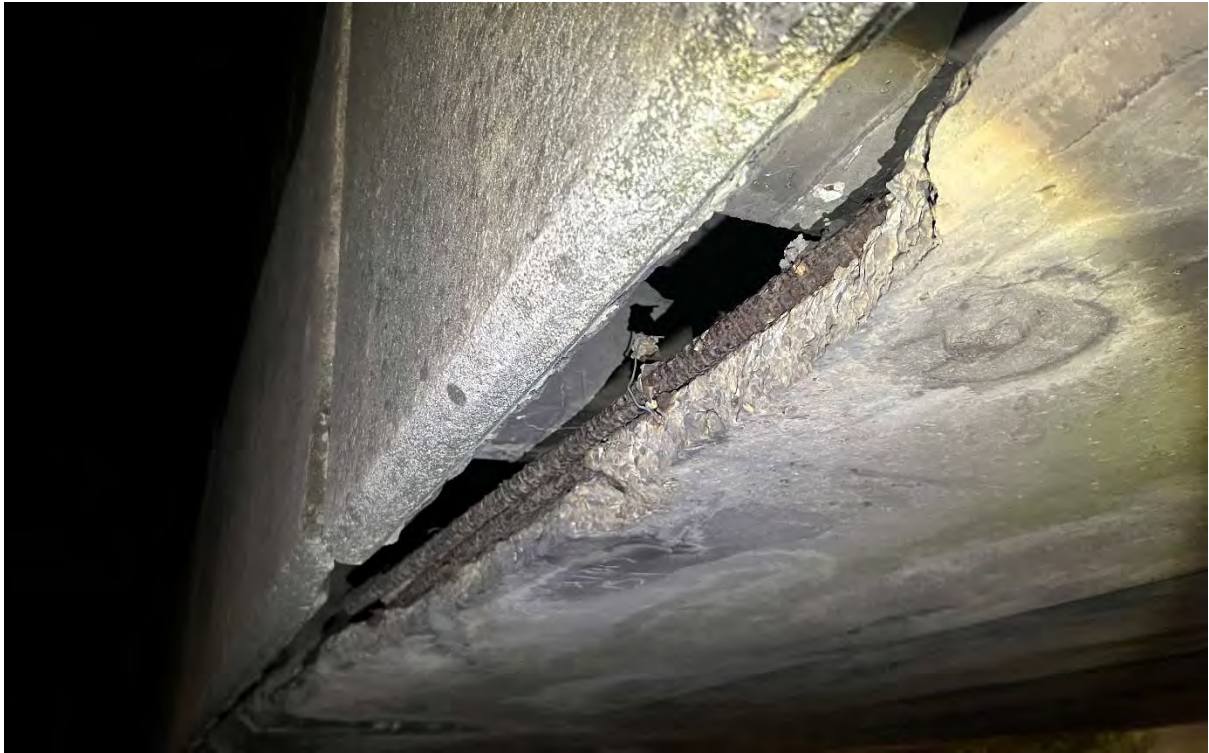
Photograph 17 - Span 2 W/B, beam 9. Area of spalling with exposed reinforcement exhibiting minor corrosion, measuring 2500x80x100mm.
