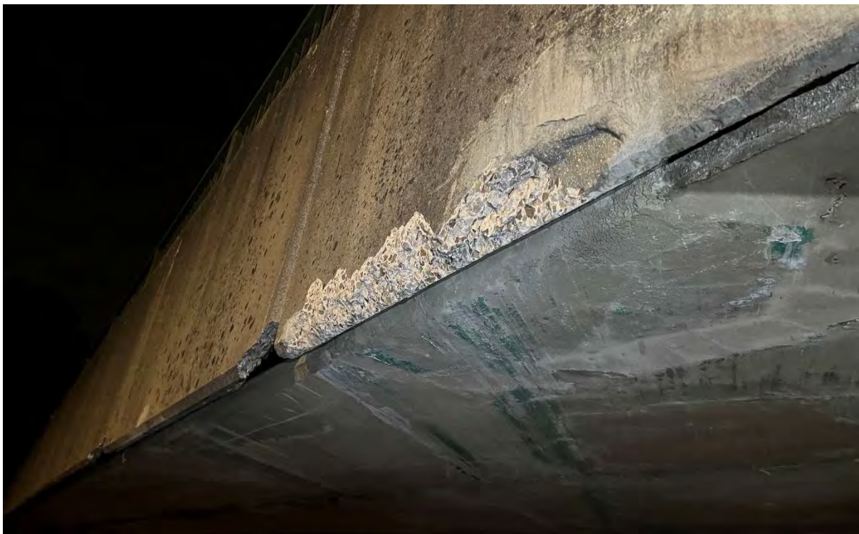
Photograph 60 - Span 2 E/B, east parapet fascia panel. Area of spalling measuring 1100x150x20mm.
