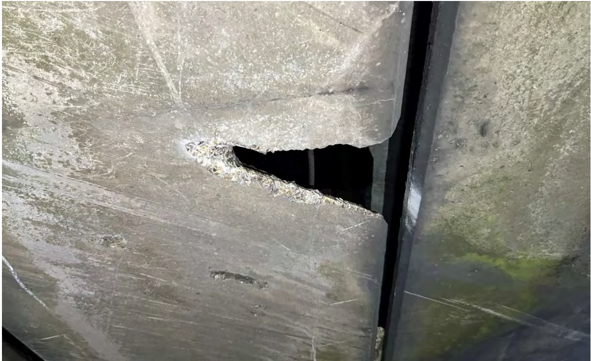
Photograph 27 - Span 2 E/B, beam 2. Area of spalling with exposed reinforcement exhibiting minor corrosion, measuring 500x300x100mm.
