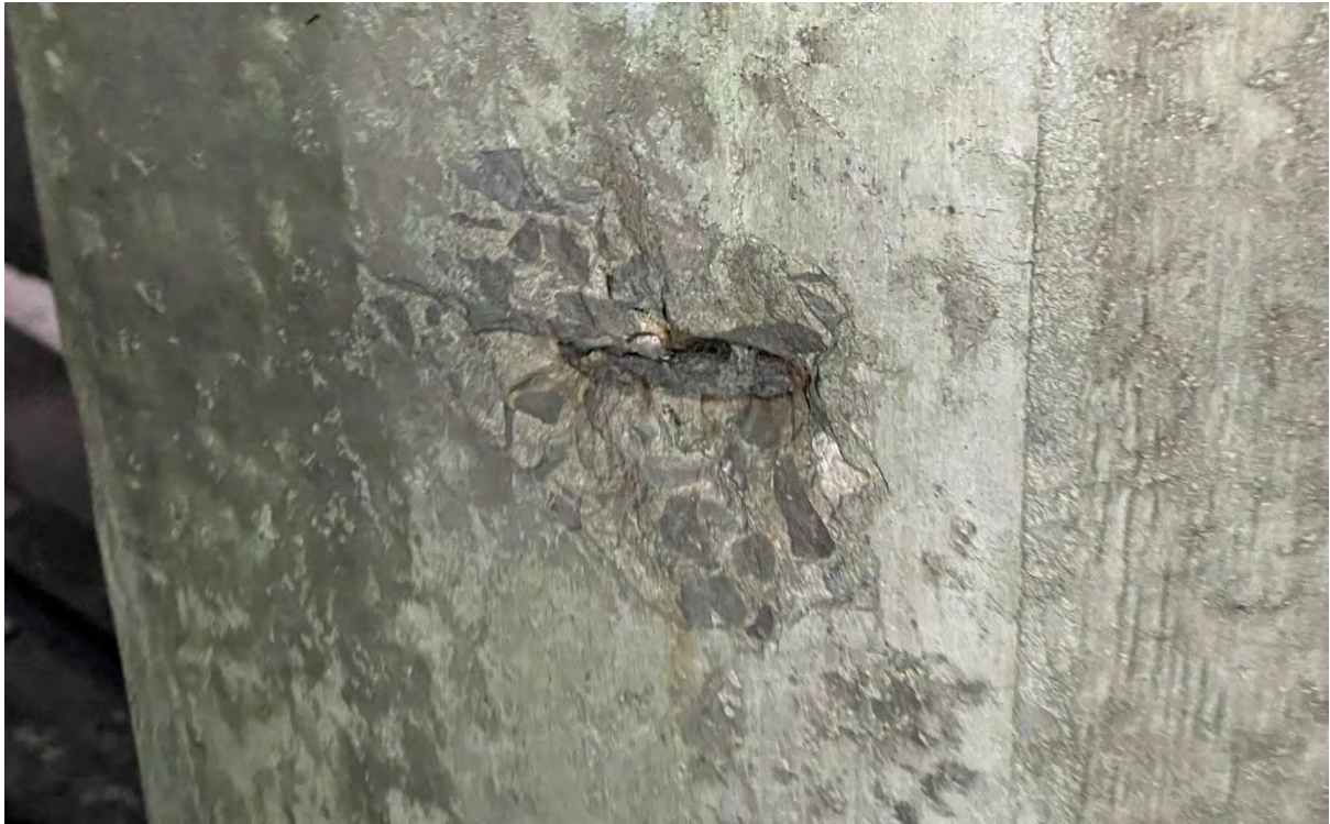
Photograph 65 – Span 2, northeast column. Minor spall with exposed reinforcement exhibiting minor corrosion, measuring 200x200x25mm.
