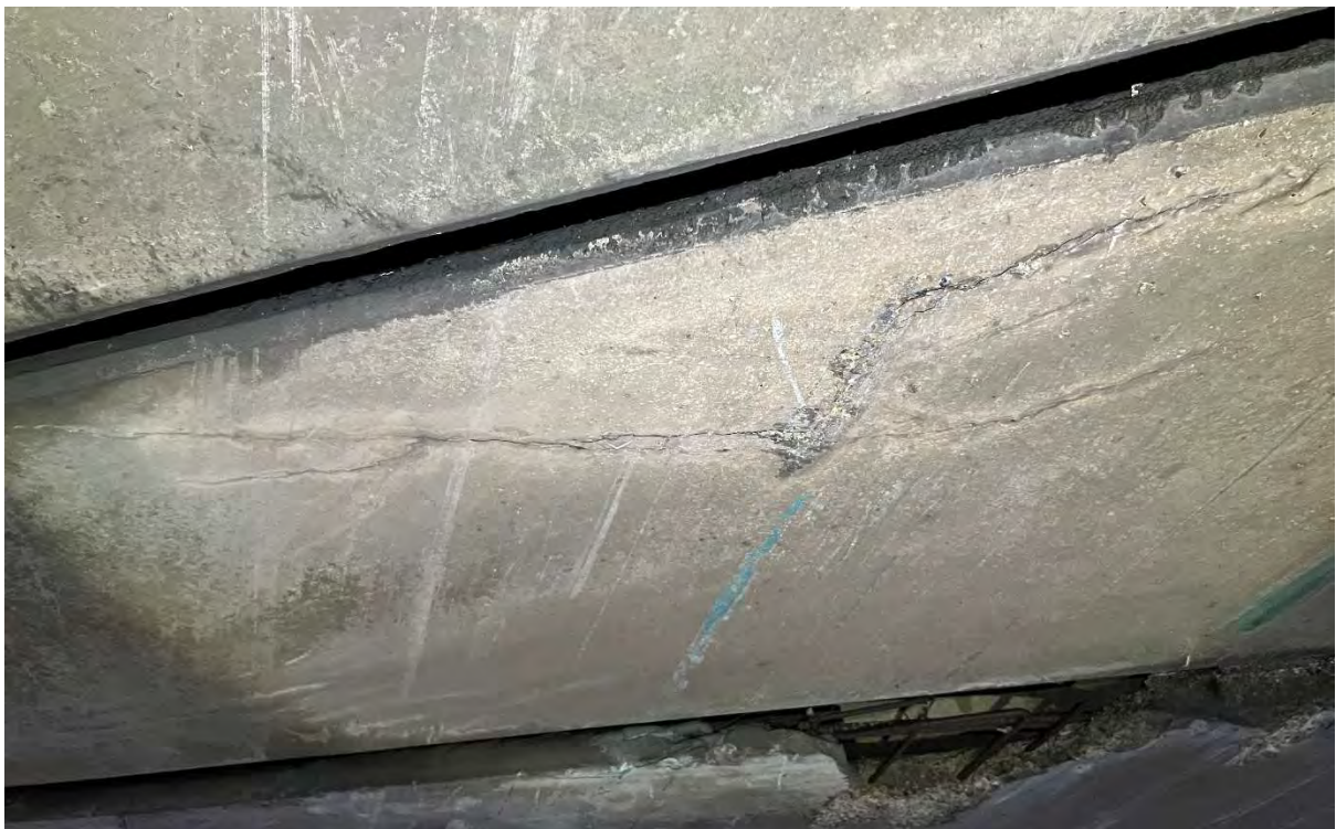
Photograph 26 - Span 2 E/B, beam 2. Longitudinal crack to beam soffit, measuring 2500mm in length and up to 0.9mm in width.
