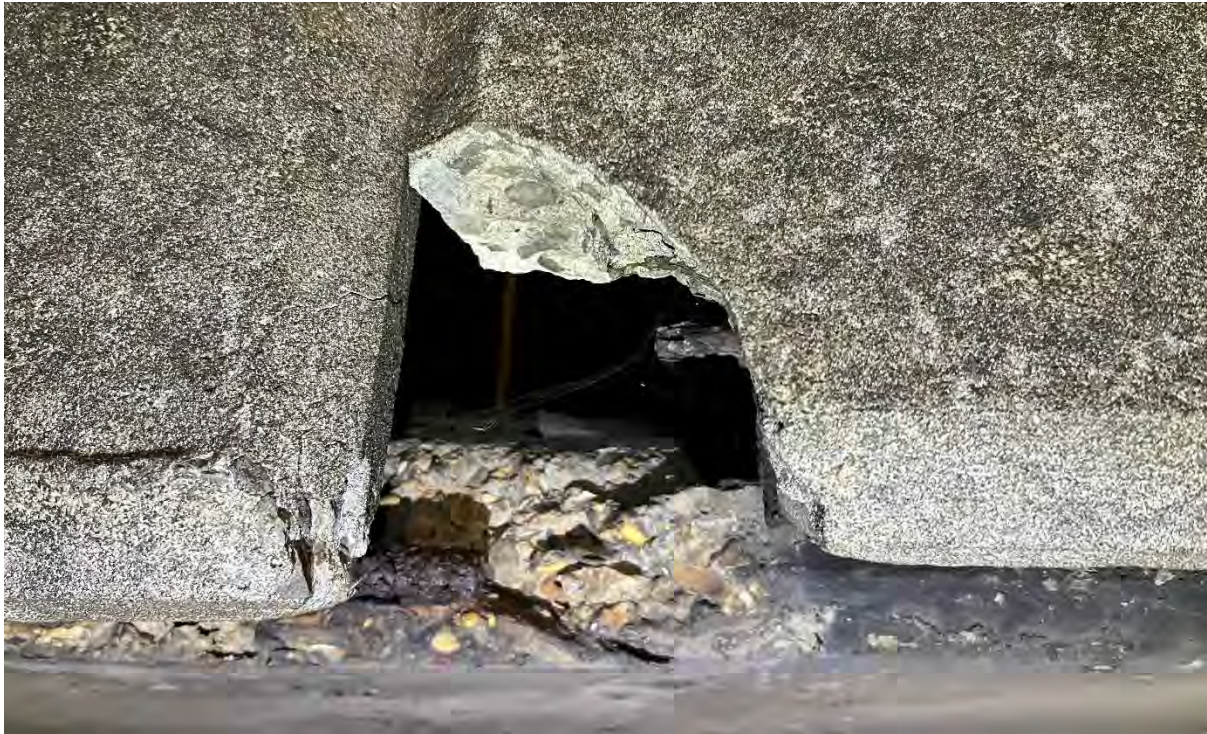
Photograph 57 - Span 2 W/B, west parapet fascia panel. Area of spalling with exposed reinforcement exhibiting minor corrosion, measuring 100x120x75mm.
