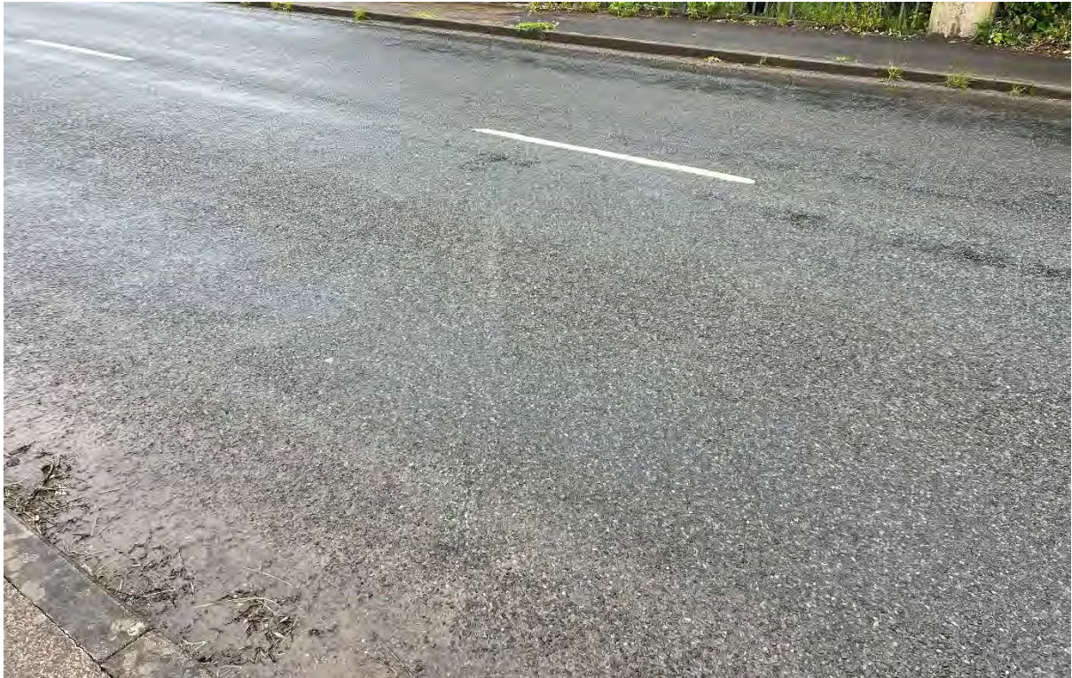
Photograph 75 - Span 3. No crack inducer to north expansion joint.
