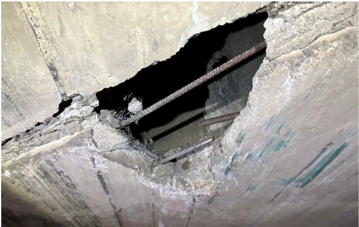
Photograph 38 - Span 2 E/B, beam 6. Area of spalling with exposed reinforcement exhibiting minor corrosion, measuring 300x400x100mm.
