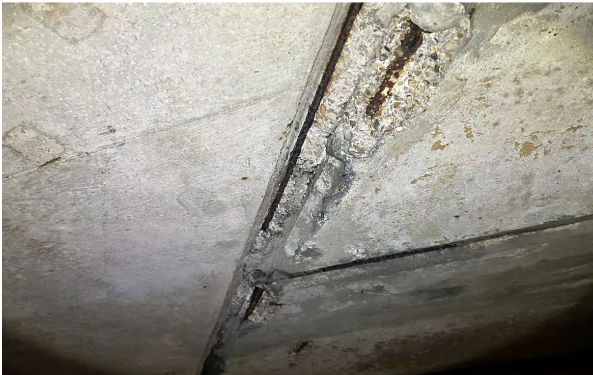
Photograph 14 - Span 2 W/B, beam 6. Sporadic areas of spalled concrete with exposed reinforcement exhibiting minor corrosion between the beam & crosshead.
