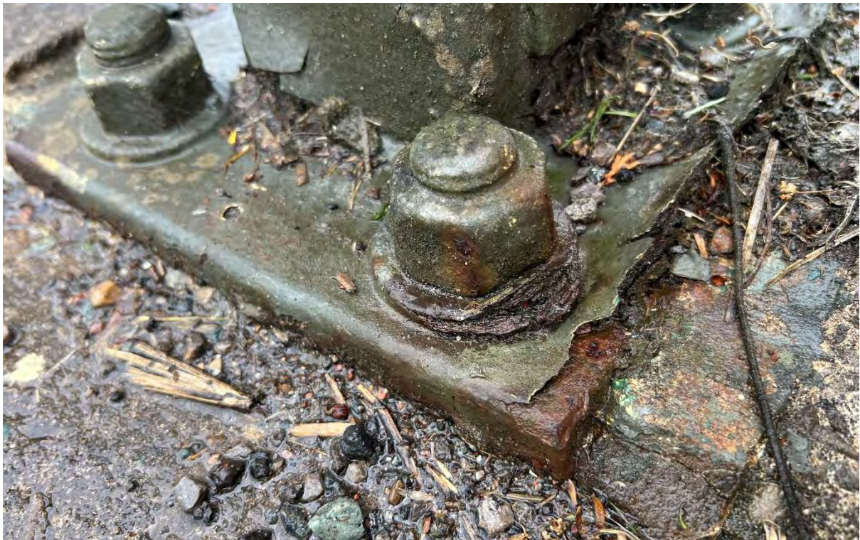
Photograph 78 - Isolated minor corrosion to parapet base plates and holding down bolts.
