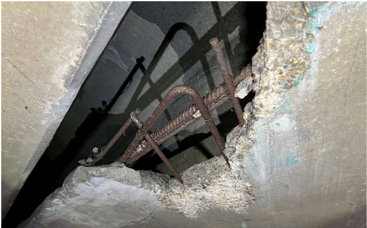
Photograph 30 - Span 2 E/B, beam 3. Area of spalling with exposed reinforcement exhibiting minor corrosion, measuring 700x600x100mm.
