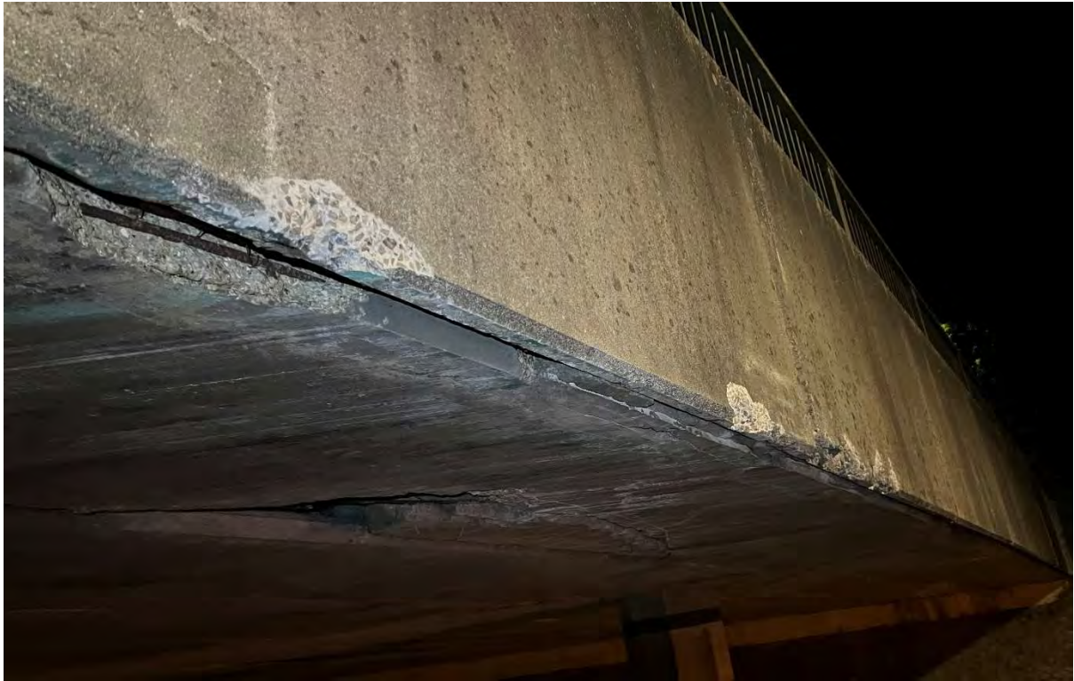
Photograph 61 - Span 2 E/B, east parapet fascia panel. Three minor spalls, all measuring 200x100x20mm.
