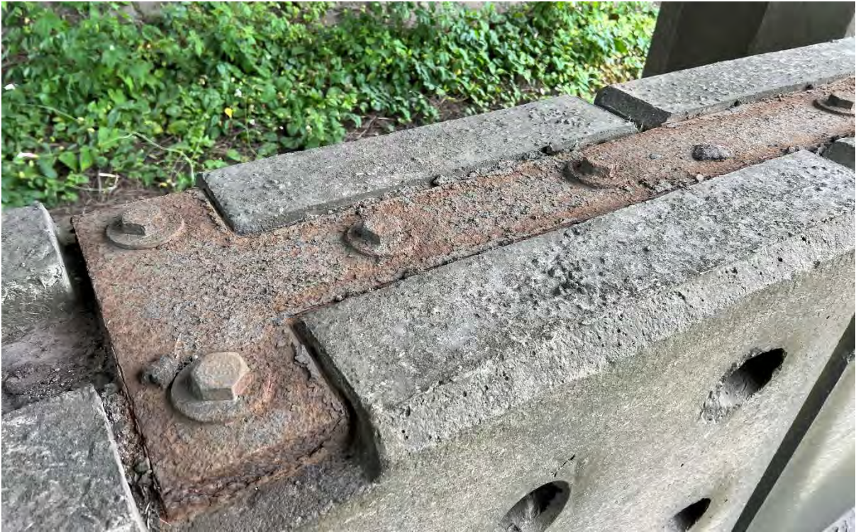
Photograph 87 - Span 2. Minor surface corrosion to the TVCB connections.
