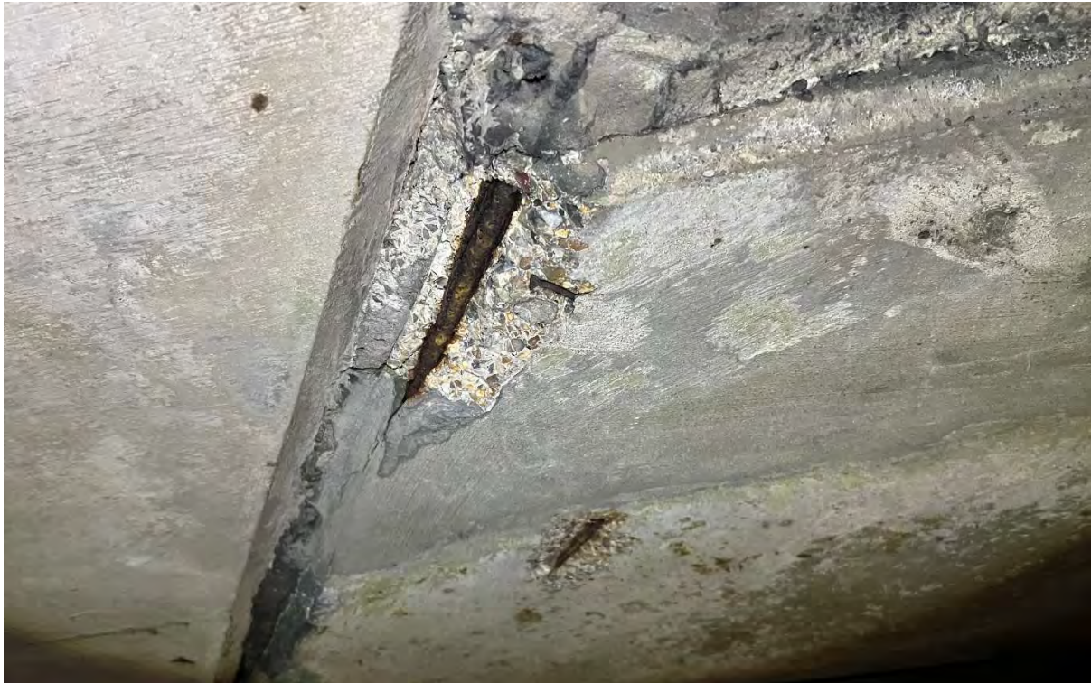
Photograph 13 - Span 2 W/B, beam 5. Sporadic areas of spalled concrete with exposed reinforcement exhibiting minor corrosion to the beam soffit.
