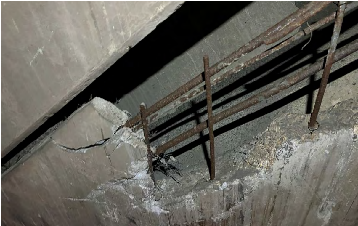
Photograph 41 - Span 2 E/B, beam 7. Area of spalling with exposed reinforcement exhibiting minor corrosion, measuring 1200x450x100mm.
