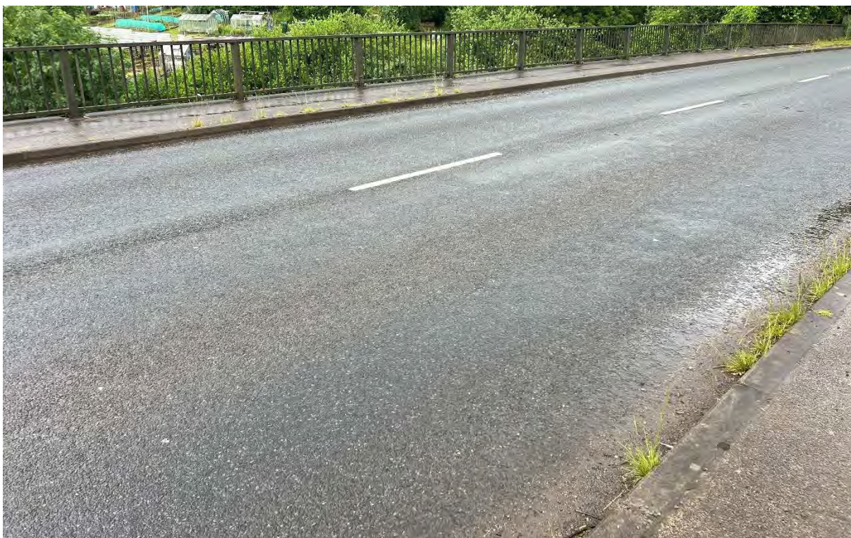
Photograph 82 - Minor vegetation growth to edges of carriageway.
