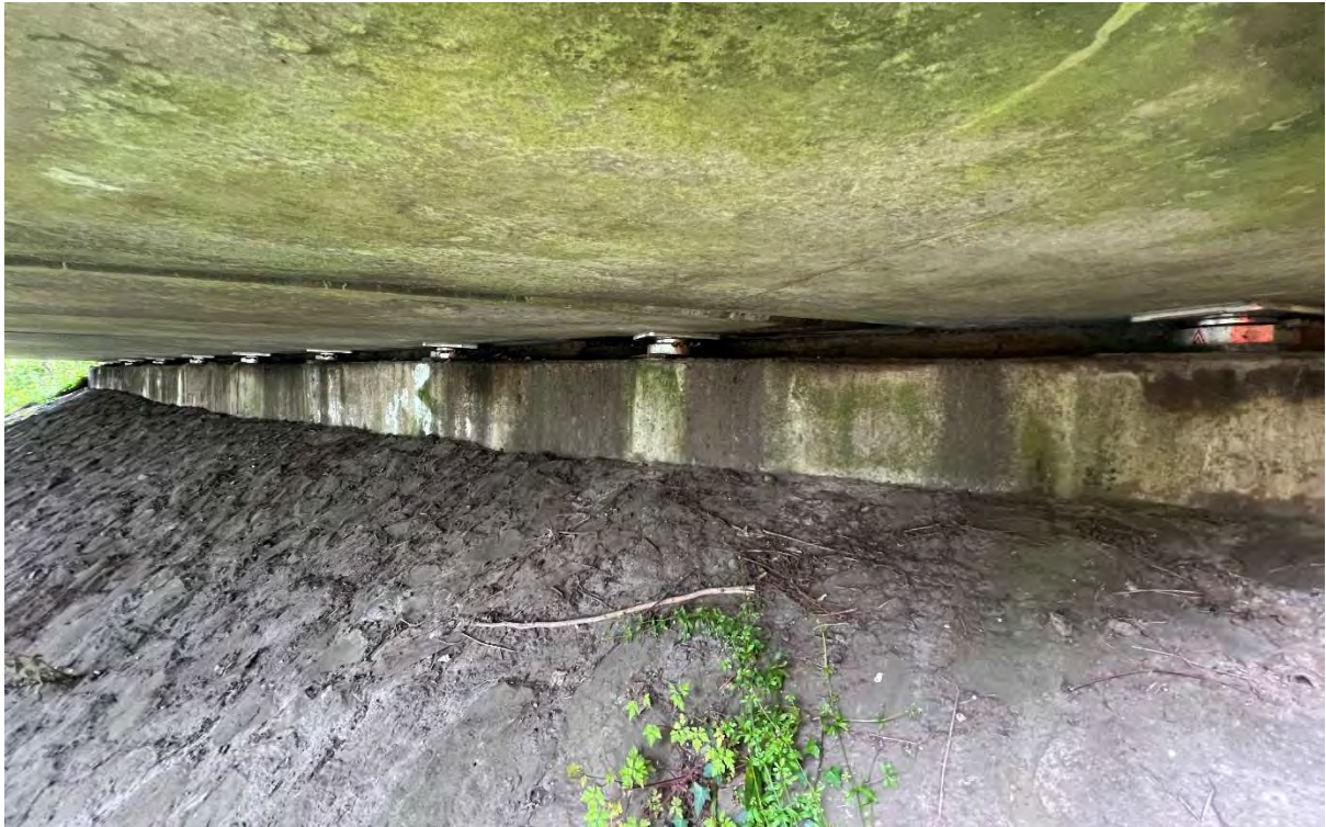
Photograph 63 - Span 1. Historic water seepage & algae staining to south abutment.
