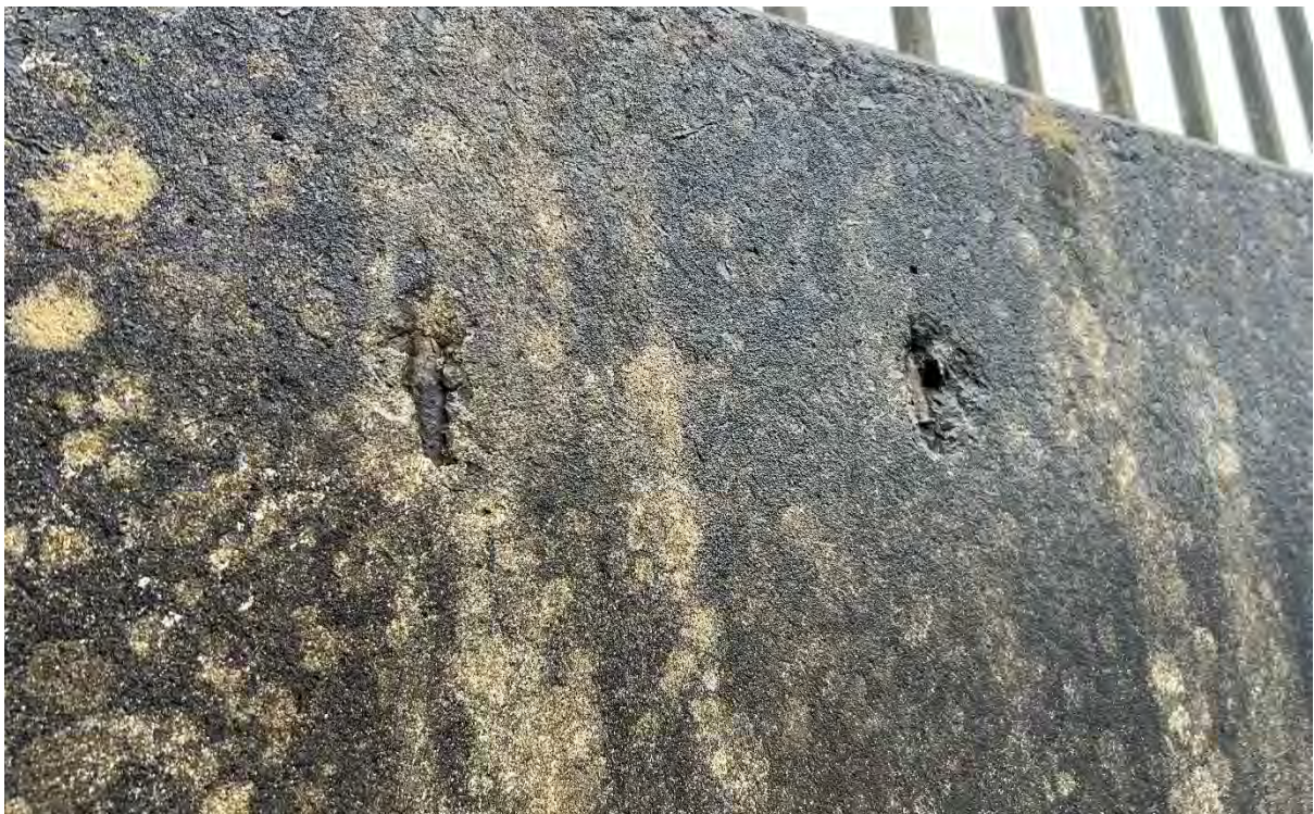
Photograph 52 - Span 1. Multiple minor spalls with exposed reinforcement exhibiting minor corrosion to southeast parapet panels, measuring 100x100x10mm.
