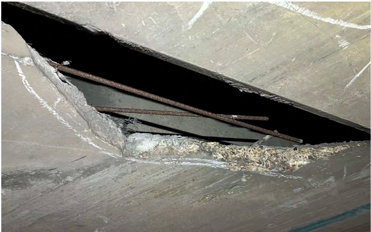
Photograph 36 - Span 2 E/B, beam 5. Area of spalling with exposed reinforcement exhibiting minor corrosion, measuring 800x200x100mm.
