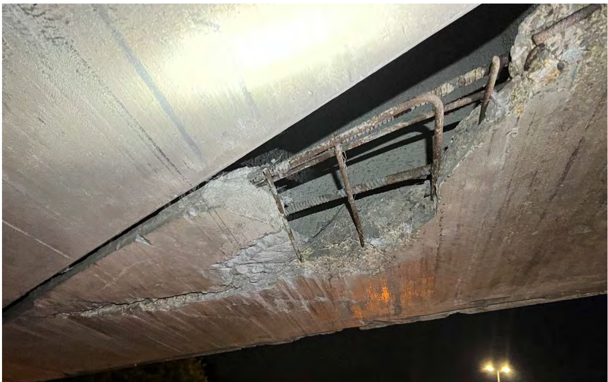
Photograph 46 - Span 2 E/B, beam 9. Area of delamination (2000x500mm) and spalling (1200x550x100mm) with exposed reinforcement exhibiting minor corrosion.
