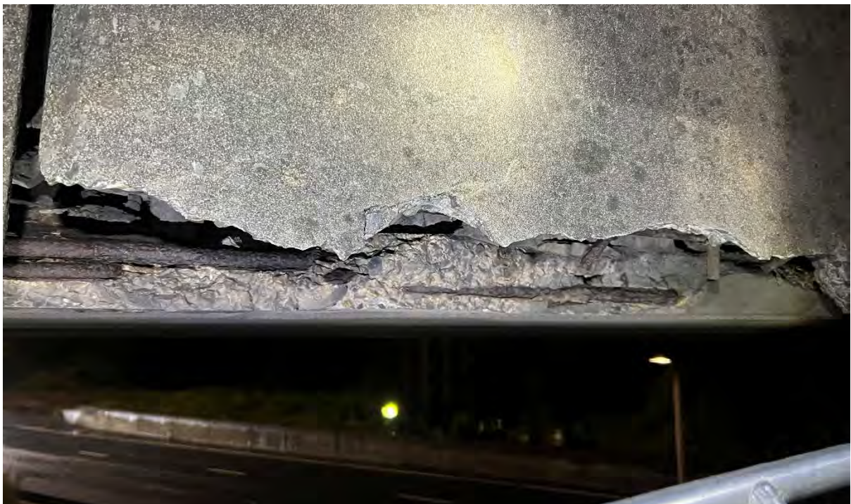
Photograph 54 - Span 2 W/B, east parapet fascia panel. Area of spalling with exposed reinforcement exhibiting minor corrosion, measuring 900x75x75mm.
