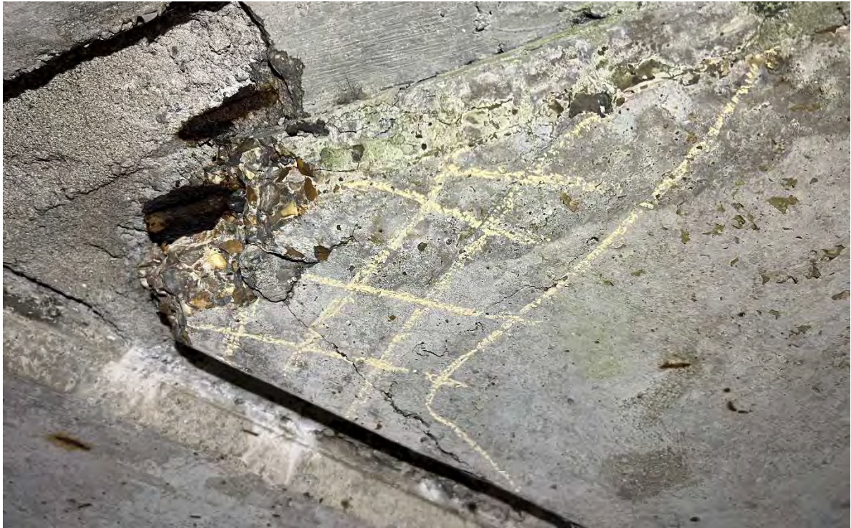
Photograph 25 - Span 2 E/B, beam 1. Area of spalling & delamination with exposed reinforcement exhibiting minor corrosion, measuring 300x200x40mm.
